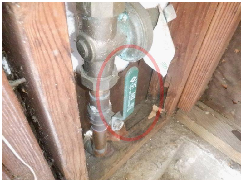
The main water shut off valve
