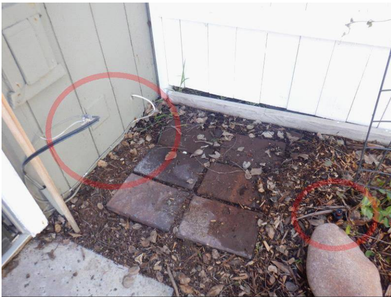
Sprinklers striking wall
