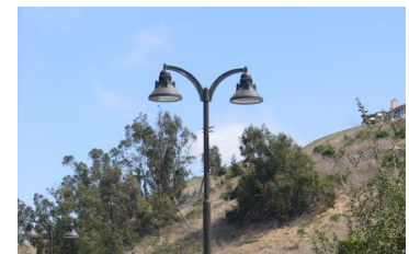
Figure 44. Hooded light fixture directs light downward.
