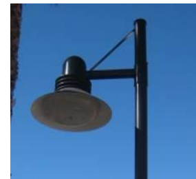
Figure 46. Pole mounted light.
