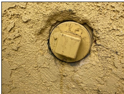
Clean out used for inspection
