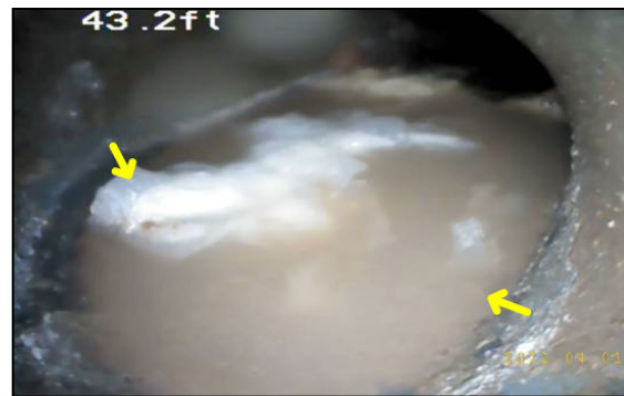
Final Distance/ Standing water/ Debris was present in the sewer line at an approx distance of 43 feet
