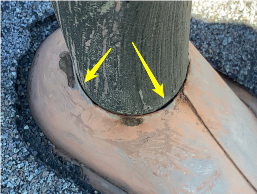
Visible openings and separations
