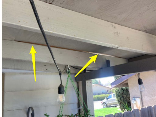
Example. Loose lifting roof plywood
