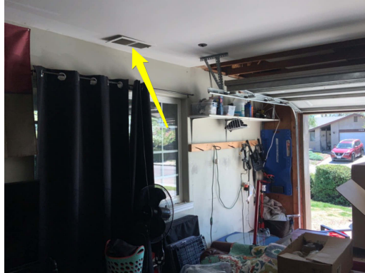
Added Heating register in the garage
