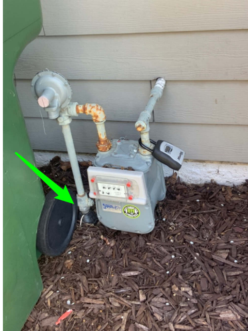
Main shut off valve
