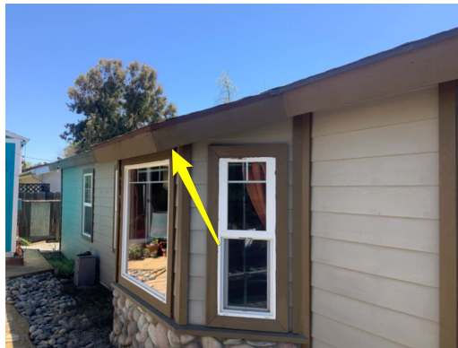
Under the roof overhang, visible moisture staining and damage.
