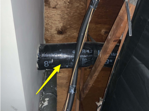
Improper use of non-fire rated flex ducting through the garage firewall
