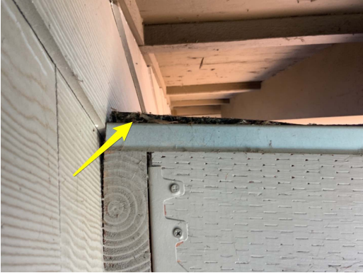
Example. Loose lifting roofing material
