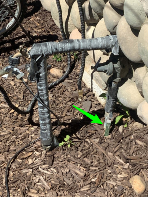
Main water supply shut off valve
