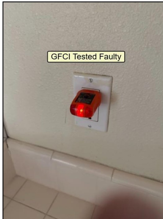
45. Test faulty on GFCI/GFI (Ground Fault...
