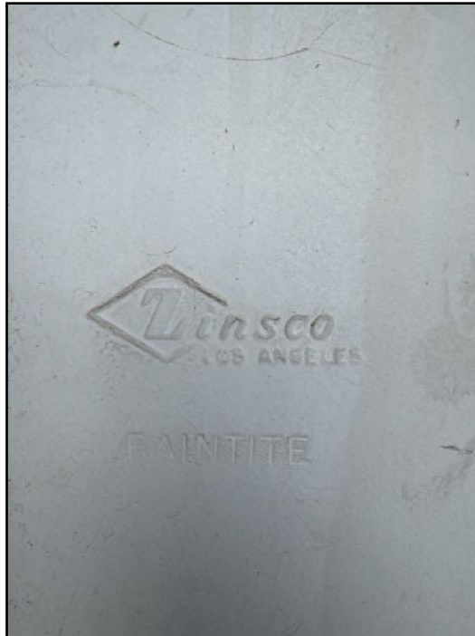
43. Federal Pacific & Zinsco Electrical Panels
