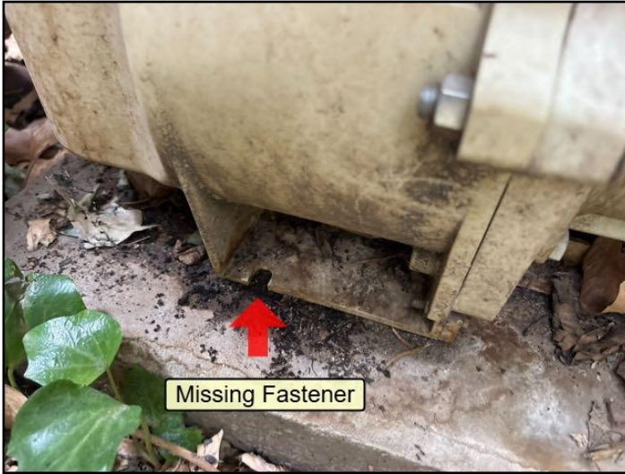
92. Pump has no attachment
