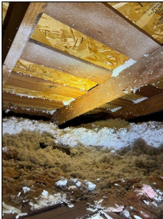
39. Rodent droppings noted in attic.
