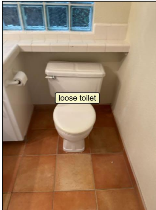
75. Toilet is loose on floor.
