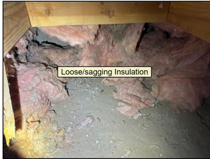
63. Loose, sagging or voids
