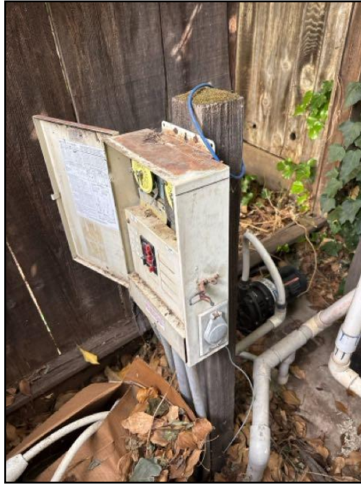
44. Not well secured
