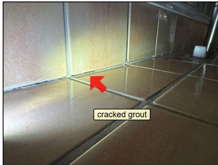
84. Grout loose or missing
