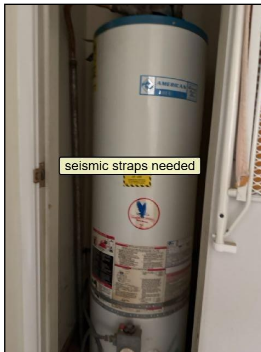
70. Seismic Strapping Needed.
