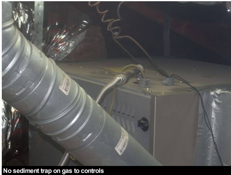
No sediment trap on gas to controls
