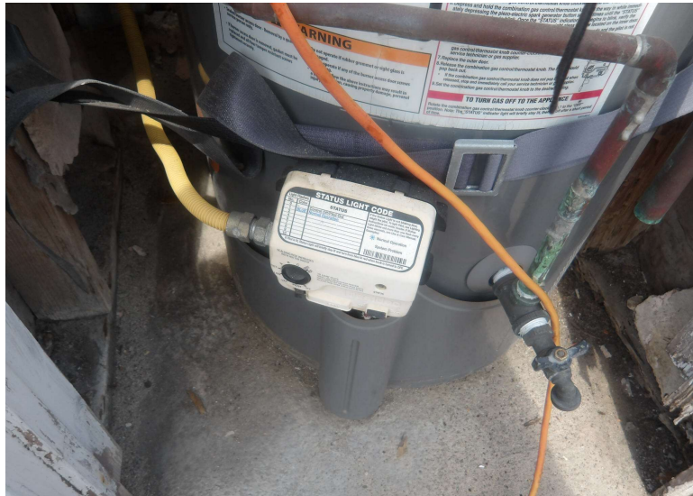
No sediment trap on gas to controls
