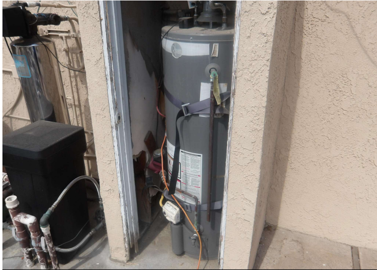
General view of water heater side yard
