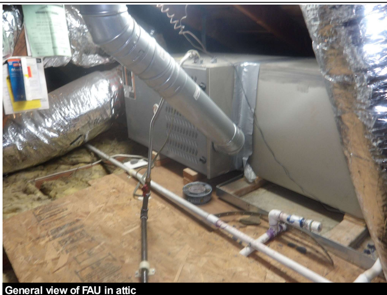
General view of FAU in attic
