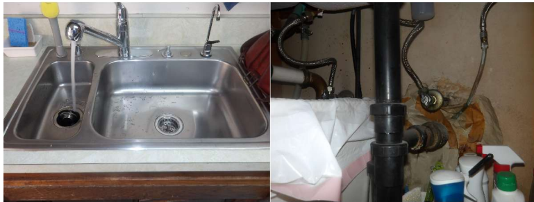
General view of plumbing
