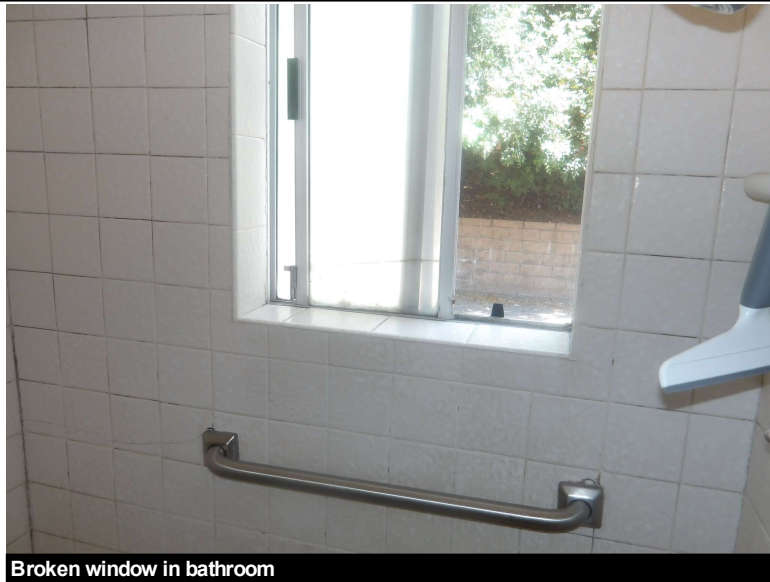
Broken window in bathroom
