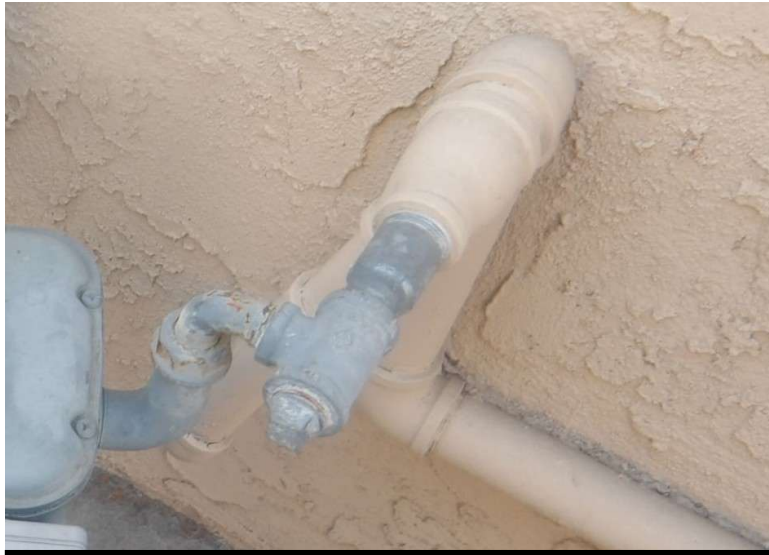
No isolation valve on pool heater gas line
