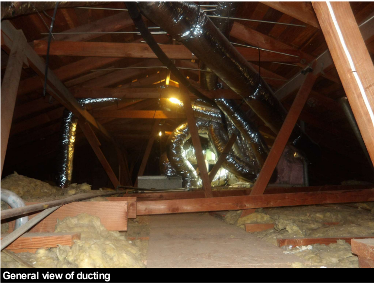
General view of ducting
