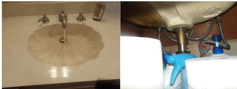
General view of plumbing cabinet
