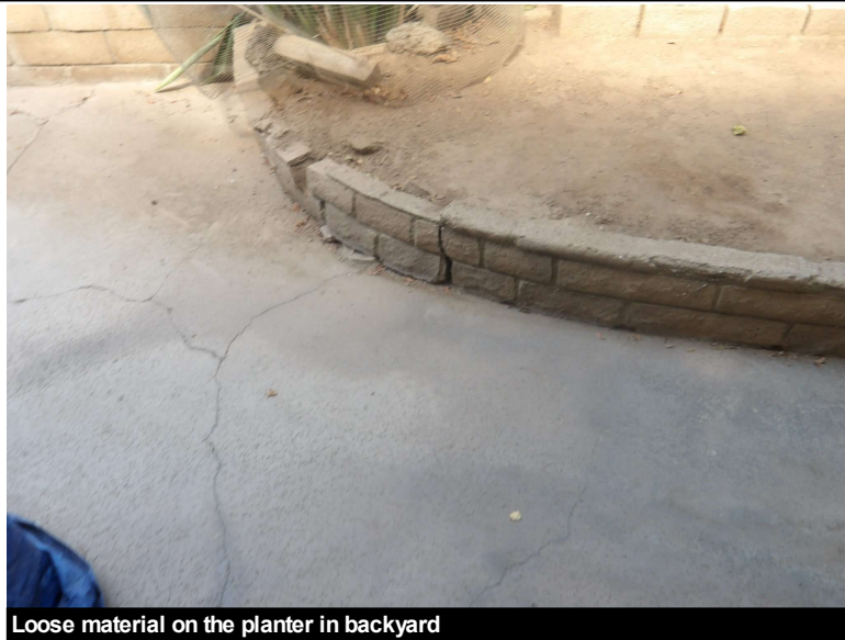
Loose material on the planter in backyard
