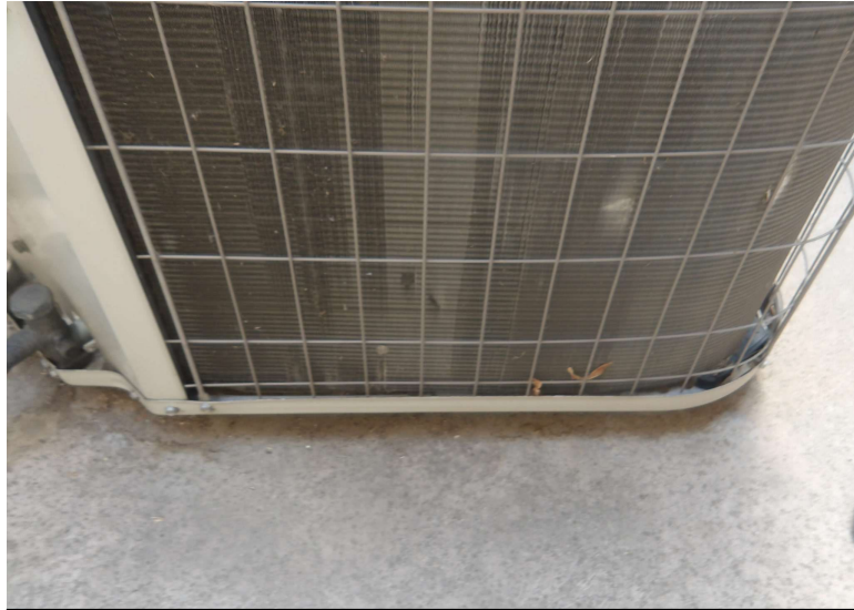
No pad under AC on side yard
