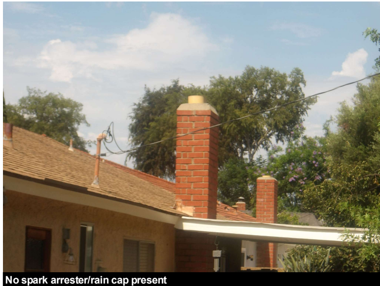
No spark arrester/rain cap present
