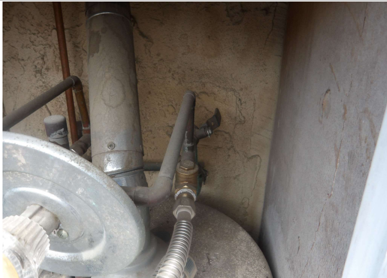
General view of ball valve shut off
