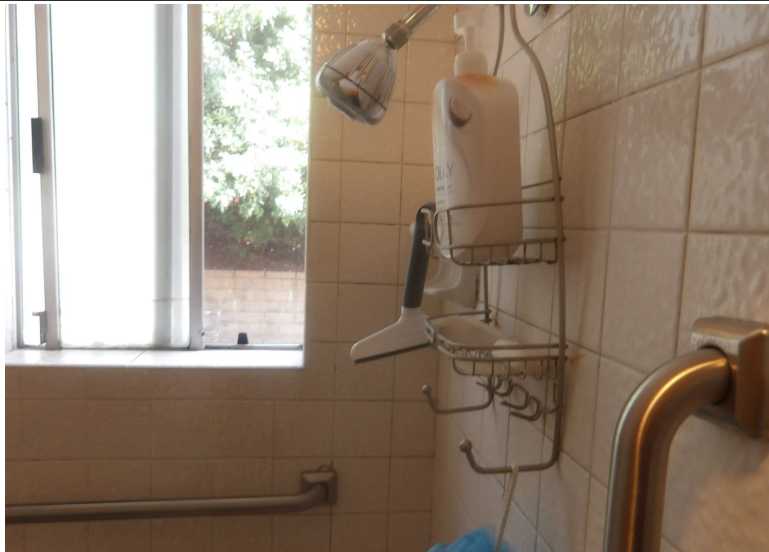
General view of tub plumbing
