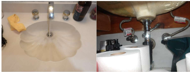
General view of plumbing cabinet
