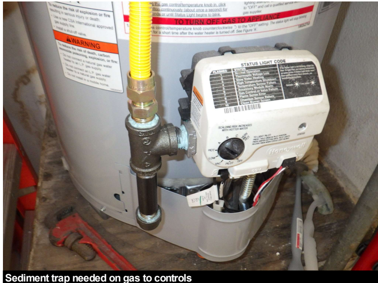
Sediment trap needed on gas to controls
