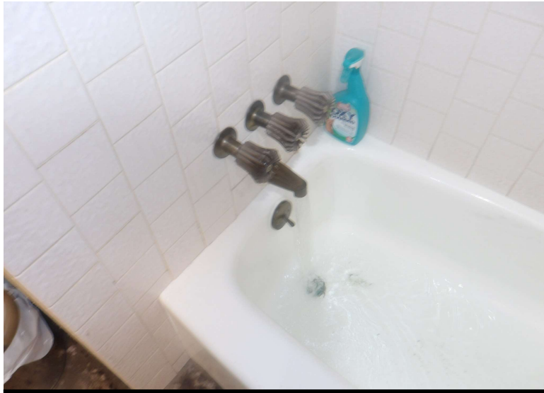
General view of tub plumbing
