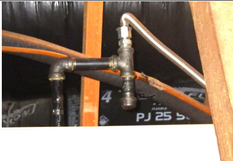
Sediment trap needed on gas to controls
