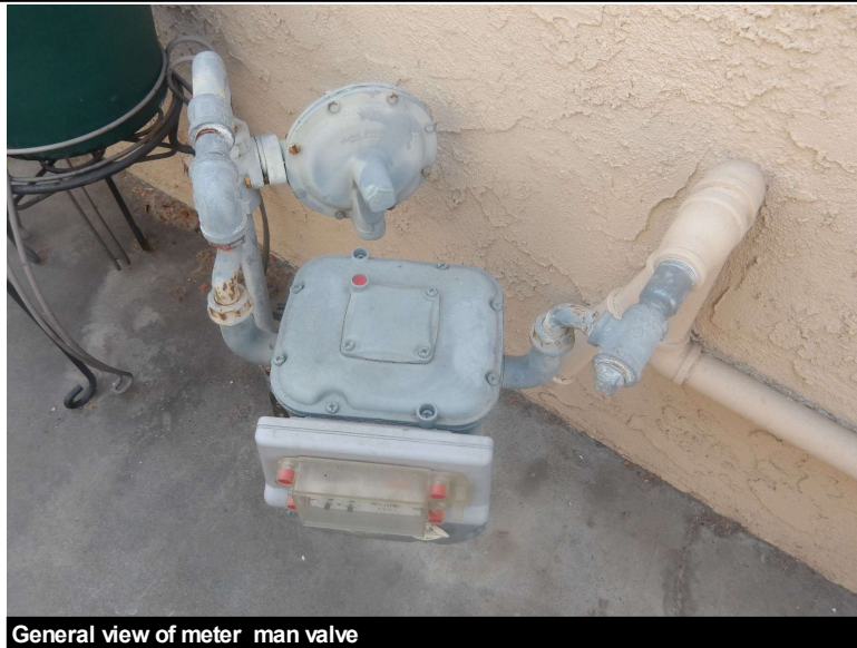
General view of meter man valve
