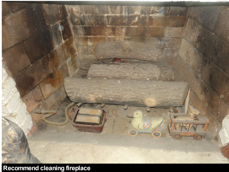
Recommend cleaning fireplace
