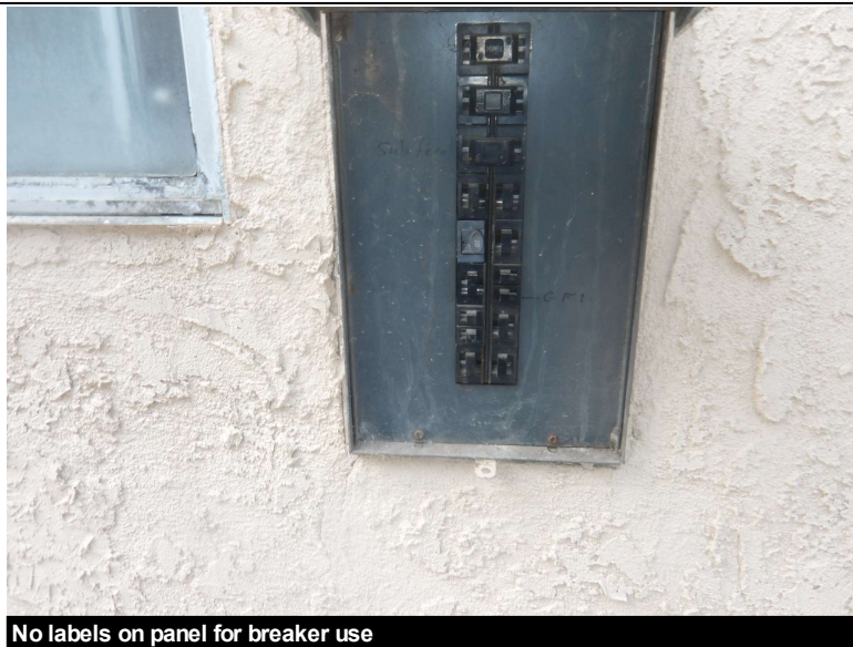
No labels on panel for breaker use
