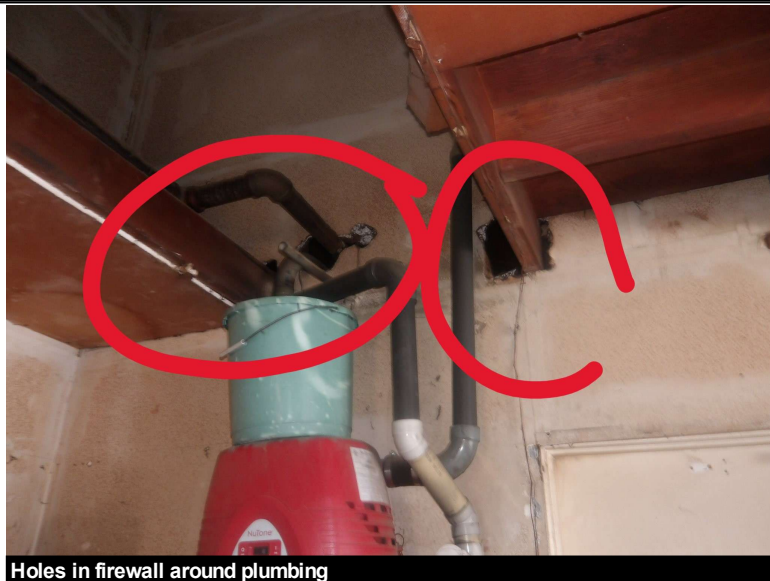
Holes in firewall around plumbing
