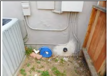
Damaged areas below left side elevation electrical panel boxes
