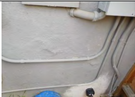
Damaged areas below left side elevation electrical panel boxes
