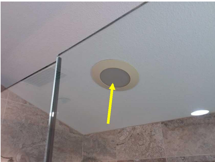
A ceiling light does not respond properly or is flickering and should be serviced.
