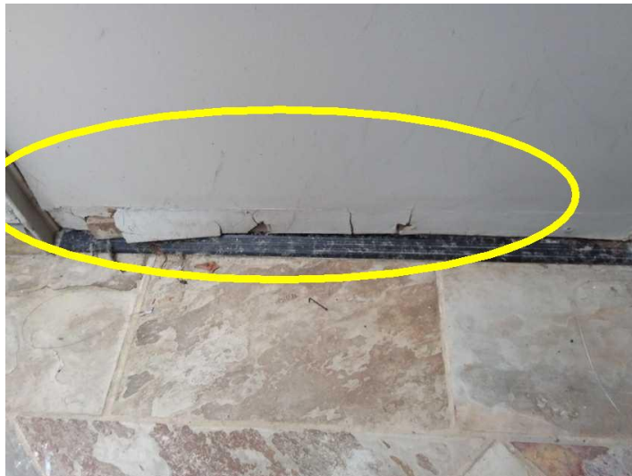
The finish on some of the exterior doors are weathered, and should be refinished or monitored.
