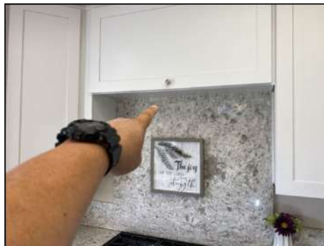
None present - recommend installing an exhaust vent system
