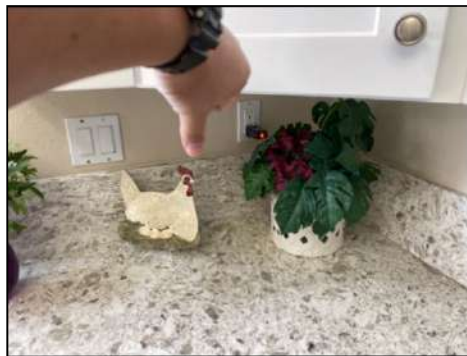
Test did not operate - needs to be serviced
