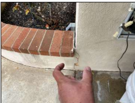
Loose/cracked materials present - needs to be serviced
