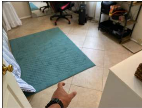
Cracked/loose/missing grout in areas - recommend grout and sealer maintenance
