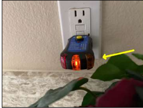
Ungrounded outlets present - consider upgrading electrical services
