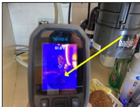
Visible leaking under sink - recommend licensed plumbing contractor for further evaluation and repair
