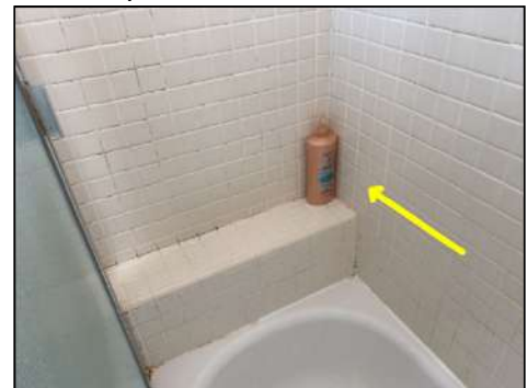
Surface microbial growth/irregular staining is present in areas on nonporous surfaces - recommend cleaning and sealing materials regularly
