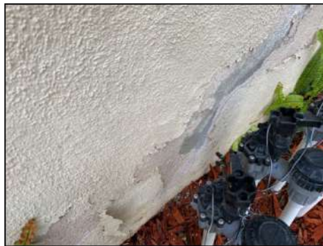
Cracking/chipping/holes more than typical - needs to be serviced
