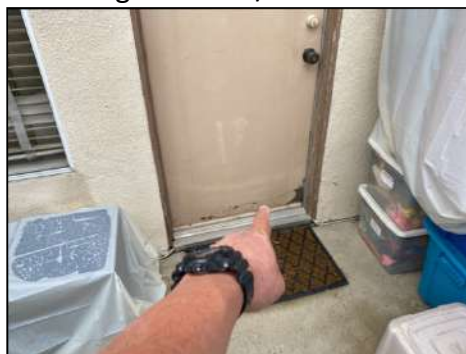
Worn/weathered – recommend weather tight service/ maintenance
