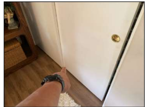
Bypass door guides missing at base - needs to be serviced
