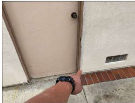
Doors/trim/fascia paint weathered - recommend servicing
