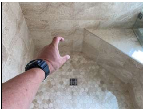
Cracked/loose/missing grout in areas - recommend grout and sealer
