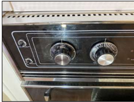
Control knobs not readable - needs to be serviced
