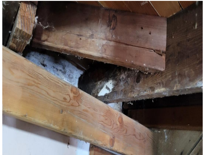
3F - Damaged floor joist.
