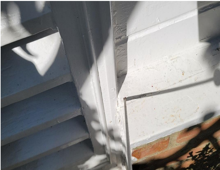
3A - Damaged trim members.
