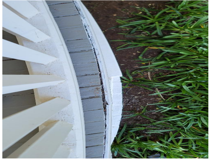
3B - Damaged deck trim.
