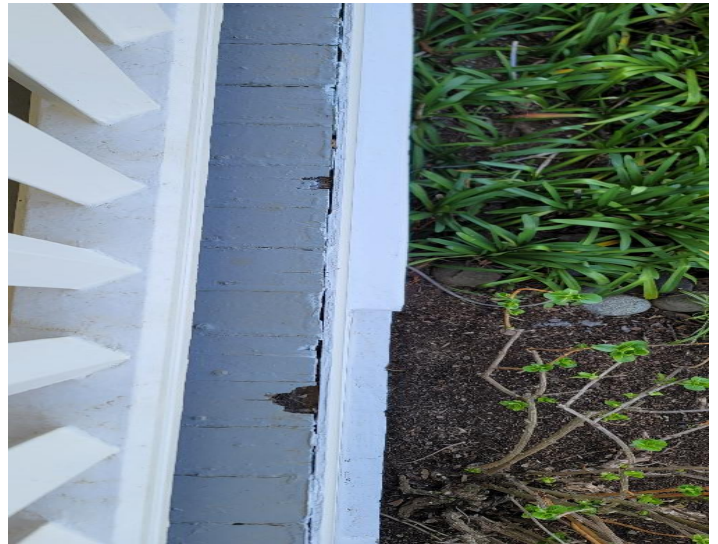
3B - Damaged decking.
