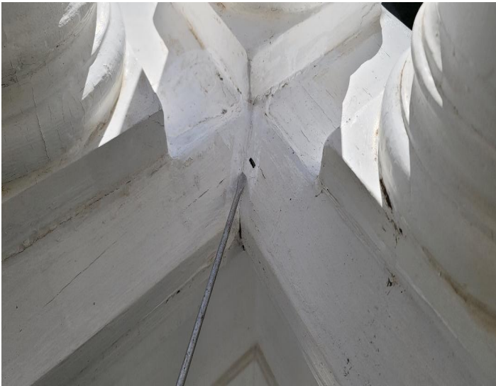
3A - Damaged trim members.
