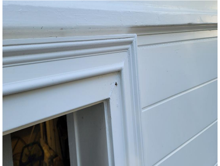
3D - Damaged door jambs.
