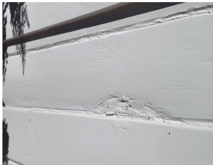
3G - Damaged siding.
