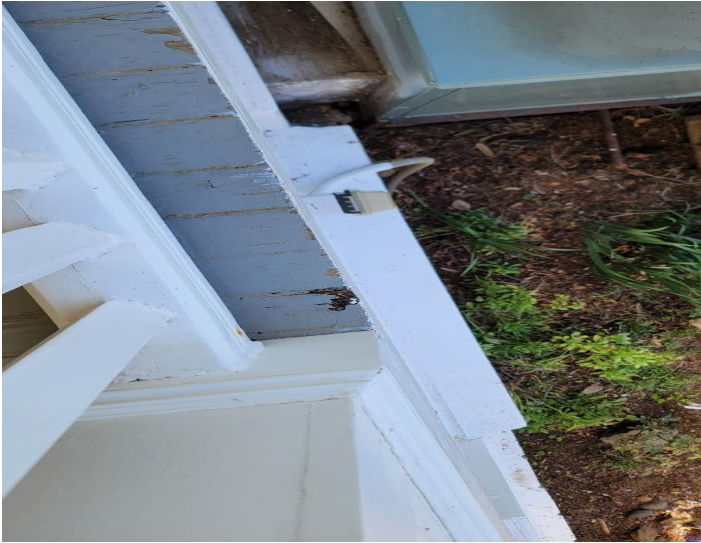
3B - Damaged decking.
