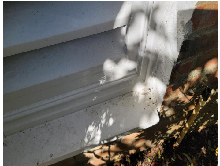
3A - Damaged trim members.
