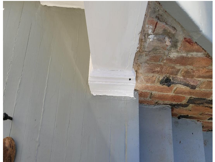
3A - Damaged trim members.
