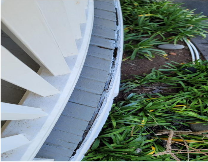
3B - Damaged deck trim.
