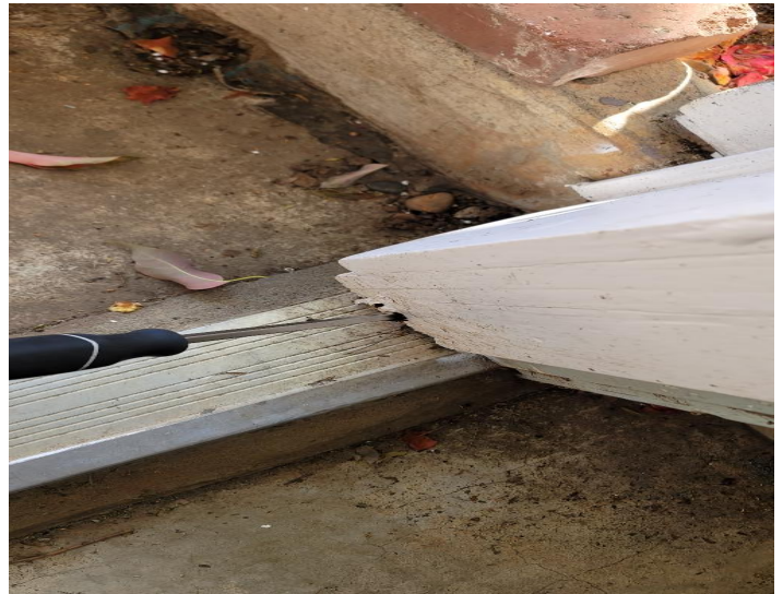
3D - Damaged door jambs.
