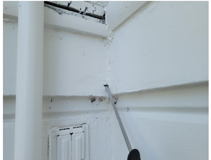
3A - Damaged trim members.
