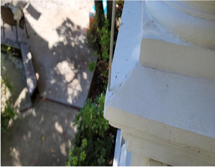
3A - Damaged trim members.
