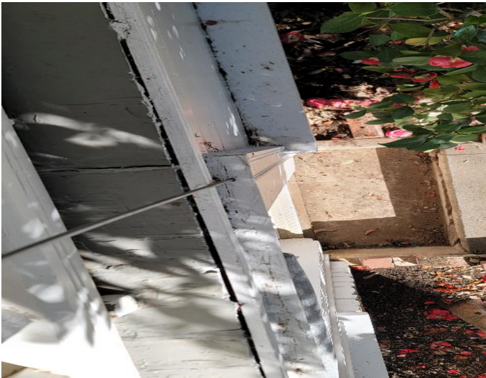
3A - Damaged trim members.
