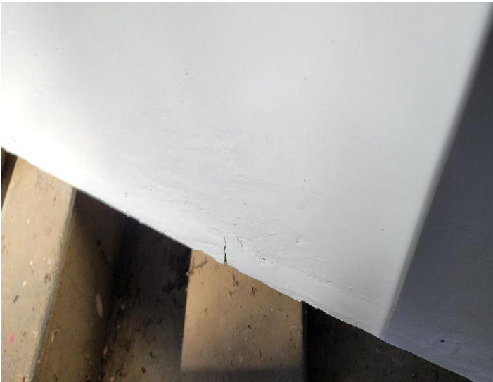
3E - Damaged basement door.
