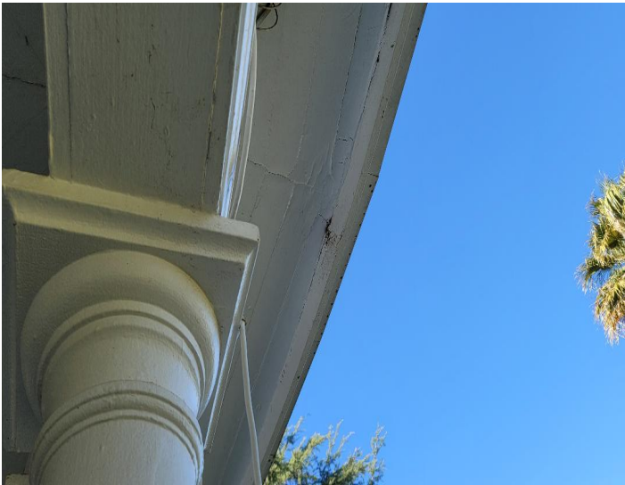
3C - Damaged roof soffit.
