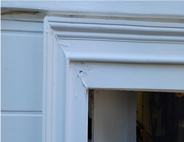
3D - Damaged door jambs.
