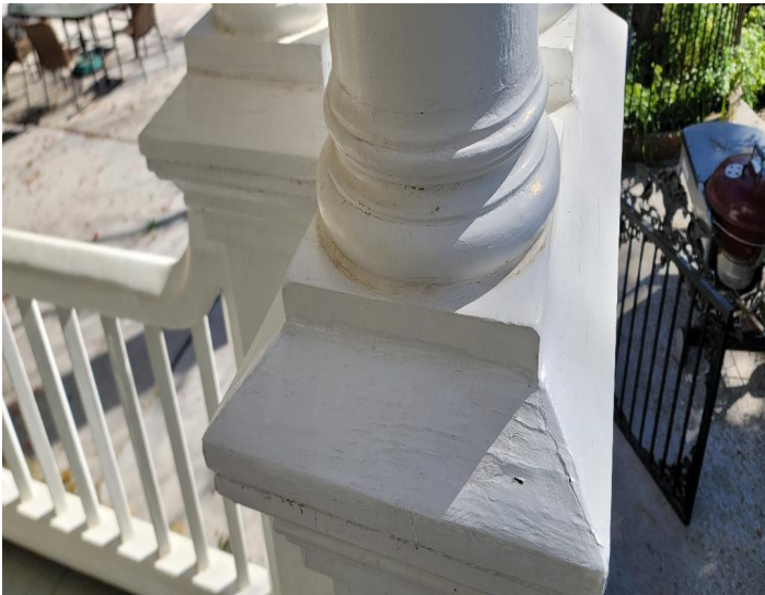
3A - Damaged trim members.
