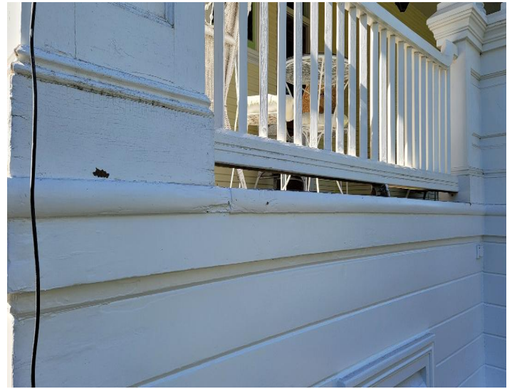
3A - Damaged trim members.
