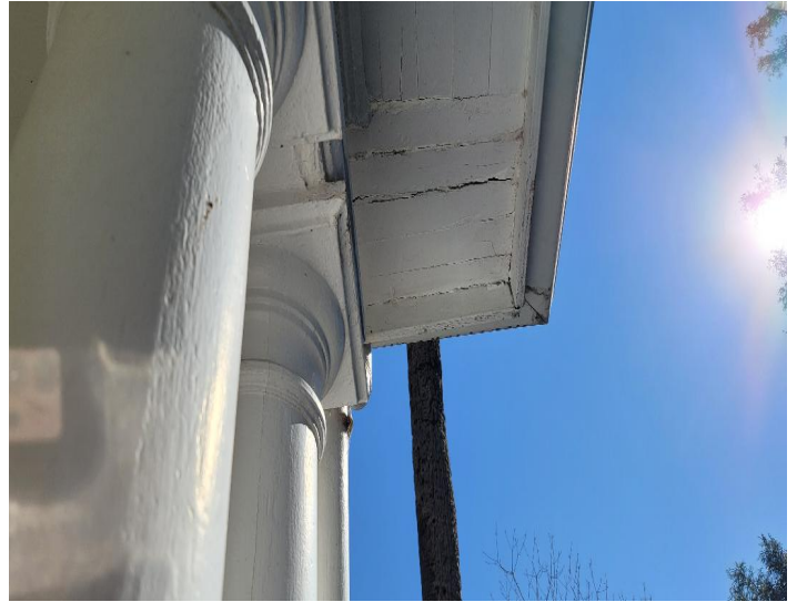
3C - Damaged roof soffit.
