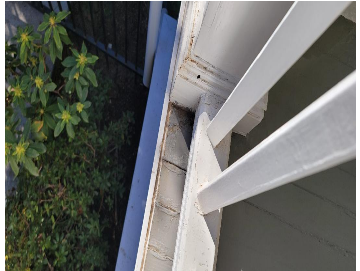
3A - Damaged trim members.
