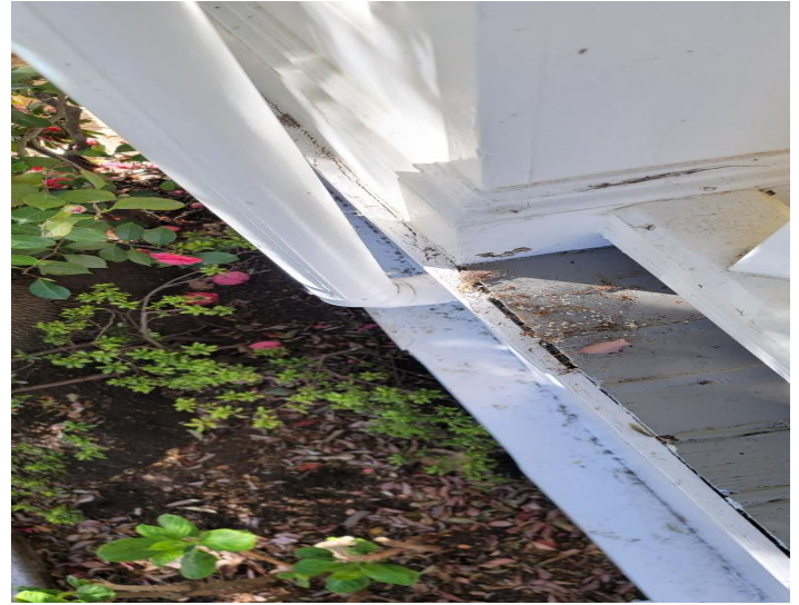
3A - Damaged trim members.
