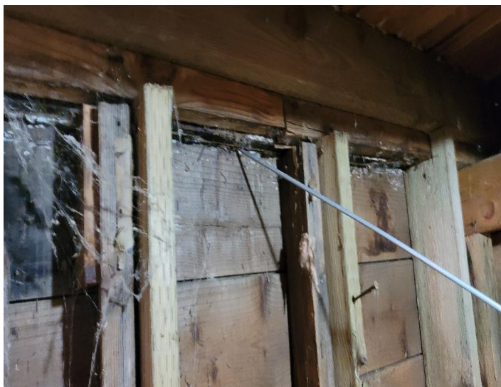
3F - Damaged framing plate.
