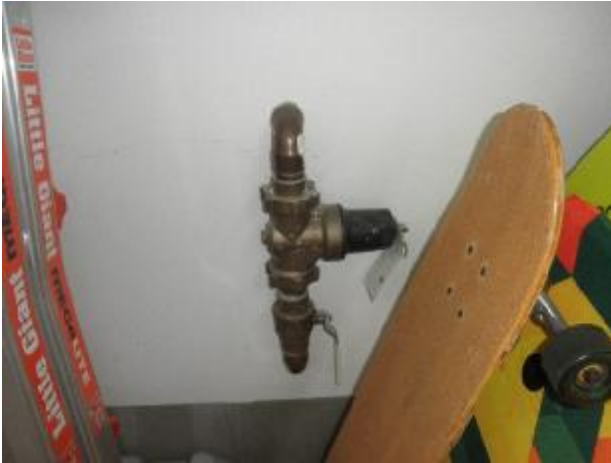
The main water shut off is located at the interior SW wall of the garage.
