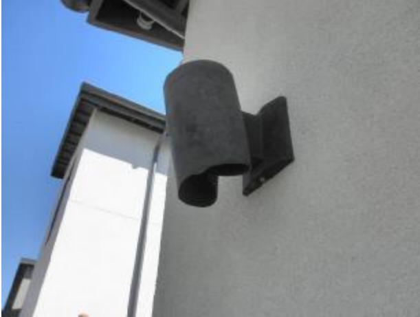
Damaged light fixture at the front of the garage.
