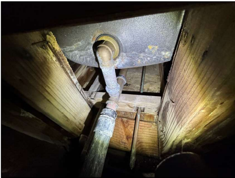
Leak found under tub – service recommended
