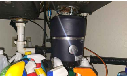
Dishwasher: Unit Was working properly at time of inspection? yes
