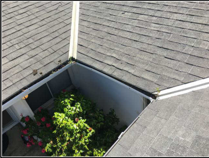
View of dirty gutters.
