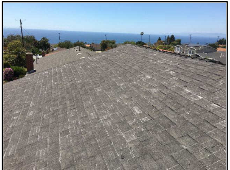
View of worn roof/loosing granules.
