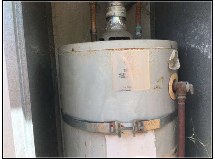
View of water heater. Unit has exceeded its life expectancy. Corroded plumbing. Rusty TP Valve/Overflow pipe.
