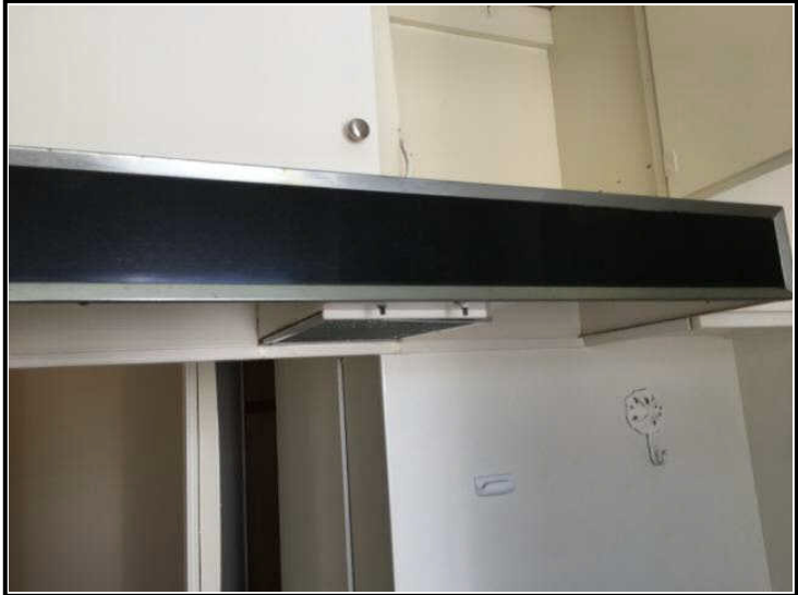
View of stove hood. Oil cleaning advisable.
