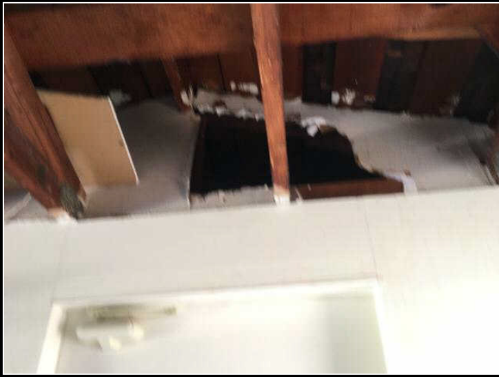
View of repairs advisable at fire wall.
