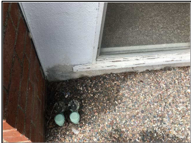
View of sprinkler valves.
