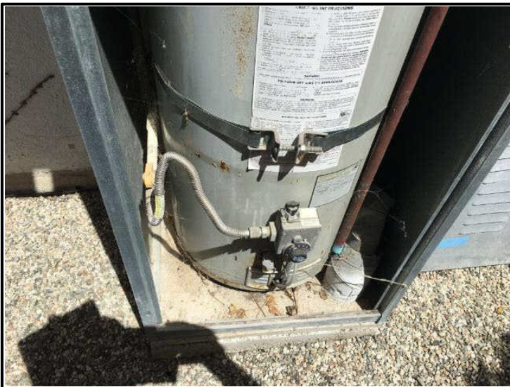
View of water heater, corrosion at plumbing.
