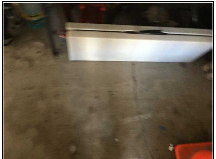
View of cracks at slab.
