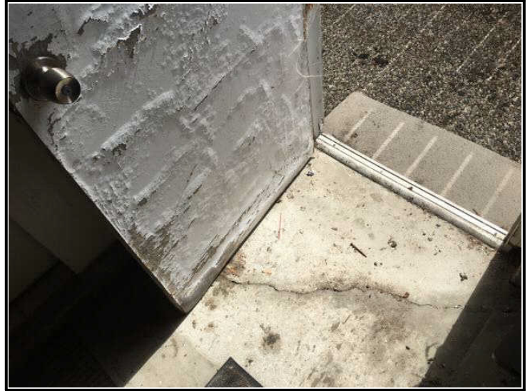
View of weatherized, water damaged access door.
