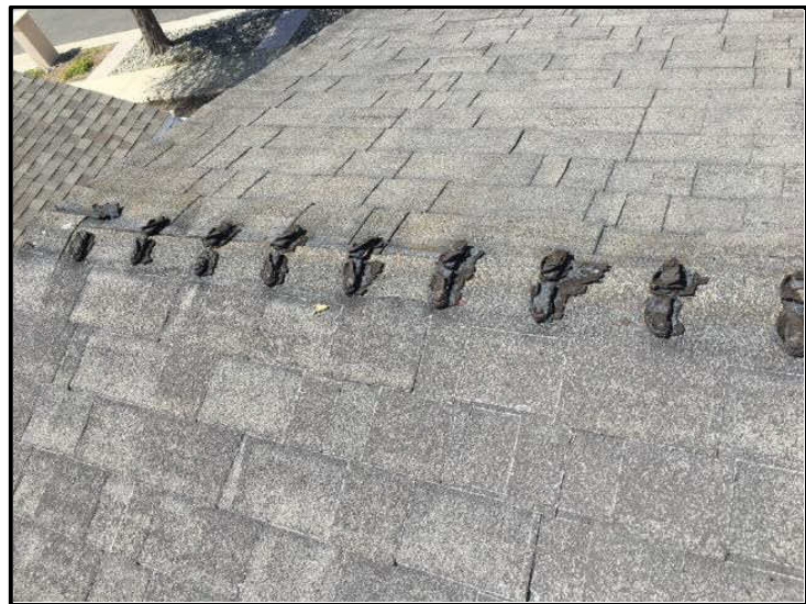
View of worn/missing caps, worn roof/loosing granules.
