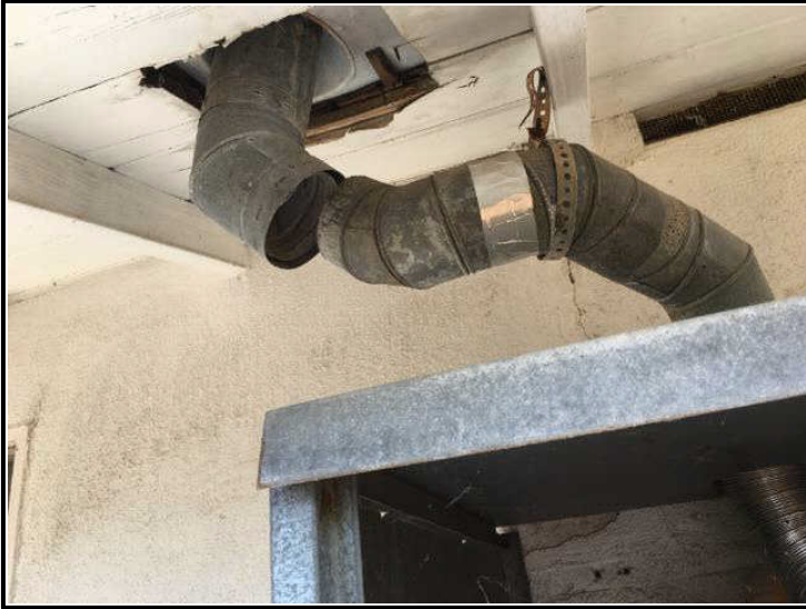
View of water heater ventilation pipe not properly installed.
