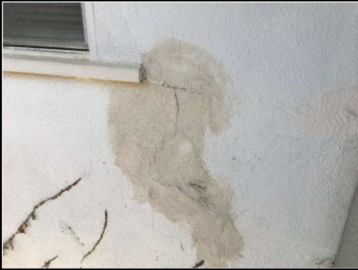
View of stucco cracks.
