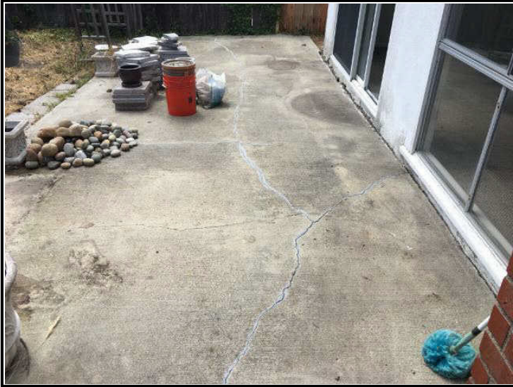
View of cracked patio slab.
