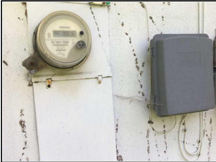
View of electric meter.
