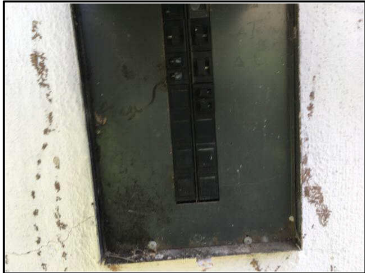
View of electric panel. Advisable to label all breakers.
