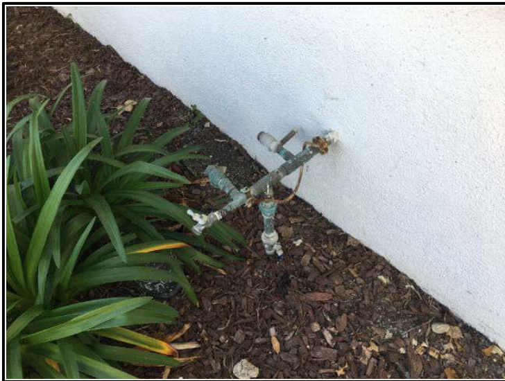
View of water service. Water shut-off buried in soil.
