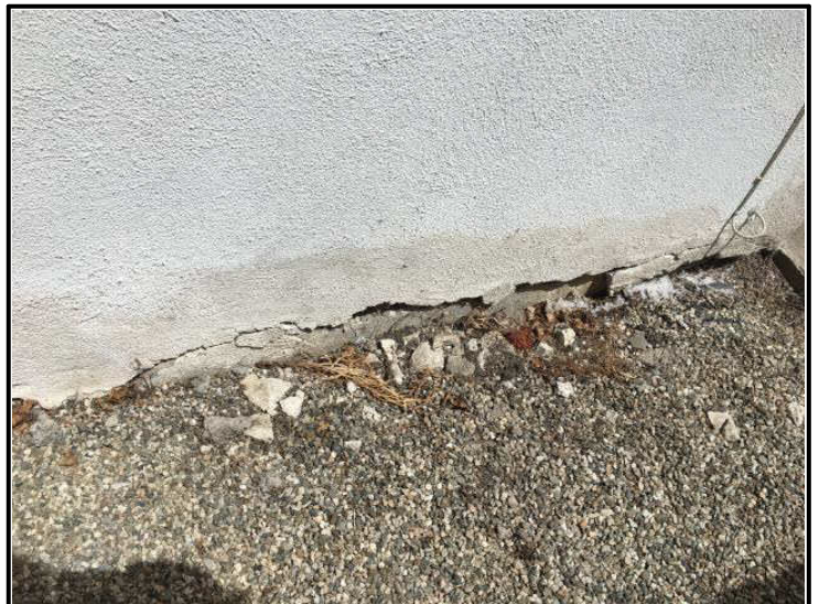
View of stucco cracks at foundation line.
