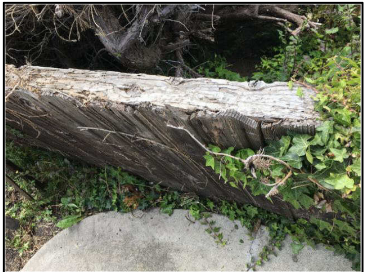
View of damaged, dry rotted wood fence.
