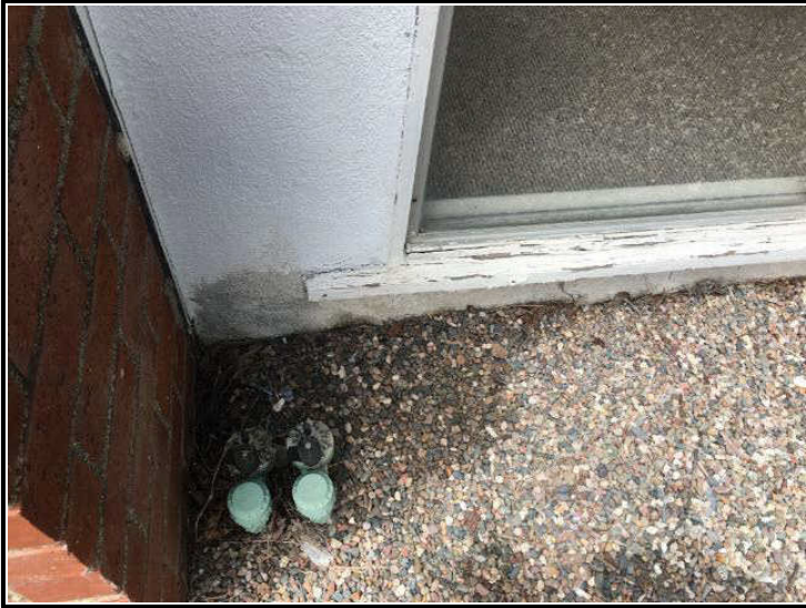
View of moisture at perimeter of the foundation wall.
