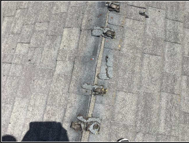
View of worn/missing caps, worn roof/loosing granules.
