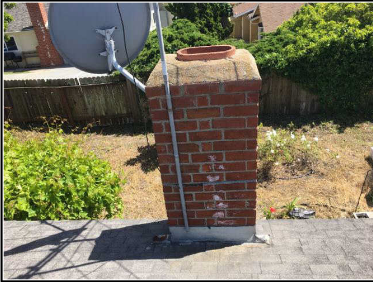
View of chimney missing cap.
