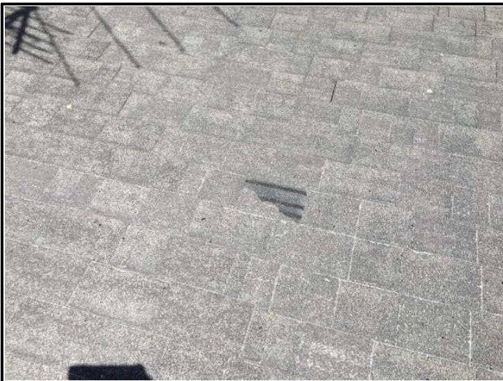
View of worn roof/loosing granules, missing shingles.
