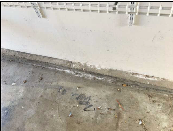
View of cracks at perimeter of foundation.
