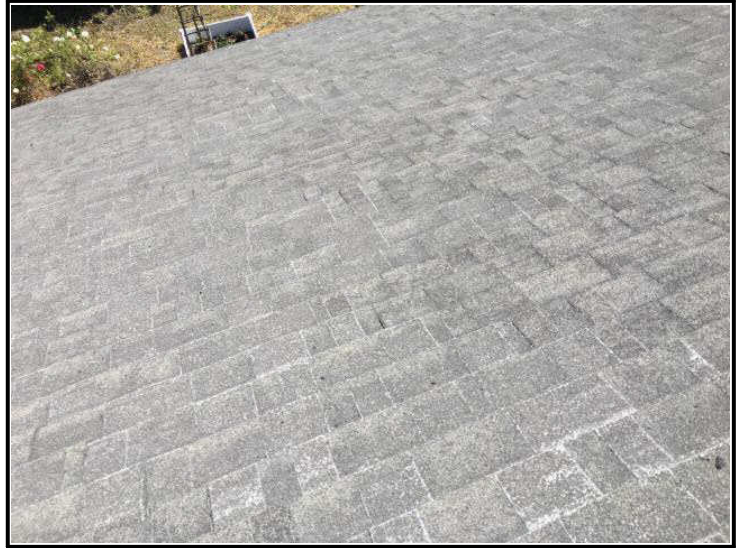
View of worn roof/loosing granules.
