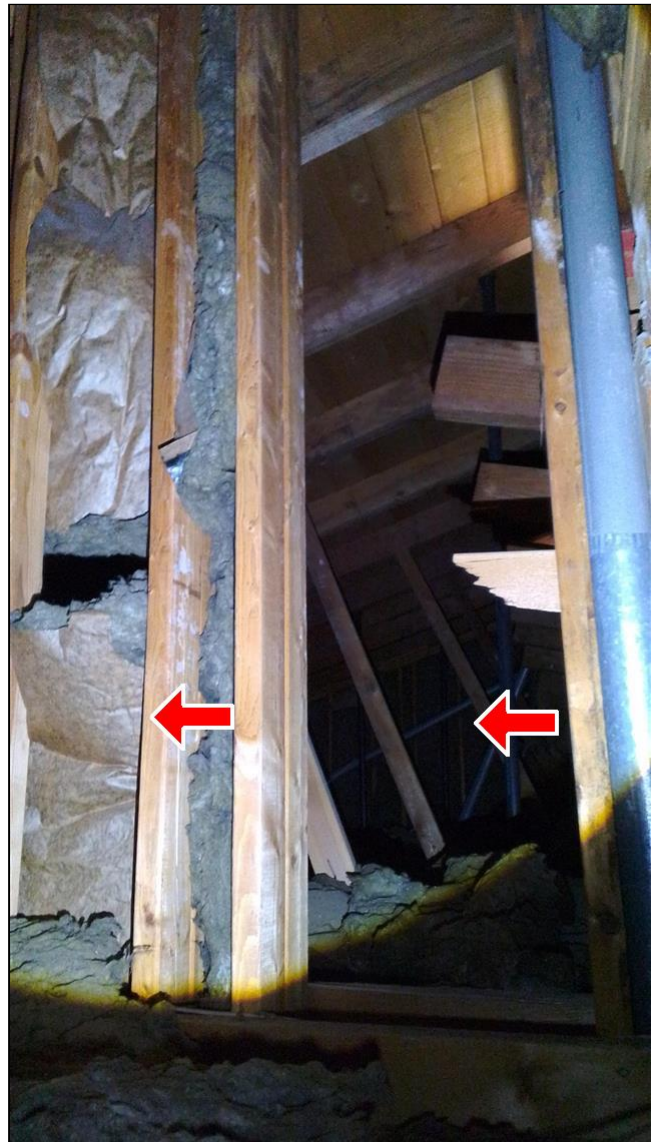
2.4 Item 1(Picture) Missing firewall separation, attic
