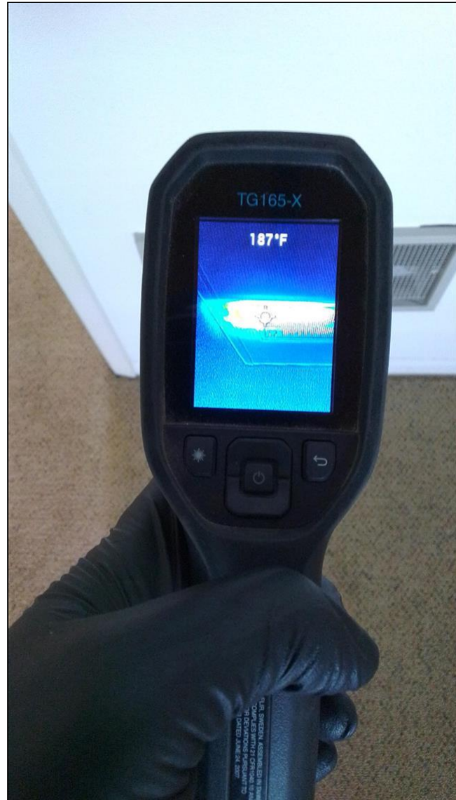
9.1 Item 2(Picture) Electric wall heater #2 temperature
