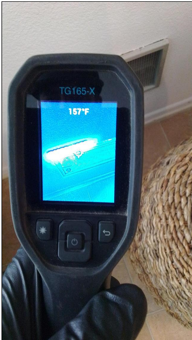
9.1 Item 3(Picture) Electric wall heater #3 temperature
