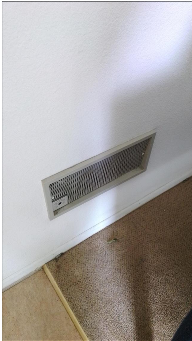
9.0 Item 5(Picture) Electric wall heater #5, living room
