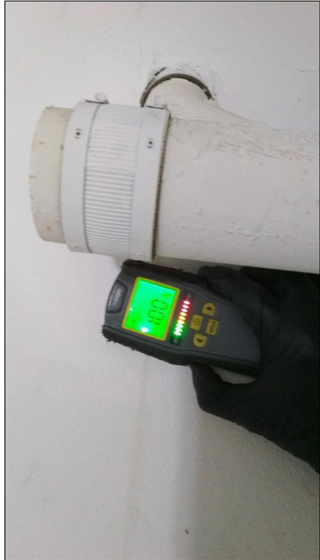
3.2 Item 4(Picture) Elevated moisture levels
