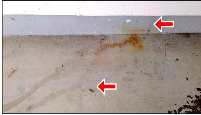
6.5 Item 6(Picture) Active leaking, garage, south wall
