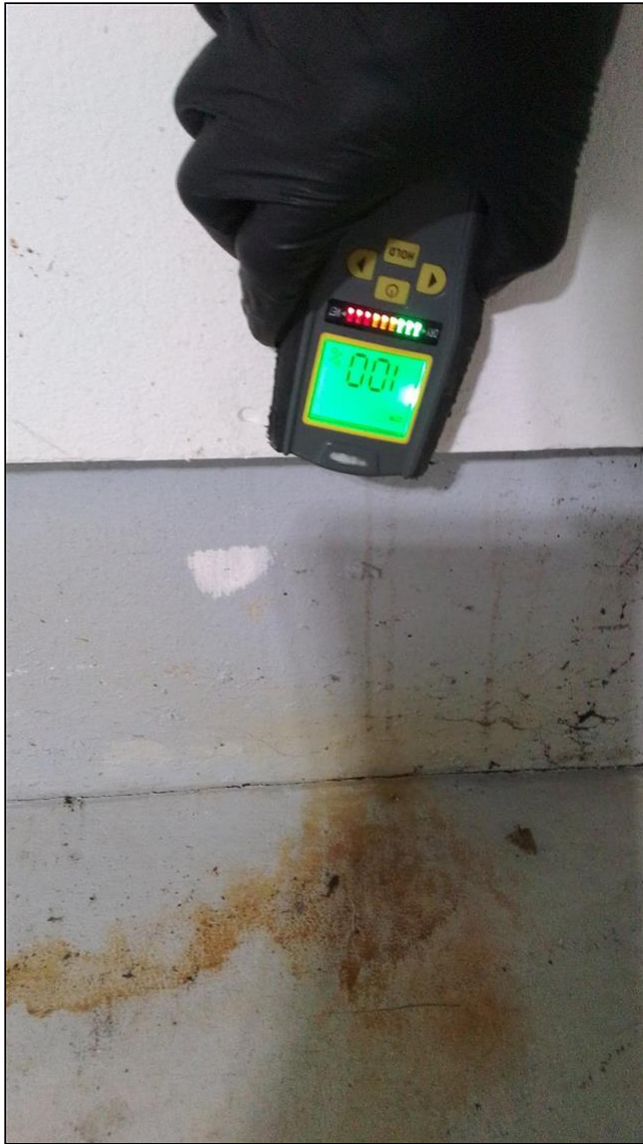
3.2 Item 3(Picture) Elevated moisture levels
