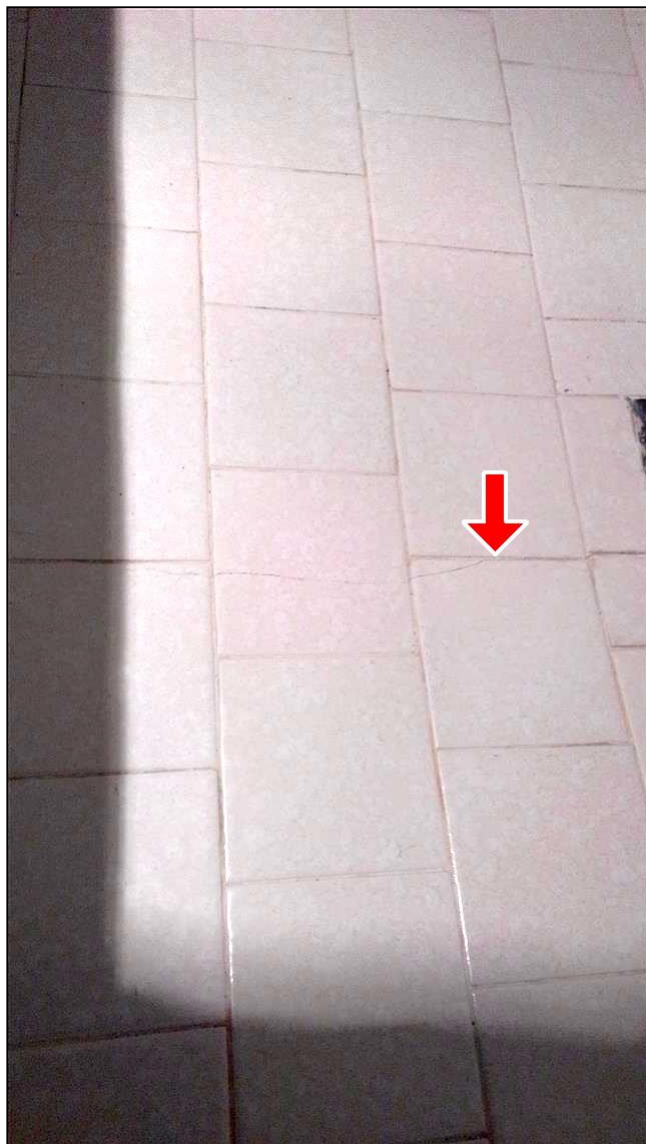
4.3 Item 1(Picture) Minor crack, primary bed bath shower
