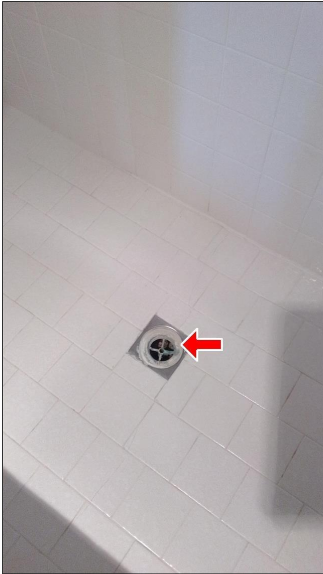
6.5 Item 1(Picture) Missing drain stop, primary bed bath
