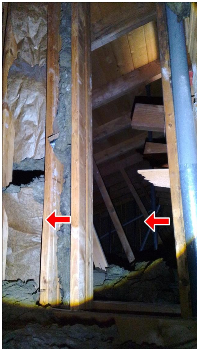
2.4 Item 1(Picture) Missing firewall separation, attic
