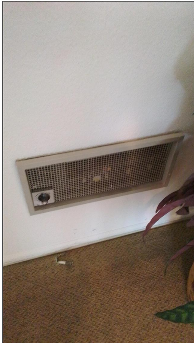
9.0 Item 4(Picture) Electric wall heater #4, dining area
