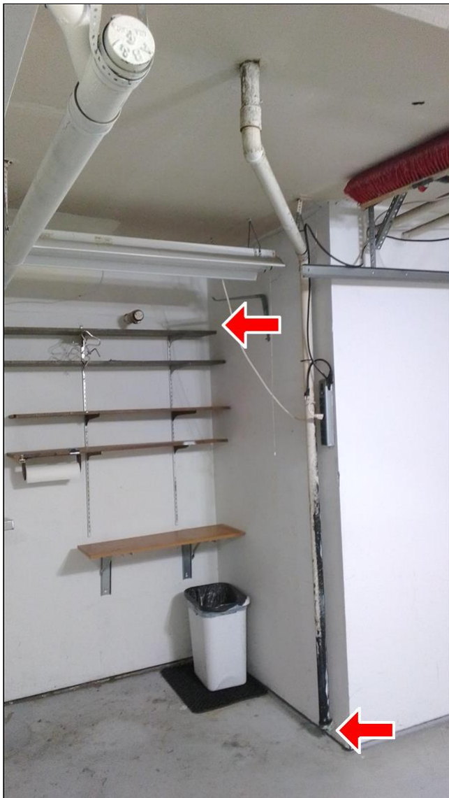
6.5 Item 7(Picture) Washer drip pan drain line, garage
