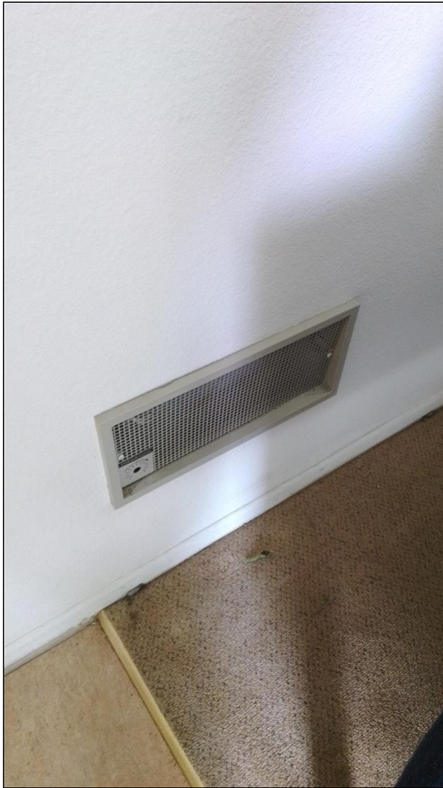
9.0 Item 5(Picture) Electric wall heater #5, living room
