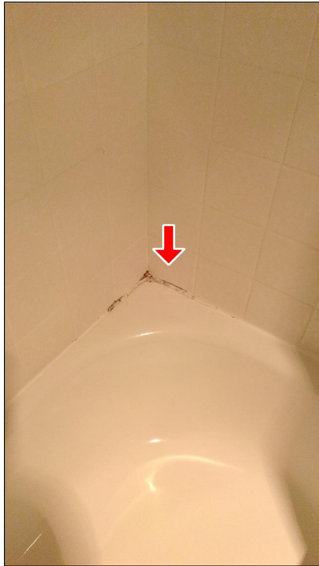
4.3 Item 3(Picture) Cracked and deteriorated seal, 2nd floor hall bathroom
