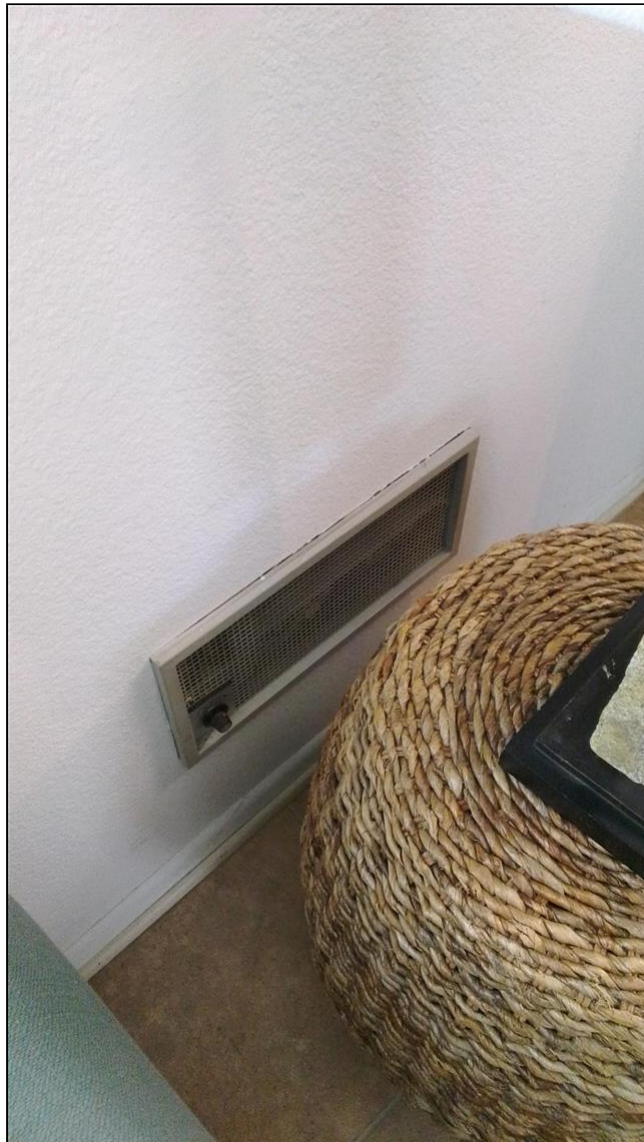
9.0 Item 3(Picture) Electric wall heater #3, kitchen area
