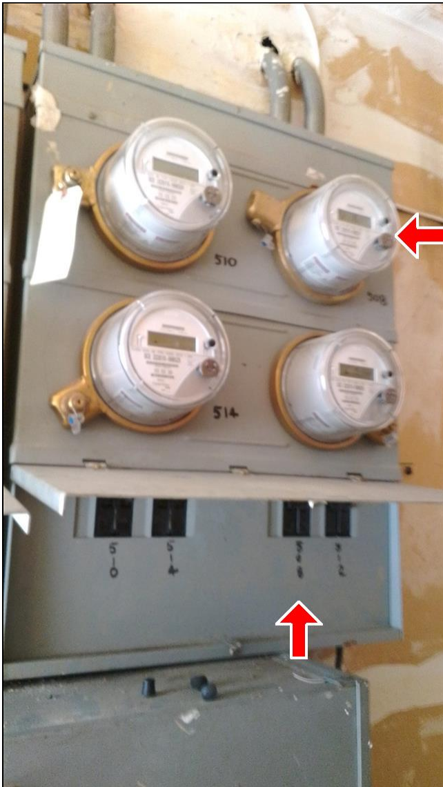
5.1 Item 1(Picture) Electric meter and main shut off
