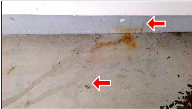
6.5 Item 6(Picture) Active leaking, garage, south wall
