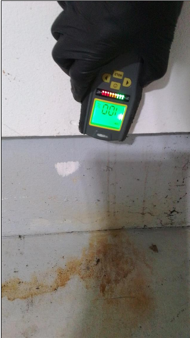
3.2 Item 3(Picture) Elevated moisture levels
