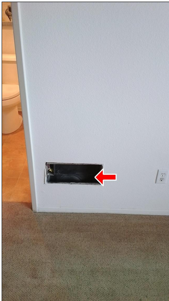
9.0 Item 6(Picture) Wall heater missing, primary bedroom
