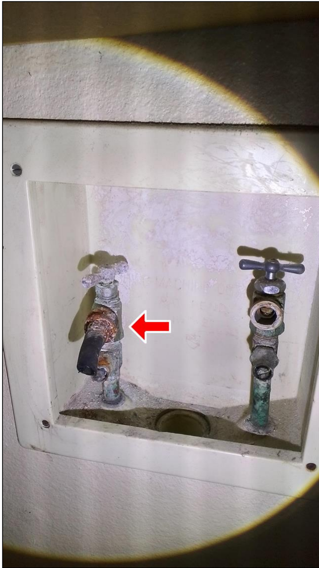
6.3 Item 3(Picture) Washer water supply, laundry closet
