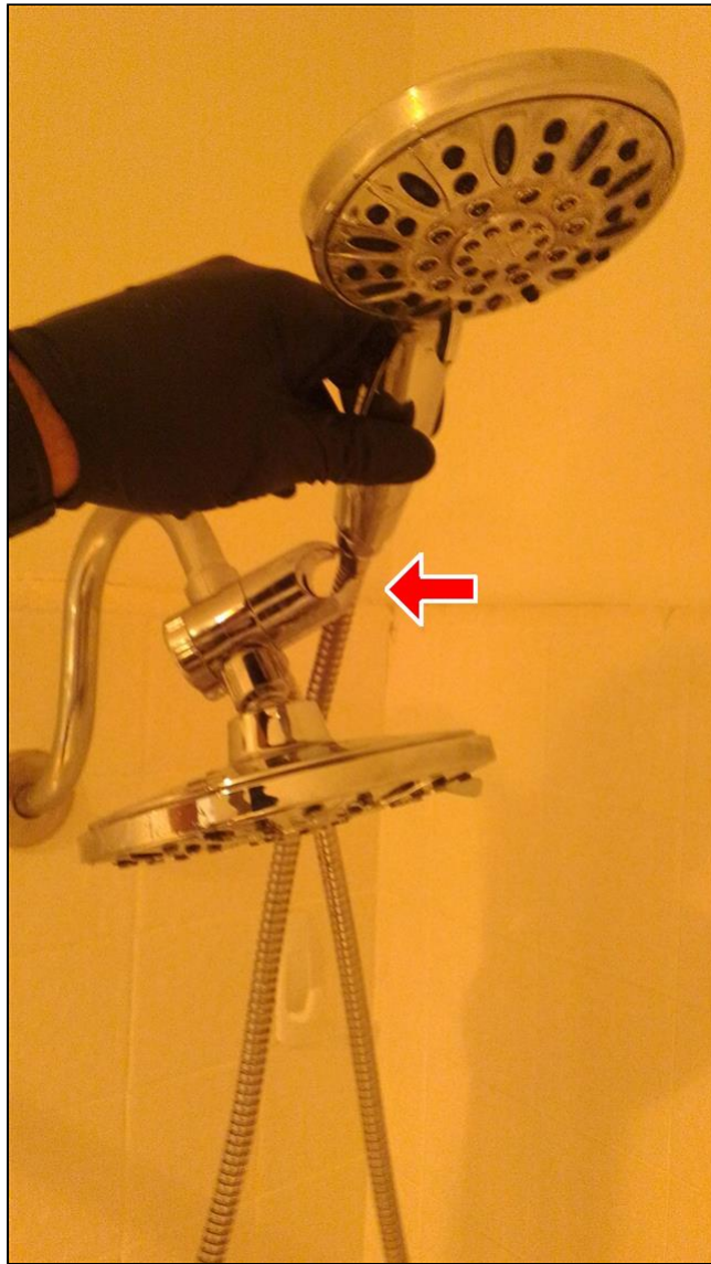
6.3 Item 2(Picture) 2nd floor hall bath shower head
