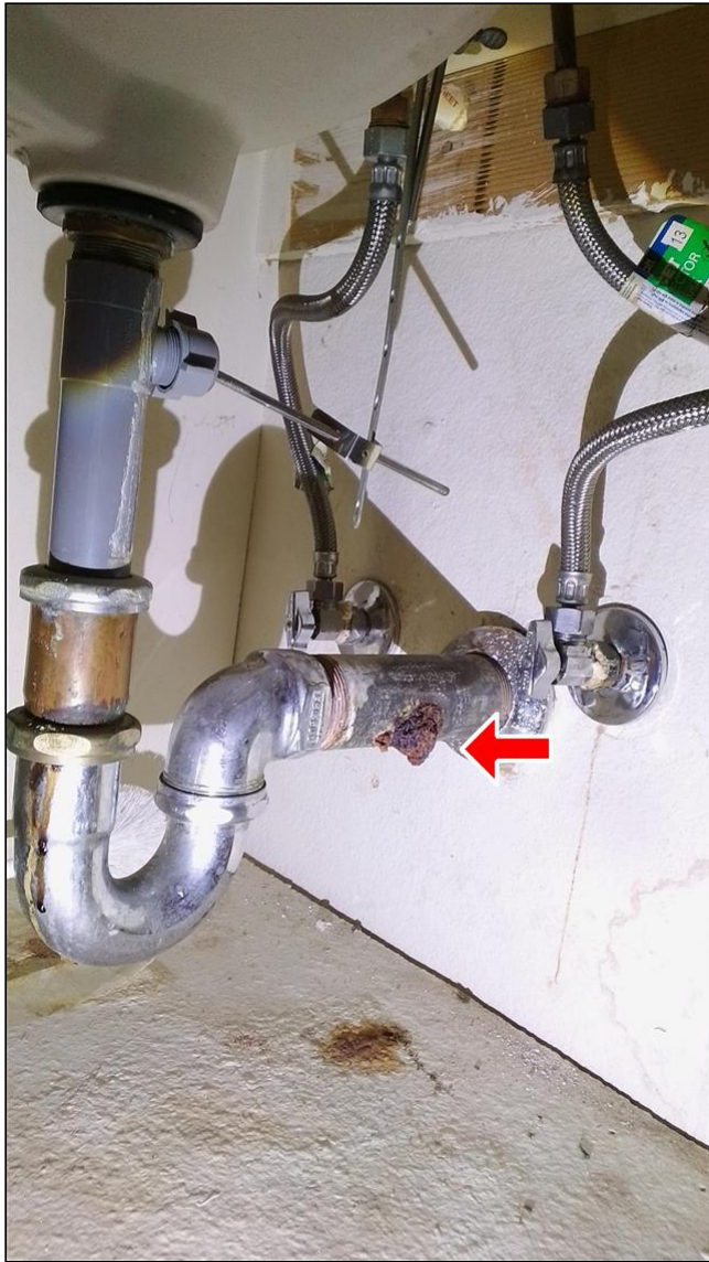
6.5 Item 4(Picture) Seepage, drain line, powder room sink
