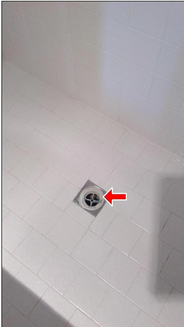
6.5 Item 1(Picture) Missing drain stop, primary bed bath
