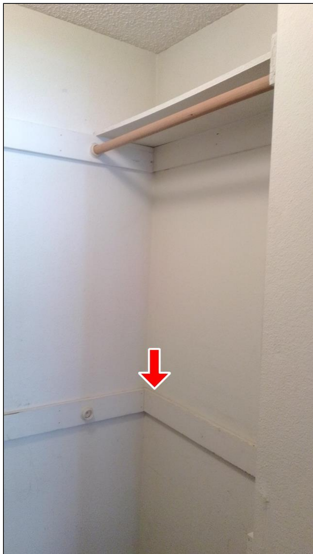
4.8 Item 1(Picture) Missing hanger rod, 2nd floor NE bed closet
