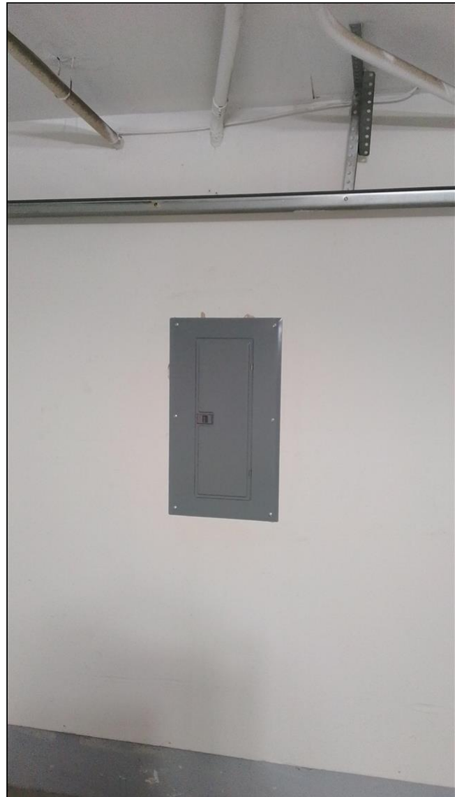
5.1 Item 2(Picture) Main distribution panel
