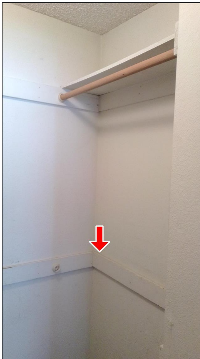
4.8 Item 1(Picture) Missing hanger rod, 2nd floor NE bed closet
