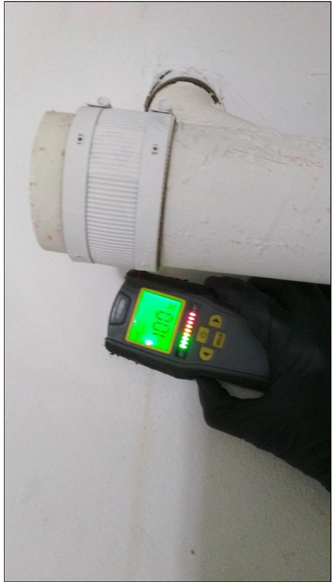
3.2 Item 4(Picture) Elevated moisture levels
