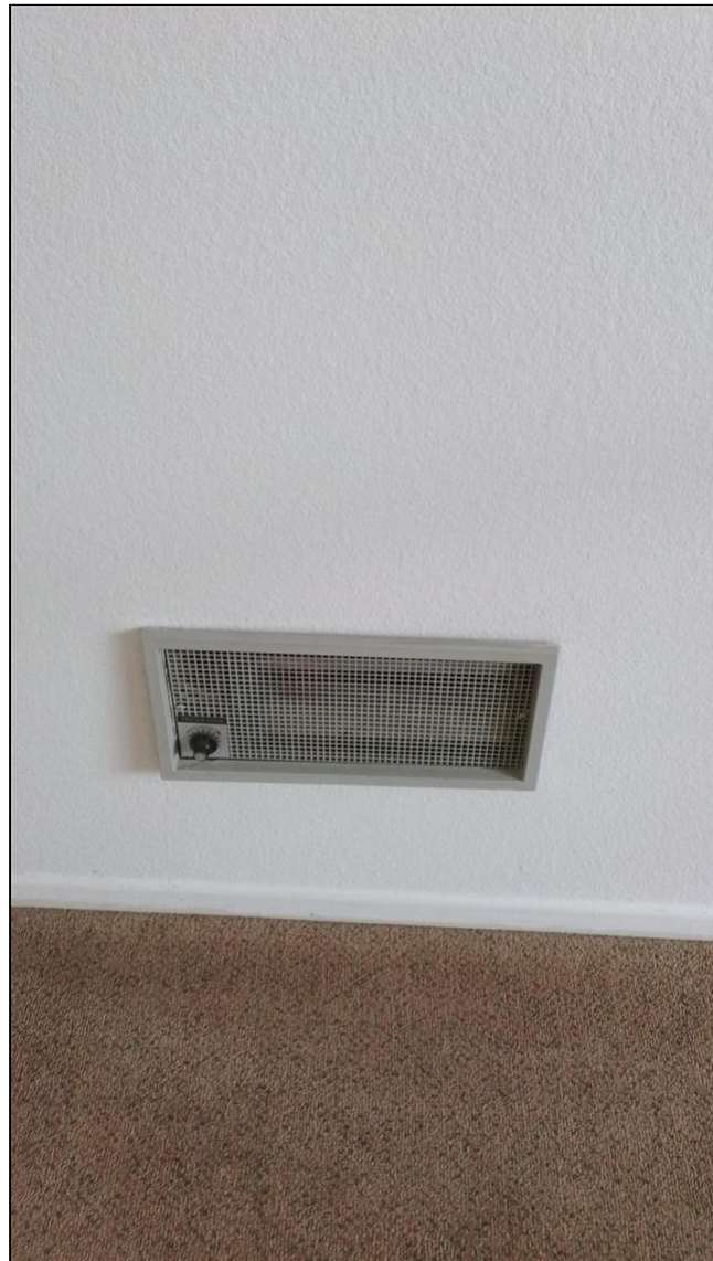
9.0 Item 1(Picture) Electric wall heater #1, 2nd floor SE bedroom
