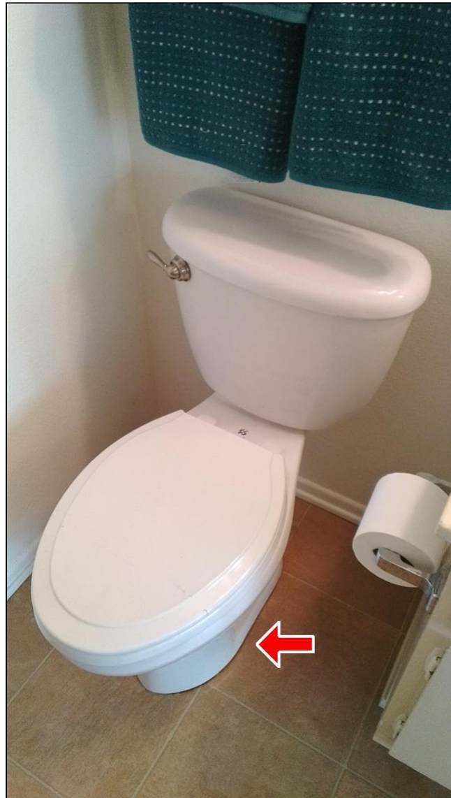
6.5 Item 3(Picture) Loose toilet, powder room off kitchen
