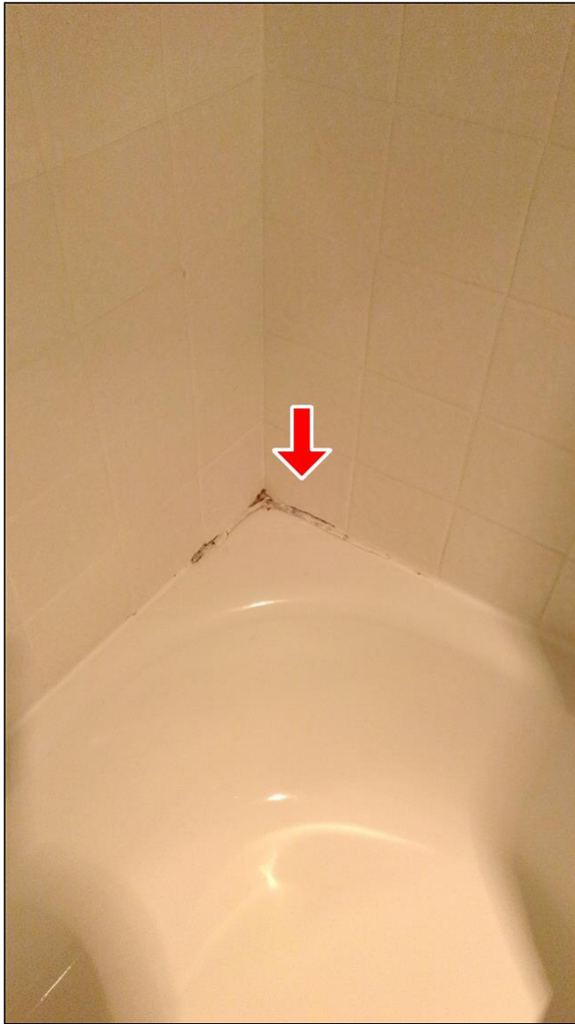
4.3 Item 3(Picture) Cracked and deteriorated seal, 2nd floor hall bathroom
