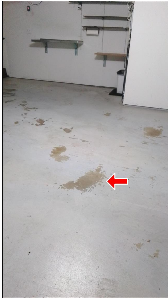
3.3 Item 1(Picture) Garage surface
