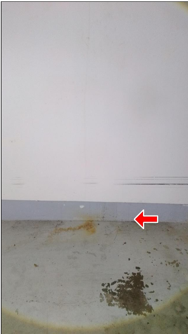
3.2 Item 1(Picture) Signs of leaking, garage south wall
