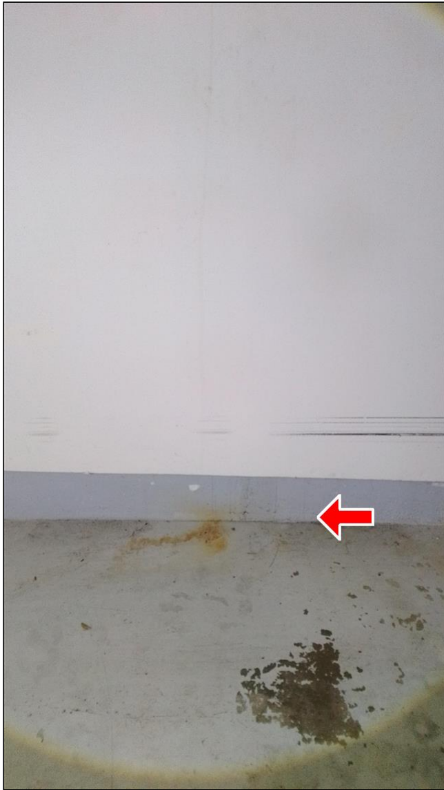
3.2 Item 1(Picture) Signs of leaking, garage south wall
