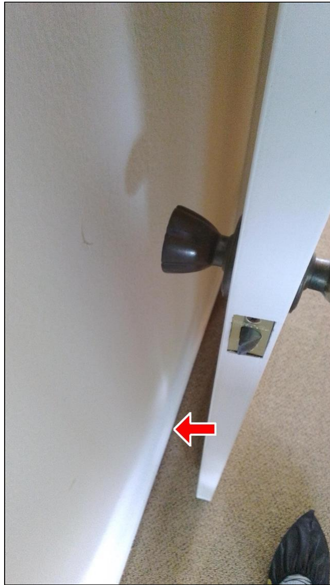
4.6 Item 1(Picture) Missing door stop
