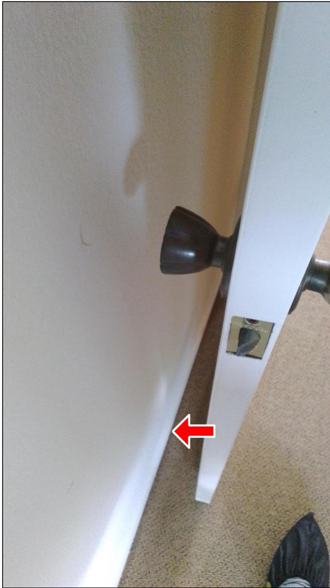
4.6 Item 1(Picture) Missing door stop
