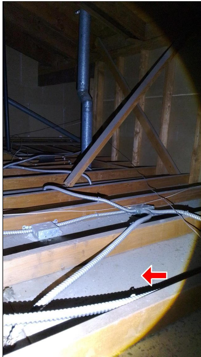
10.0 Item 1(Picture) Missing attic insulation
