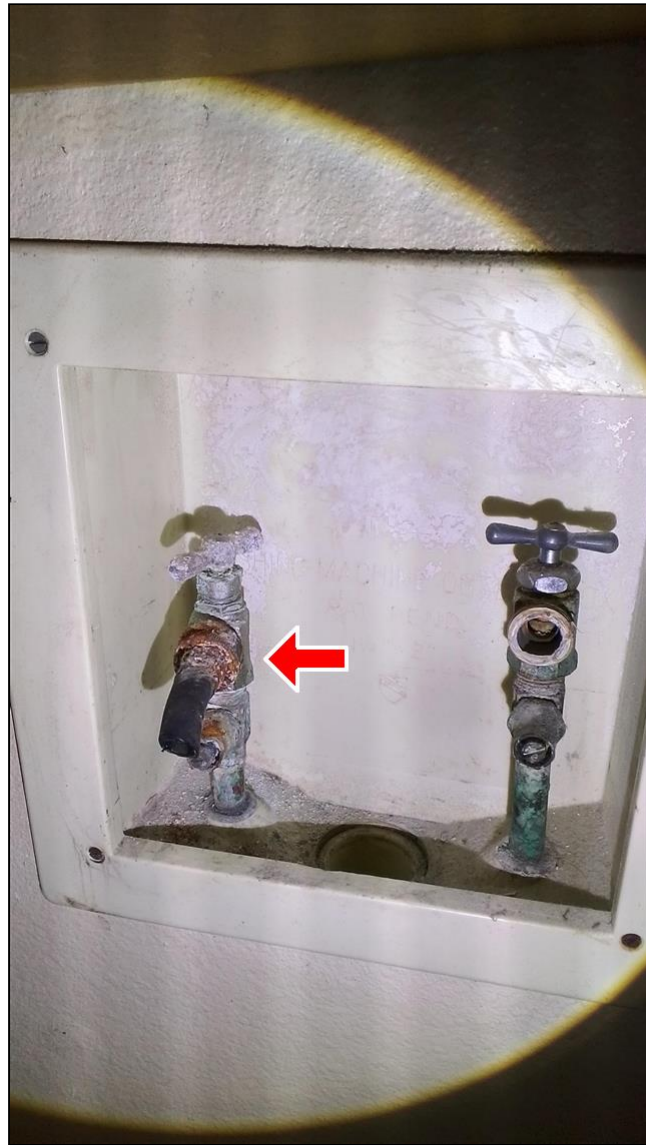
6.3 Item 3(Picture) Washer water supply, laundry closet
