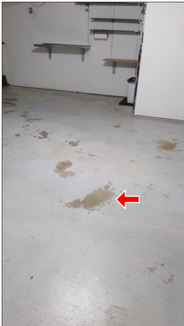
3.3 Item 1(Picture) Garage surface
