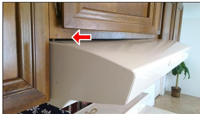
7.2 Item 1(Picture) Range hood, loose from upper cabinet
