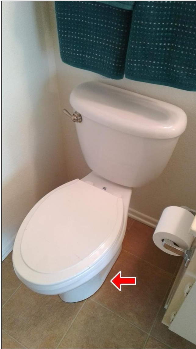
6.5 Item 3(Picture) Loose toilet, powder room off kitchen
