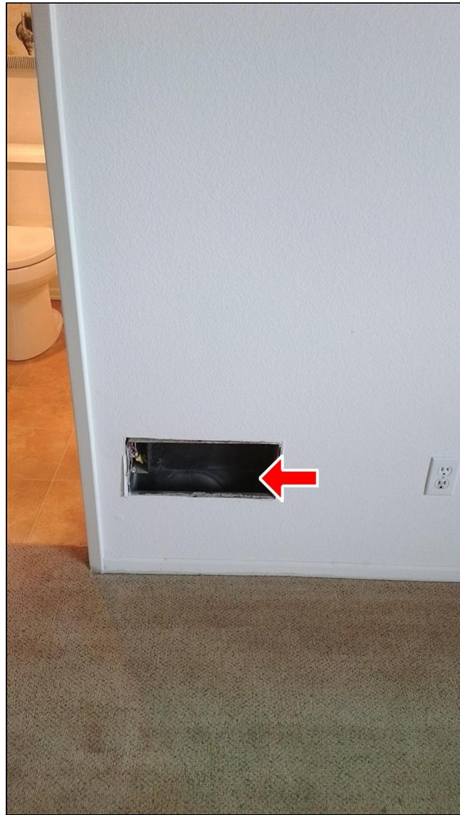
9.0 Item 6(Picture) Wall heater missing, primary bedroom
