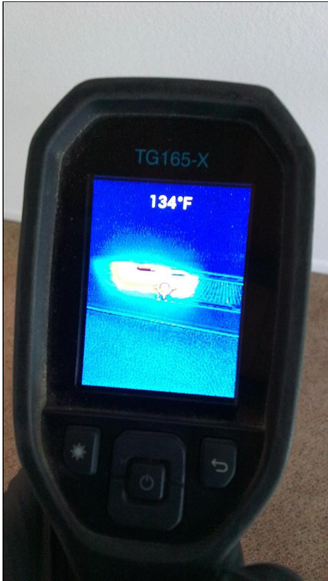
9.1 Item 1(Picture) Electric wall heater #1 temperature
