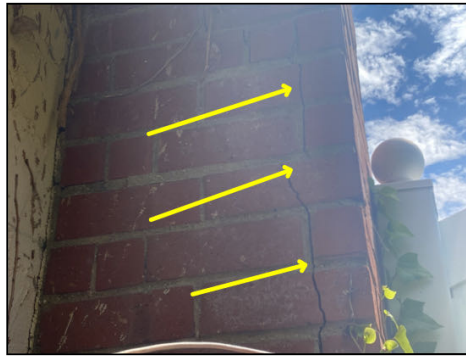
Large cracking or chipping observed - needs to be serviced
