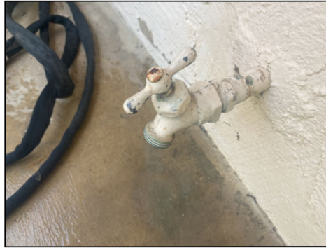
Exterior hose faucet(s) leaked at handle(s) when operated - needs to be serviced
