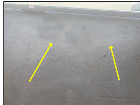
Small cracks in areas - recommend servicing
