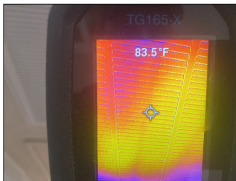
Temperature at Air Return
