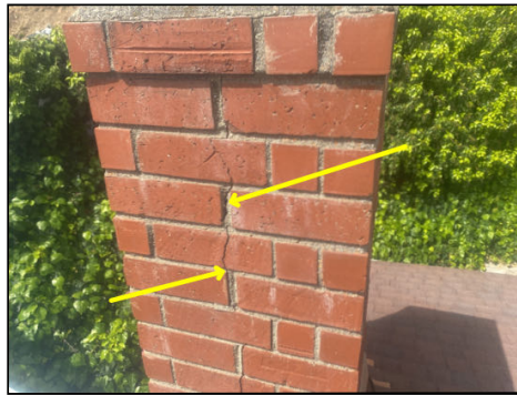
Cracks in bricks - recommend further evaluation
