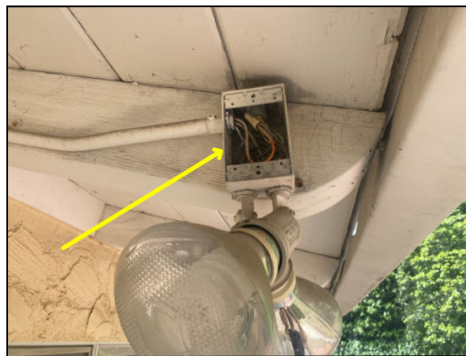
Junction box missing cover - needs to be installed
