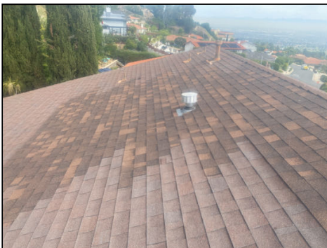
Patching observed in areas on roof materials - inspector is unable to guarantee the adequacy of these repairs - recommend maintaining a continuous water tight seal in these areas
