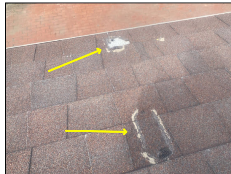
Missing/damaged shingles/tiles in one area- needs to be serviced
