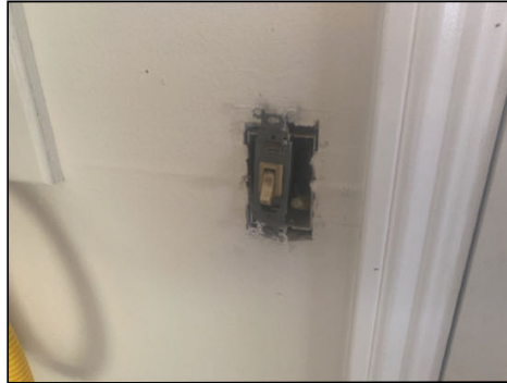
Loose switches - needs to be serviced
