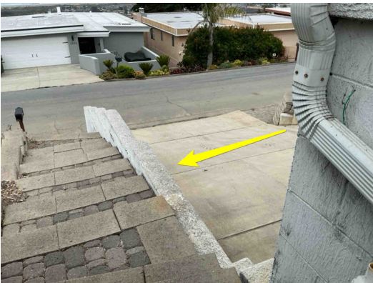
Missing required railings/ fall hazard
