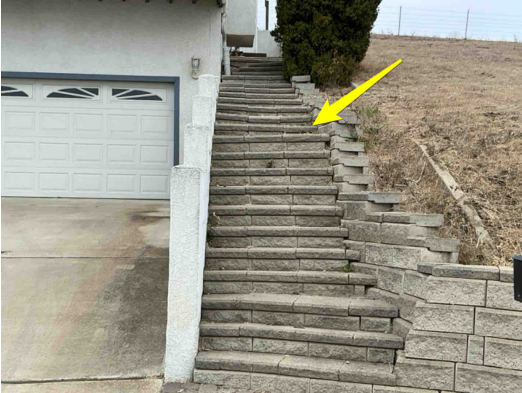
Uneven treads/ trip hazards/ no graspable handrails
