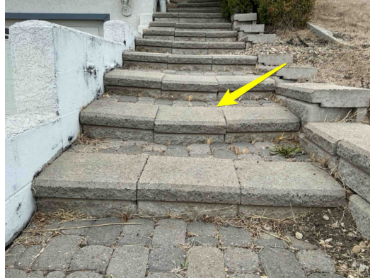
Uneven treads/ trip hazards
