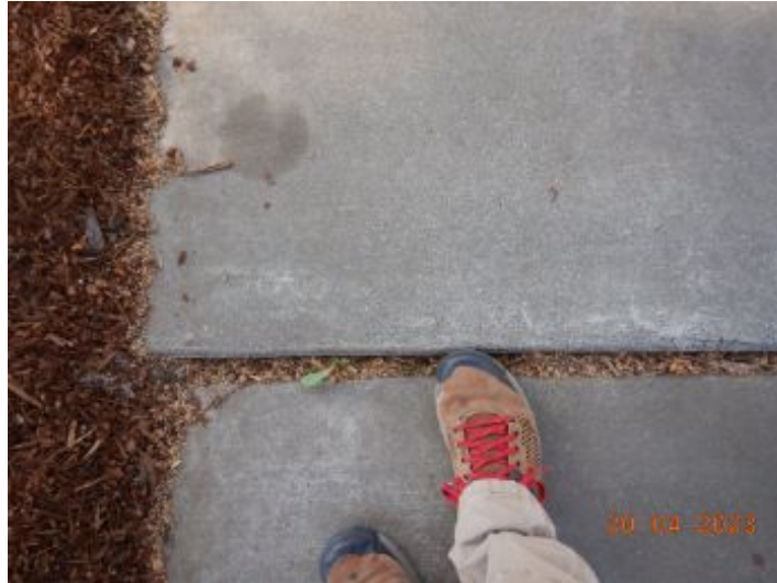
Example of trip hazard
