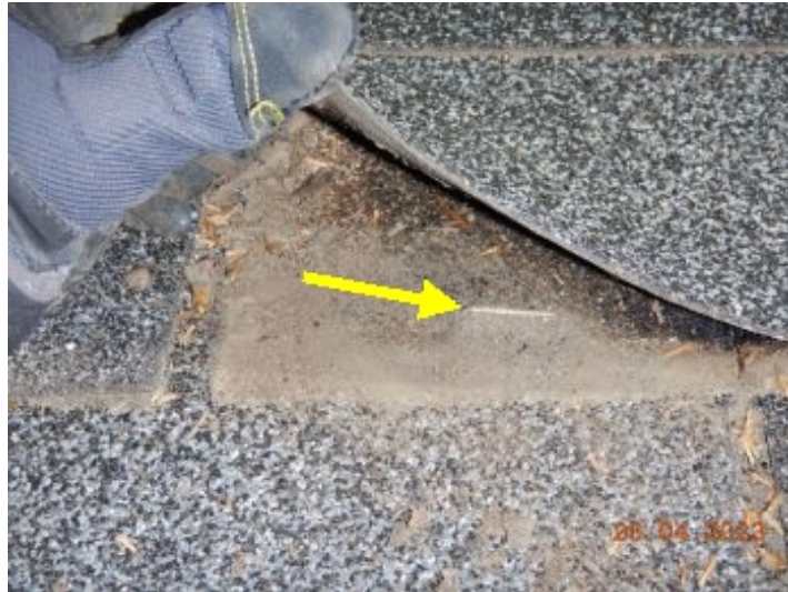
Example of fastener backing out
