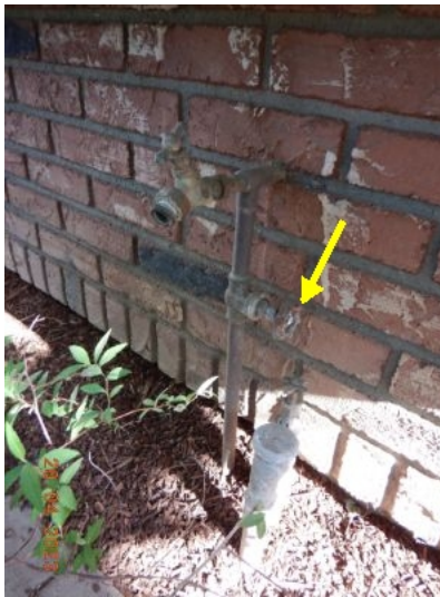
Main water shutoff
