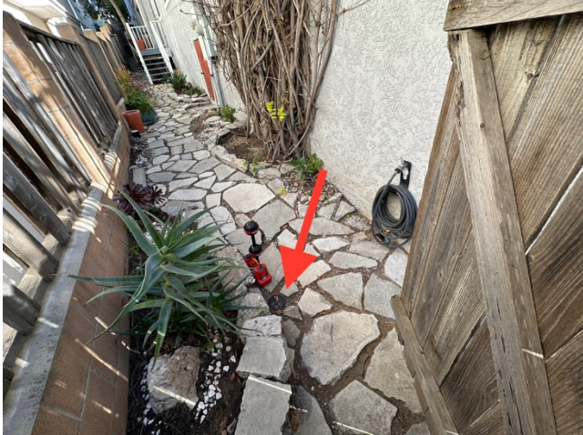
Location of root intrusion from fiberglass liner to plastic cleanout. 3' deep.
