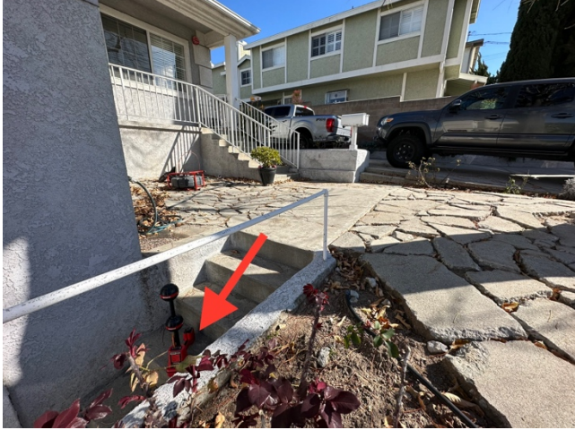
Location of heavy root intrusion in fiberglass liner. 3.5' deep under tool.
