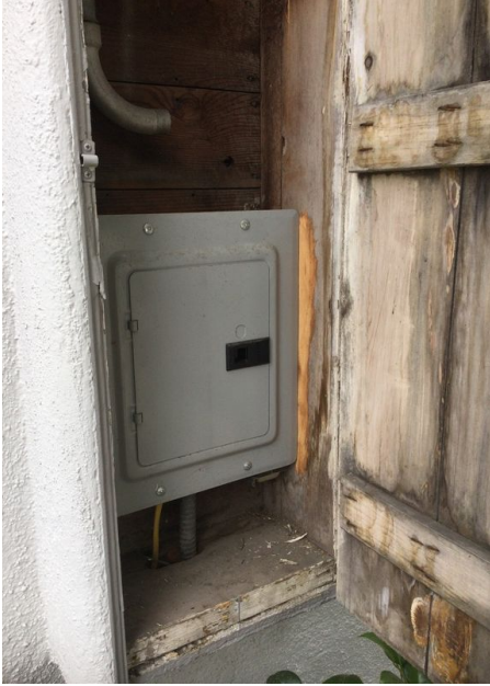
Left Exterior Sub Panel
