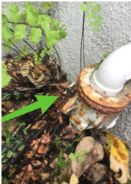
Main Shut Off Valve
