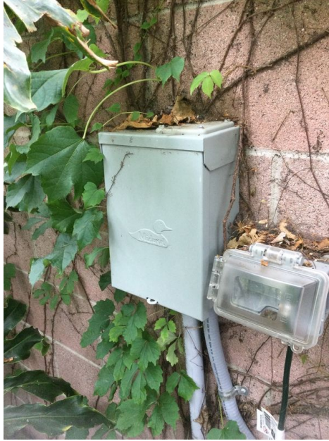
Spa Sub Panel
