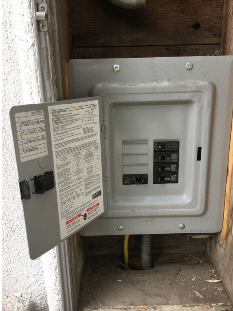
Left Exterior Sub Panel
