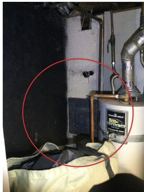
Garage Interior Sub Panel
