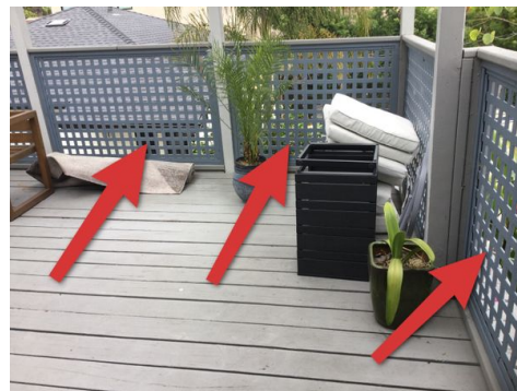
Missing Sufficient Baluster Materials
