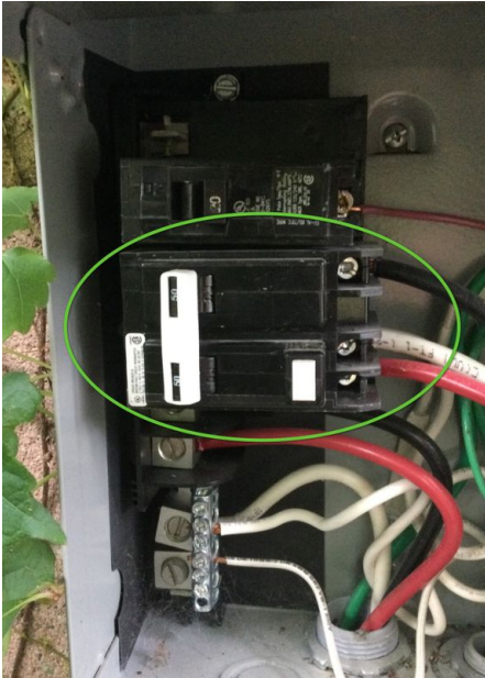
GFI Breaker at Spa Sub Panel
