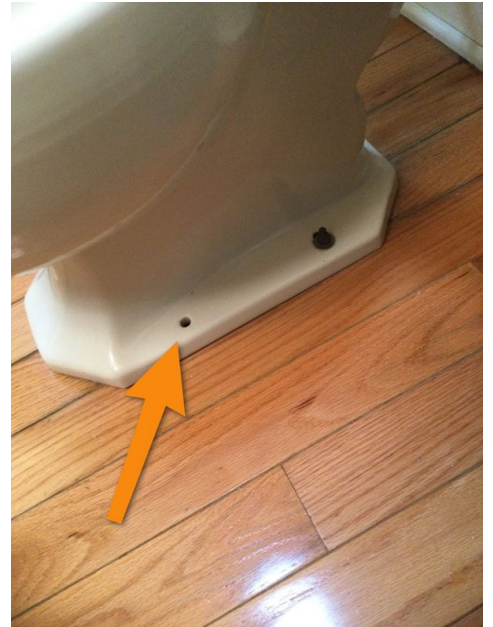
1st Floor Hallway Bathroom-Missing Anchor
