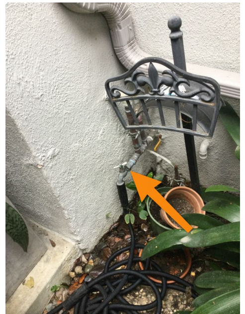
Rear Exterior Leaking Bib
