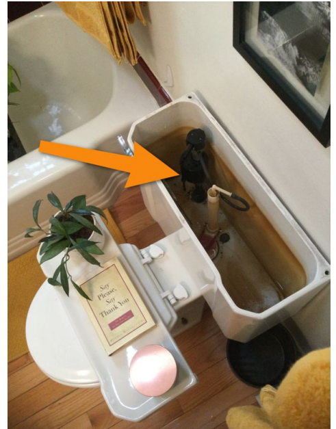
1st Floor Hallway Bathroom-Faulty ReFill
