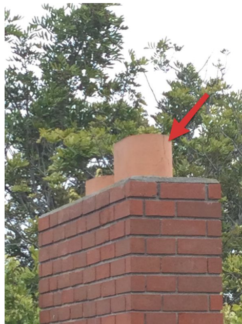
Cracks in Liner
