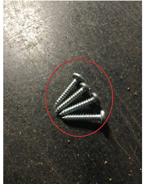
Garage Interior Sub Panel
