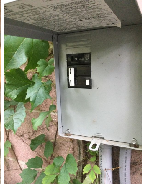
Exterior Spa Sub Panel
