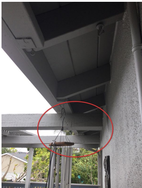
2nd Floor Balcony-Missing Ledger/Irregular Attachment Bedroom
