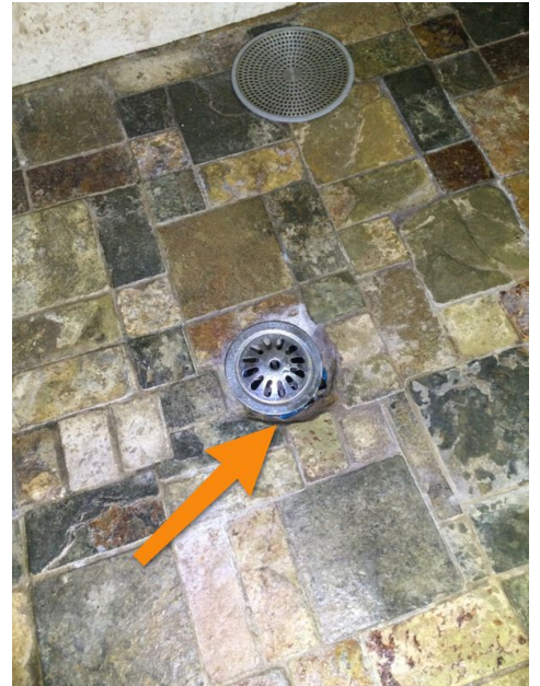
2nd Floor Master Bathroom Shower Drain Grate
