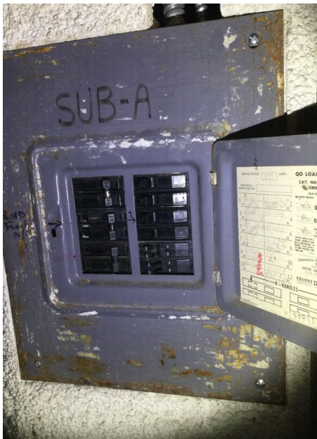
Garage Interior Sub Panel
