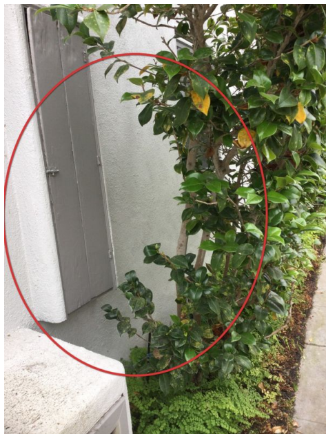
Left Exterior Sub Panel
