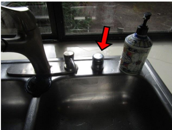
Kitchen: Water leaking from the dishwasher.
