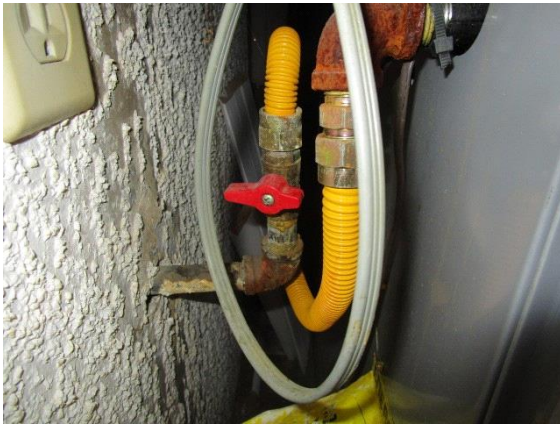
Heating: Shut-off valve
