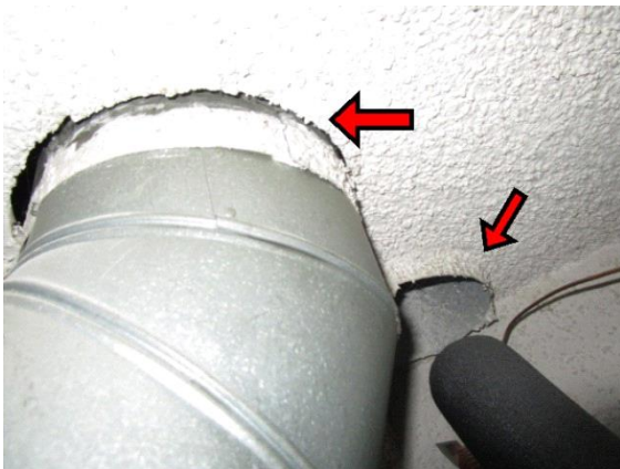
Laundry Facilities: Two air ducts
