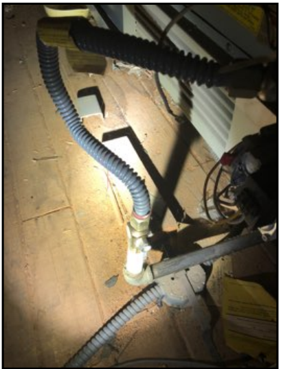
The furnace has a gas shut off.
