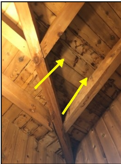
Evidence of what appears to be old water stained noted inside the master bedroom closet area on the ceiling.
