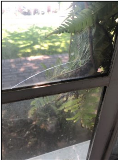
Two cracked glass windows are located inside the living room area.
