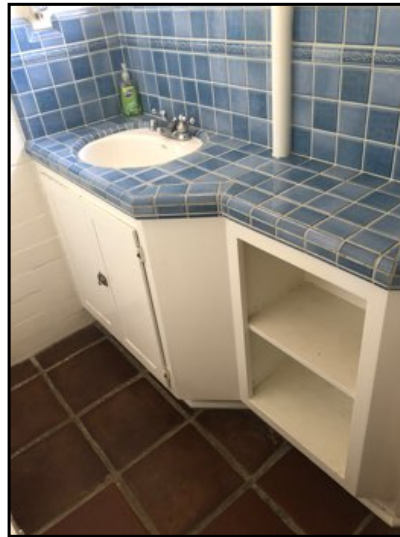
Appeared functional and in satisfactory condition, at time of inspection.
