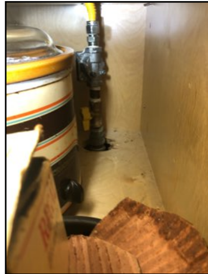
The gas cook top gas shut off is located under the cabinet.
