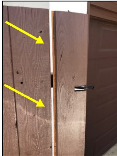
The side yard gate near the driveway has a loose plank near the lock.
