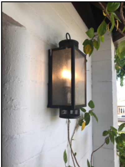
The front porch light is functional.
