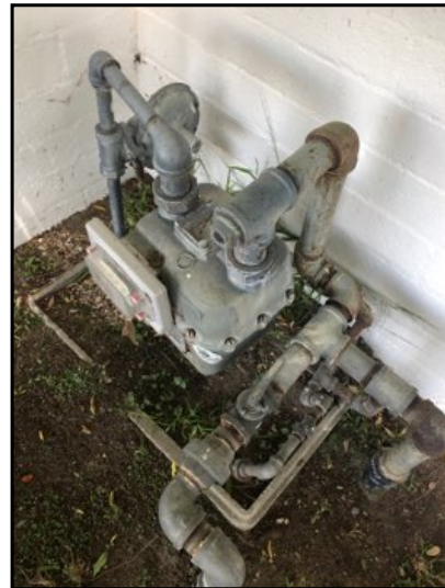
Meter located at exterior. All gas appliances have cut-off valves in line at each unit. No gas odors detected.
