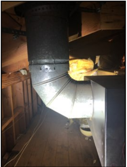
The furnace flue is vented to the exterior.
