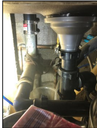
There is a hole behind the kitchen cabinet that should be closed off.
