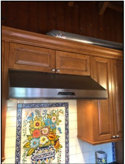
The stove hood fan is functional.
