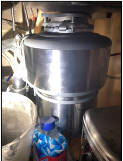
Operated - appeared functional at time of inspection.
