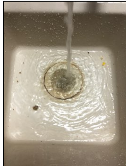
The water in the bar sink drain line moves down slow. You should have this issue corrected.
