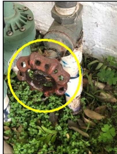
The main sprinkler shut of valve has a leak located near the gas meter. You should have this issue corrected.
