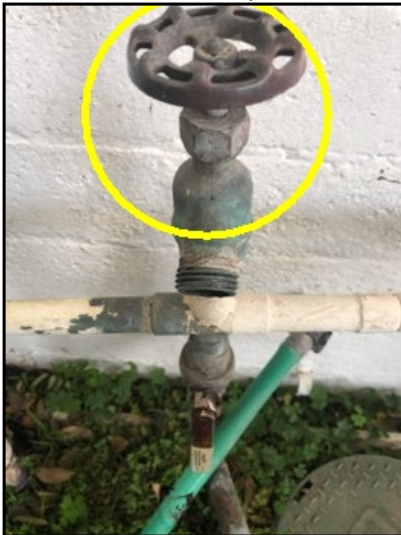
The front yard house bib shut off valve near the gas meter has a leak. You should have this issue corrected.
