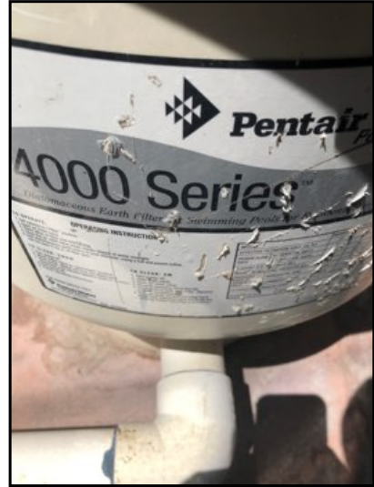
Diatom. earth filter noted.
