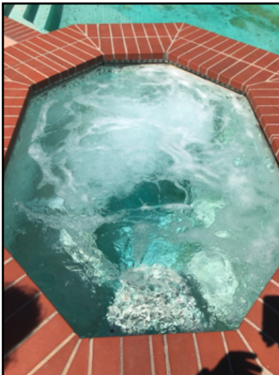
The spa tub jets are functional.
