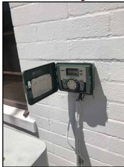
The sprinkler time is located in the rear yard near the A/C unit.
