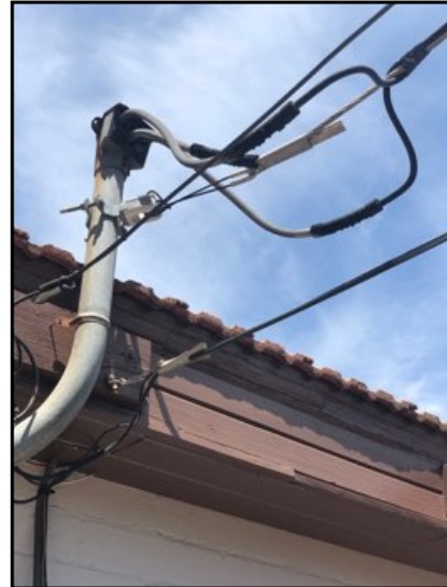
There is an overhead service drop noted.
