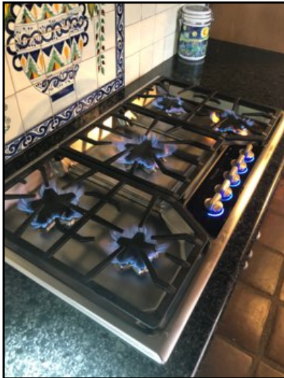
The gas cook top is functional.
