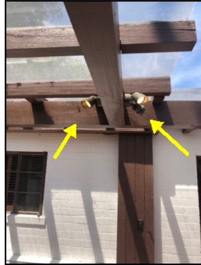
The patio lights were functional during the time of the inspection. One of the patio lights bulbs was not working.
