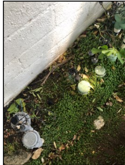
Vegetation is covering the sprinkler control station
