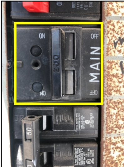
The main disconnect breaker is located inside the panel box.
