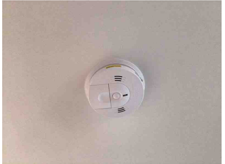
Carbon monoxide and smoke detector
