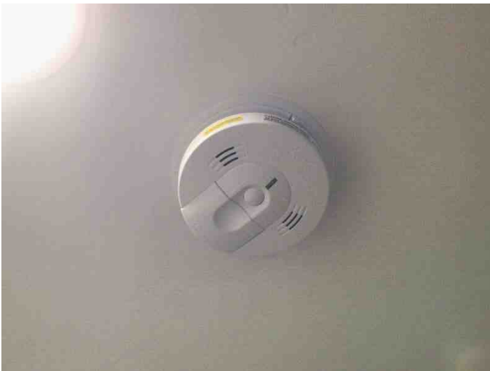
Carbon monoxide and smoke detector 1st floor
