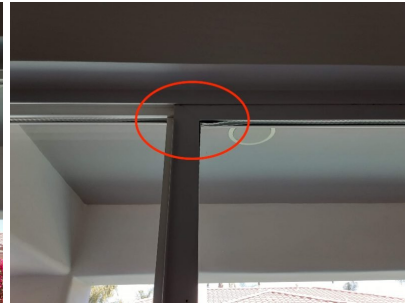
Defective Inner Seal
