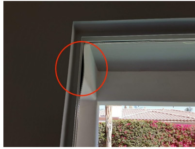
Defective Inner Seal
