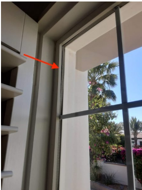
Defective Inner Seal
