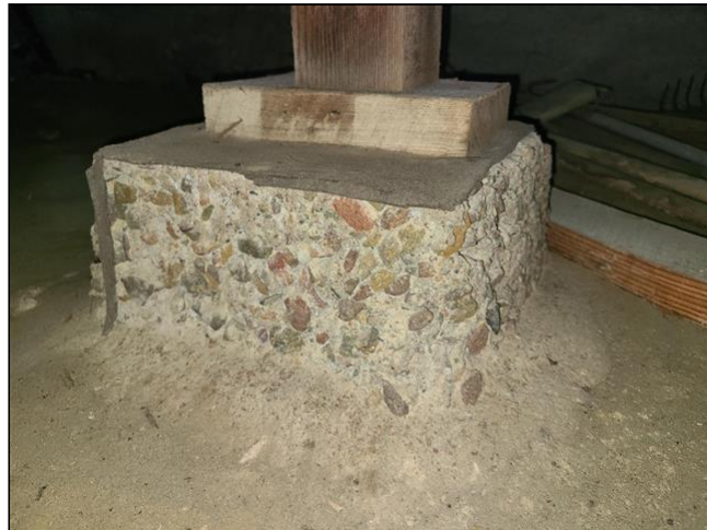
Deterioration of Piers
