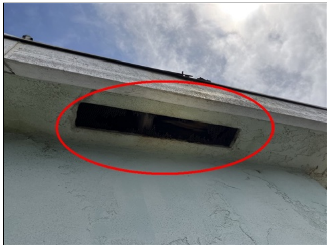
9.2 Item 2(Picture) deterioration/oxidation visible at vent screens
