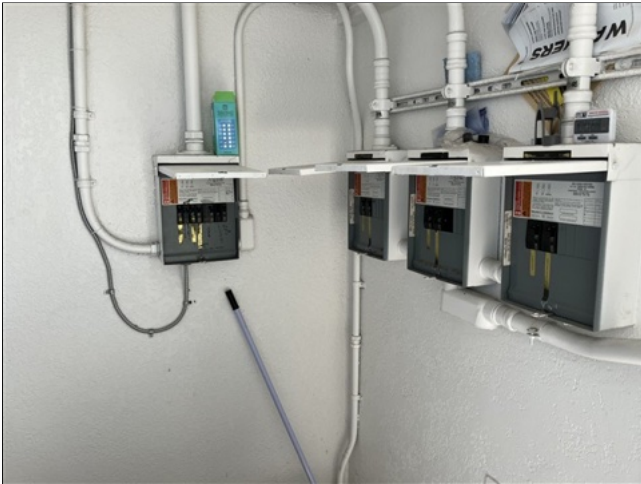
7.2 Item 4(Picture) subpanels located in the laundry room
