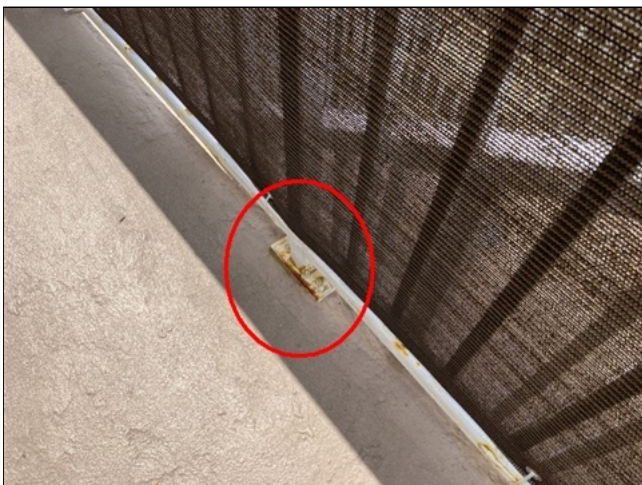
2.3 Item 15(Picture) oxidation visible at railing
