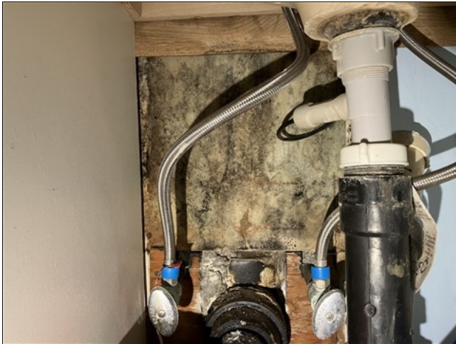
4.0 Item 5(Picture) unit 4770 bathroom #2: moisture stains or damage visible / possible evidence of fungal activity
