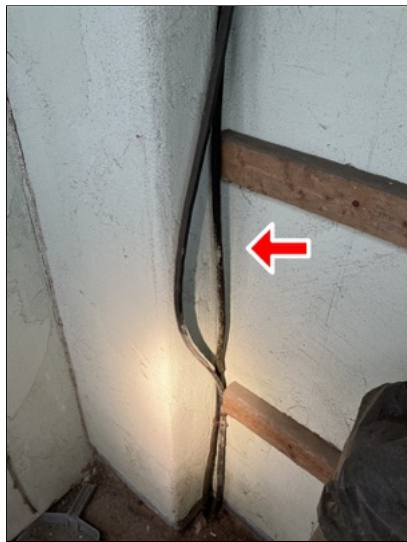
7.4 Item 1(Picture) view from second floor patio: exposed wire appeared subject to damage
