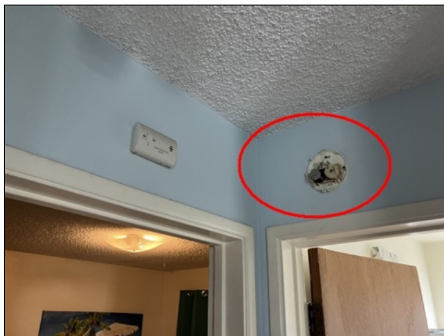
7.7 Item 4(Picture) unit 4772: missing hallway smoke detector
