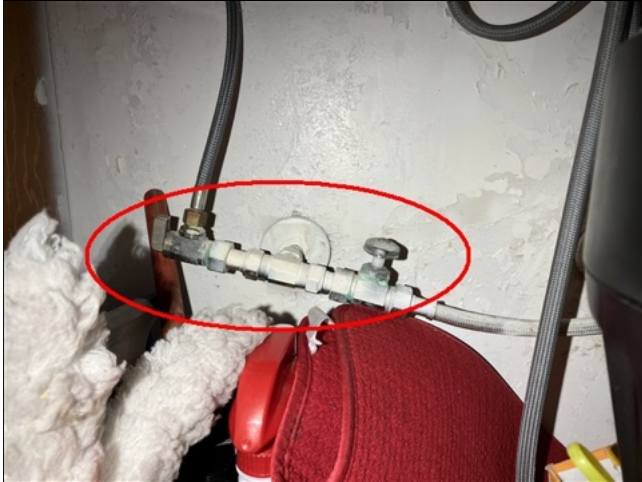
6.4 Item 1(Picture) unit 4770: aged water supply valves/hoses observed
