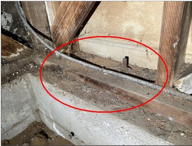
5.3 Item 6(Picture) subfloor area: possible WDO evidence or damage observed
