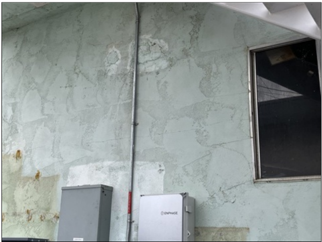
2.0 Item 4(Picture) stucco surface and paint maintenance/repairs needed
