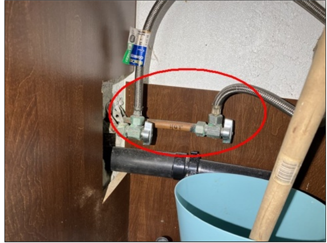
6.4 Item 6(Picture) unit 4772 (alley side): oxidation visible at valve/hoses
