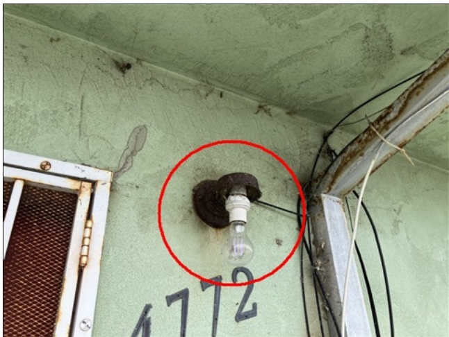
7.5 Item 2(Picture) unit 4772: aged fixture / missing cover
