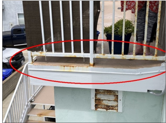
2.3 Item 7(Picture) oxidation visible at deck railing system and deck flashing
