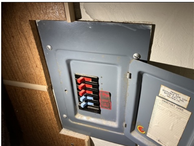
7.2 Item 2(Picture) unit 4770: electrical panel location upgrade recommended
