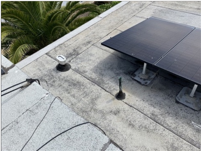
1.0 Item 5(Picture) roll roofing deterioration visible / recommend further evaluation and correction as needed
