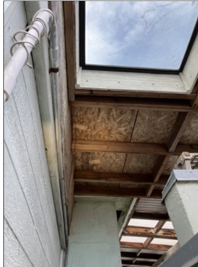
5.7 Item 2(Picture) possible evidence of modifications to original construction observed / substandard installation or building material was observed / recommend further evaluation
