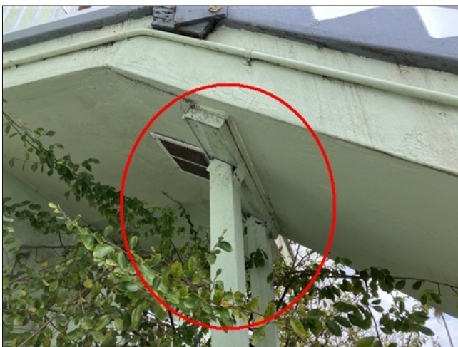
2.3 Item 9(Picture) substandard deck stair support installation observed
