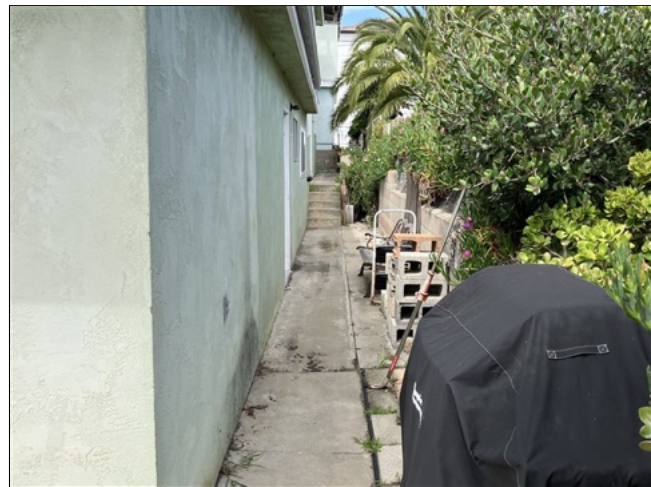
2.4 Item 4(Picture) grading or drainage improvements/ corrections are recommended to achieve positive slope away from the property
