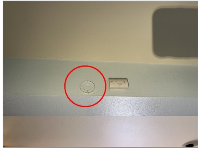
7.7 Item 6(Picture) unit 4772 (alley side): missing hallway smoke detector
