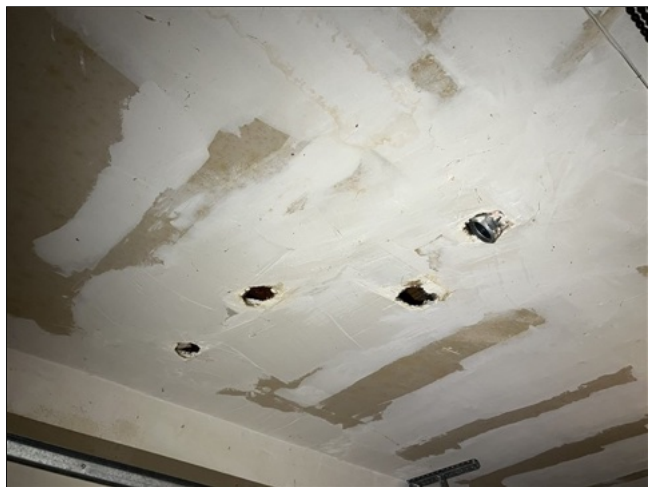
3.1 Item 1(Picture) unit 4770 garage ceiling: penetrations observed in garage firewalls
