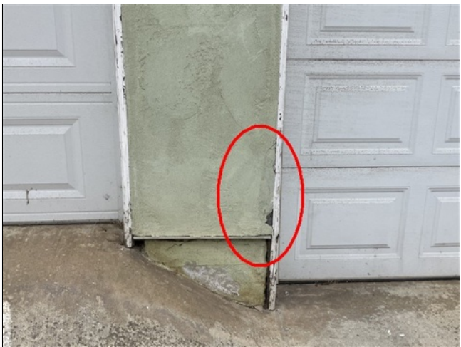
2.0 Item 2(Picture) stucco damage/defect visible // maintenance/repairs needed
