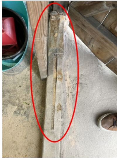
2.1 Item 6(Picture) 4772 patio door: possible WDO evidence or damage observed
