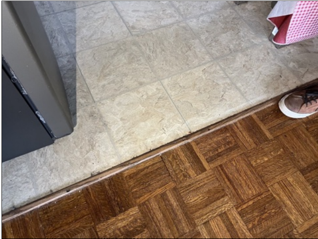
4.1 Item 1(Picture) unit 4768: aged flooring / maintenance/repairs needed
