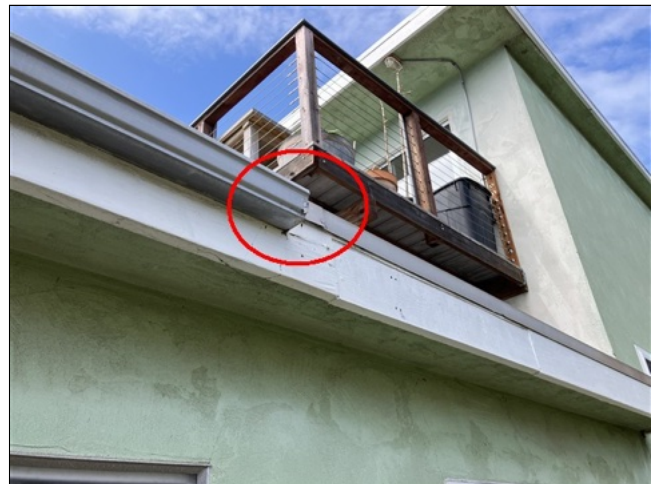
1.1 Item 2(Picture) missing gutter components
