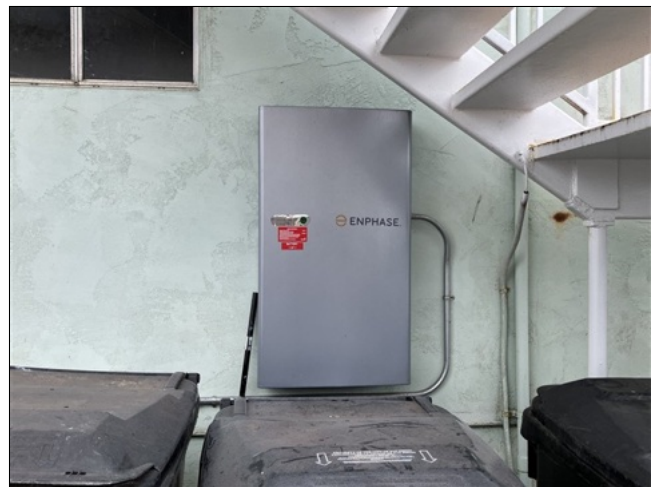
7.8 Item 2(Picture) solar system and components were not inspected or tested as part of the scope of this inspection
