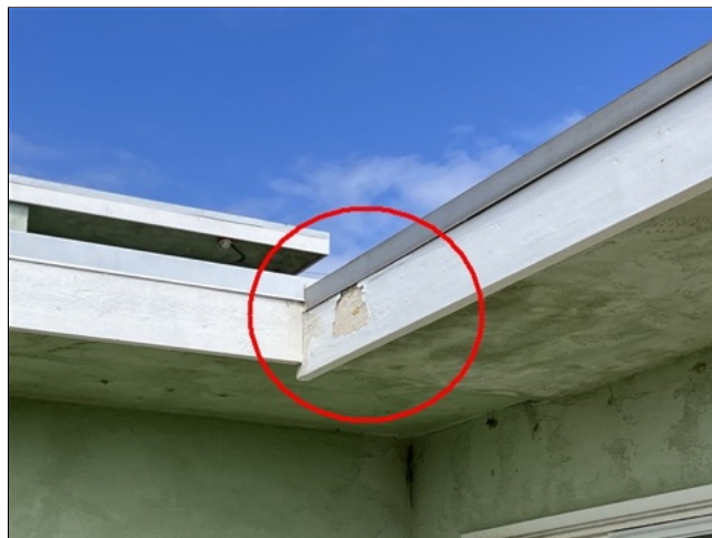
2.5 Item 2(Picture) fascia paint maintenance/repairs needed
