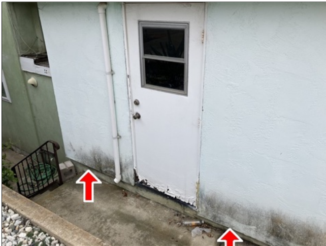
2.0 Item 11(Picture) stucco stains visible
