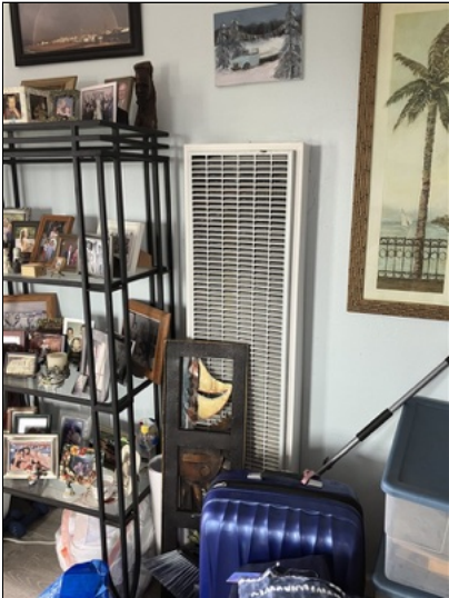
8.2 Item 2(Picture) unit 4772 wall furnace: no visible maintenance record observed
