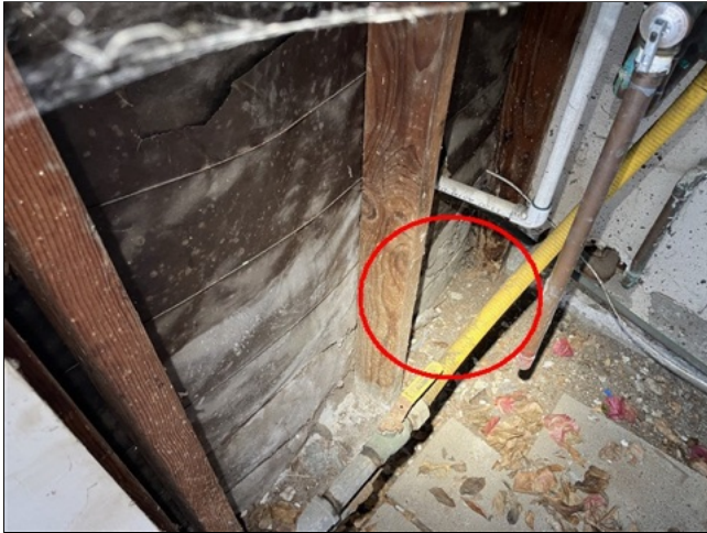
6.0 Item 1(Picture) water heater storage shed: possible WDO evidence or damage observed
