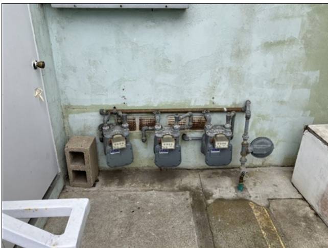
6.2 Item 1(Picture) 3 meters and main disconnects
