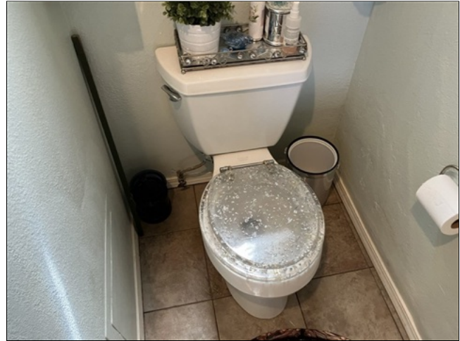
6.5 Item 2(Picture) unit 4772 (alley side): loose toilet
