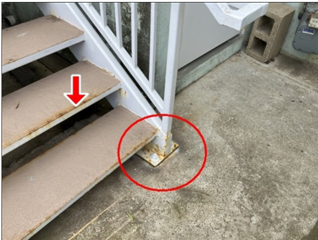
2.3 Item 1(Picture) oxidation visible at stair system
