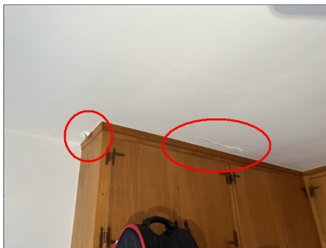
4.0 Item 3(Picture) unit 4772: ceiling paint defects observed
