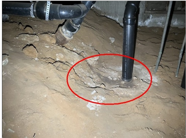
6.3 Item 4(Picture) evidence of past leakage observed / no visible leaking observed / recommend sewer camera inspection
