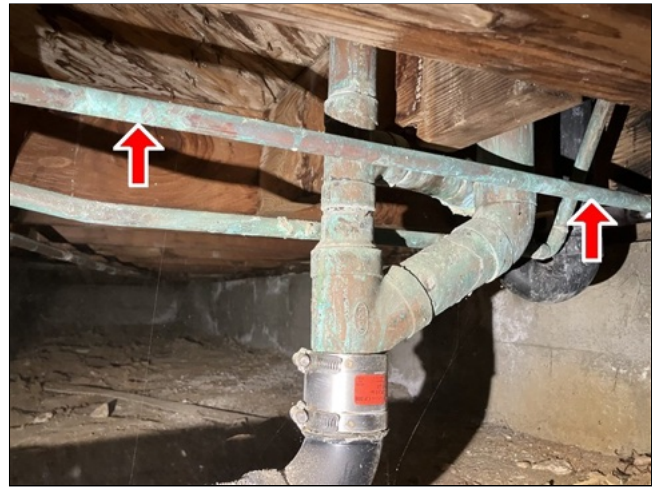
6.4 Item 8(Picture) subfloor area: oxidation visible at water supply pipe
