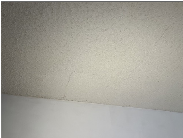
4.8 Item 1(Picture) popcorn ceiling texture materials installed before 1978 may contain asbestos
