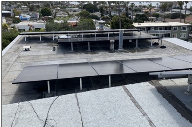
7.8 Item 3(Picture) solar system and components were not inspected or tested as part of the scope of this inspection
