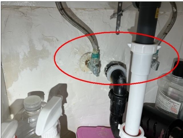
6.4 Item 3(Picture) unit 4772: aged water supply valves/hoses observed
