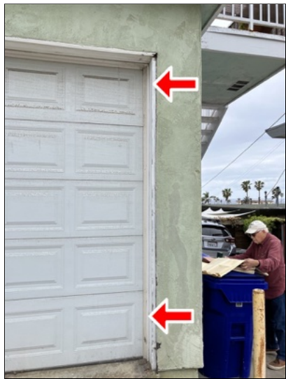
3.4 Item 1(Picture) missing garage door trim
