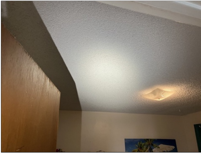
7.7 Item 5(Picture) unit 4772: missing bedroom smoke detectors
