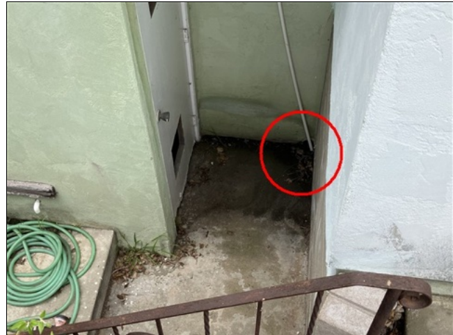
2.4 Item 2(Picture) exterior drain observed / evidence of inadequate drainage observed
