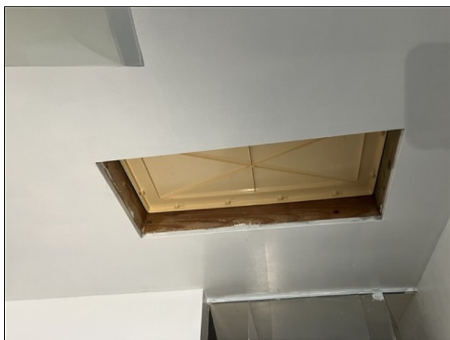
4.0 Item 2(Picture) unit 4770 bathroom: unfinished ceiling / possible abandoned skylight
