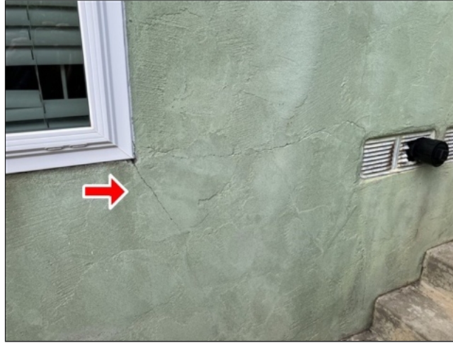
2.0 Item 10(Picture) crack visible at stucco
