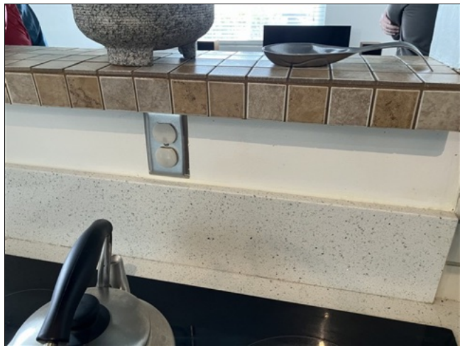
7.6 Item 3(Picture) unit 4770: recommend evaluation and upgrade of any non-GFCI outlets
