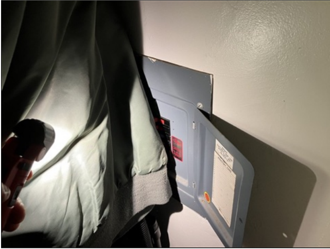
7.2 Item 3(Picture) unit 4772: electrical panel location upgrade recommended
