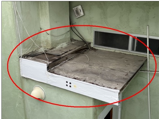
1.0 Item 1(Picture) water heater utility room roof: substandard installation or building material was observed / recommend further evaluation
