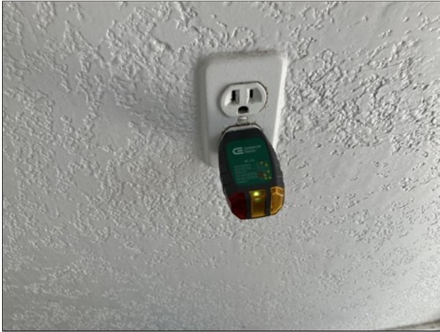
7.6 Item 5(Picture) laundry room: non-grounded three-pronged outlets observed
