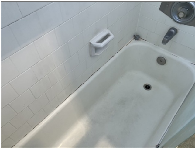
4.6 Item 2(Picture) unit 4772: aged tub/wall surround system observed
