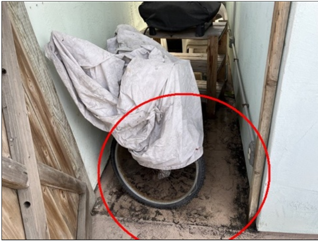
2.3 Item 16(Picture) ponding water observed / evidence of possible inadequate drainage
