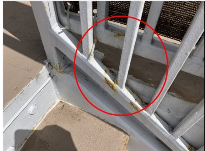
2.3 Item 14(Picture) oxidation visible at railing
