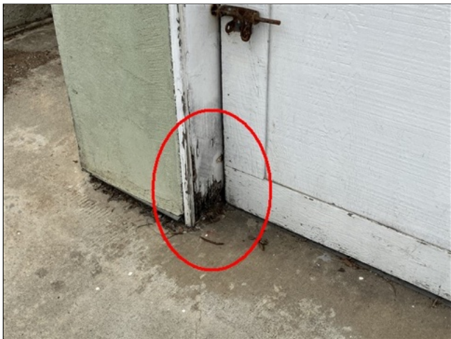
3.4 Item 2(Picture) possible WDO evidence or damage observed at garage door jamb
