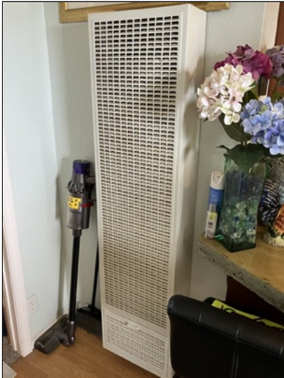
8.2 Item 3(Picture) unit 4772 (alley-side) wall furnace: no visible maintenance record observed
