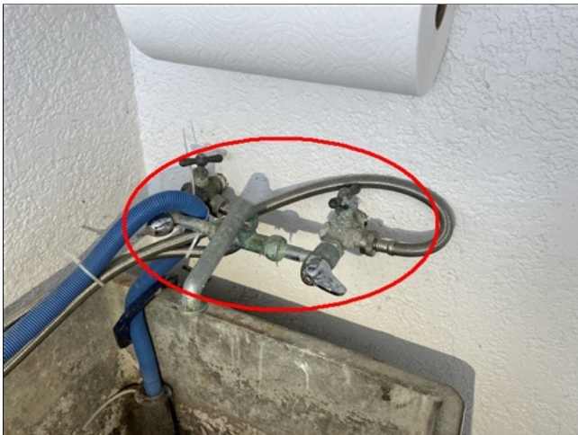
6.5 Item 3(Picture) laundry room: aged sink basin faucet
