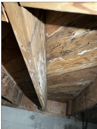
5.2 Item 3(Picture) subfloor area: moisture stains or damage visible
