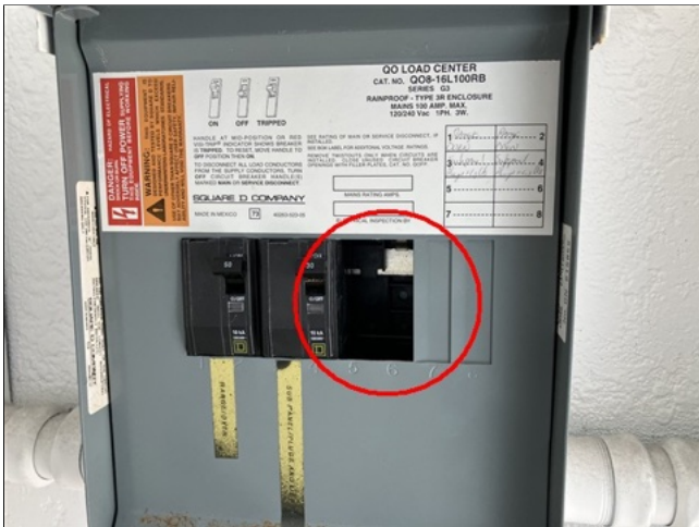
7.3 Item 3(Picture) laundry room subpanel: missing breaker blank
