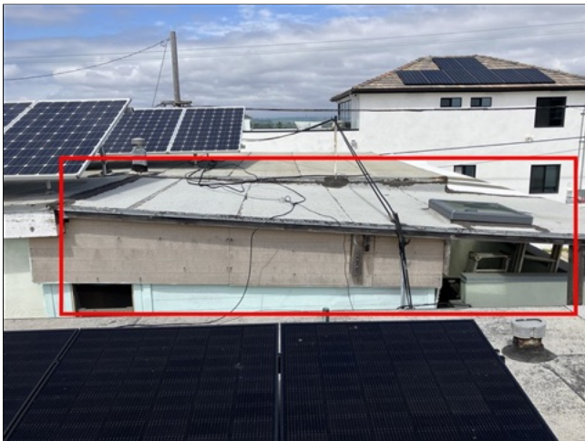
5.7 Item 3(Picture) possible evidence of modifications to original construction observed / substandard installation or building material was observed / recommend further evaluation
