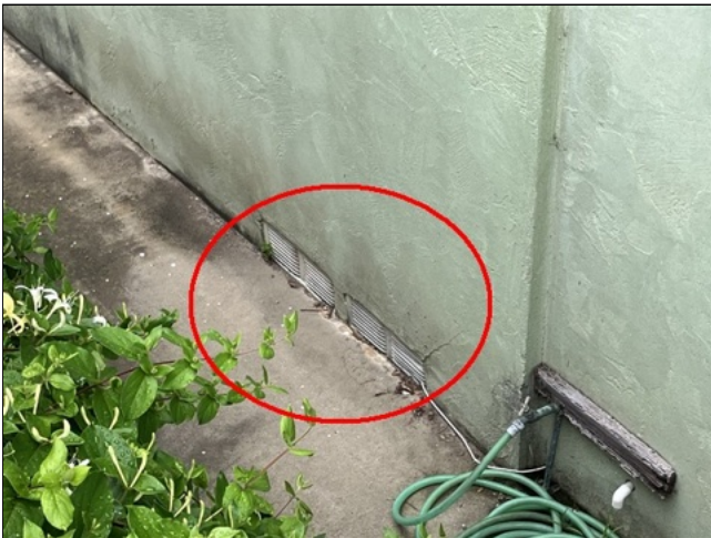
9.2 Item 6(Picture) vent appeared below grade level or was susceptible to moisture intrusion
