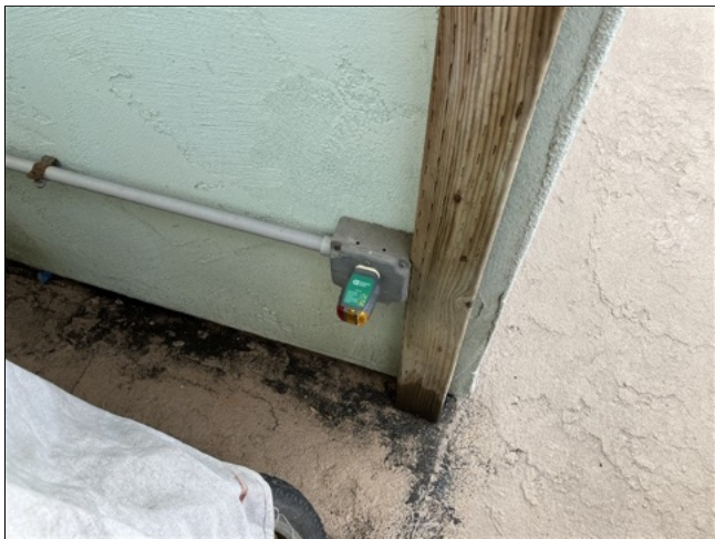
7.6 Item 4(Picture) exterior patio: recommend evaluation and upgrade of any non-GFCI outlets
