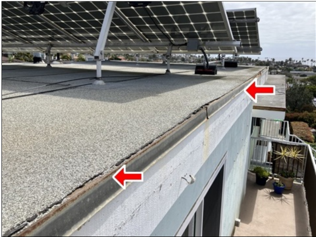
1.0 Item 3(Picture) roll roofing defects observed around the perimeter
