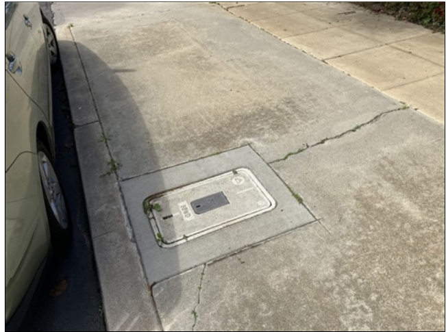
6.1 Item 2(Picture) water meter and main shut-off
