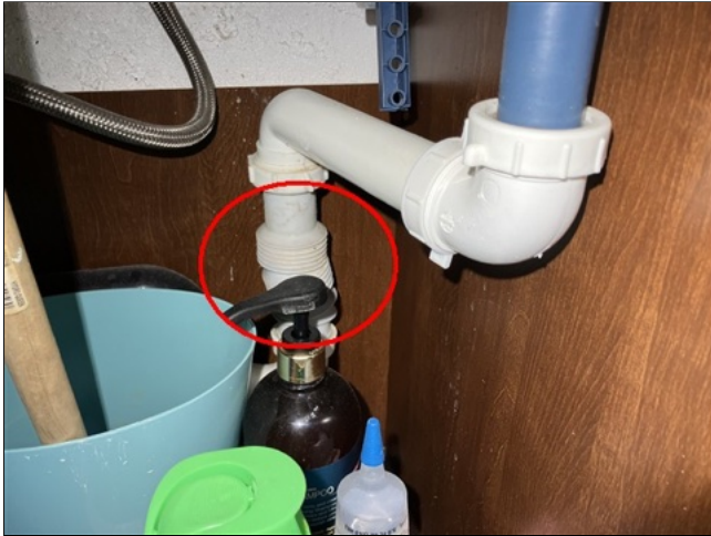
6.3 Item 5(Picture) unit 4772 (alley side) bathroom: substandard drain material
