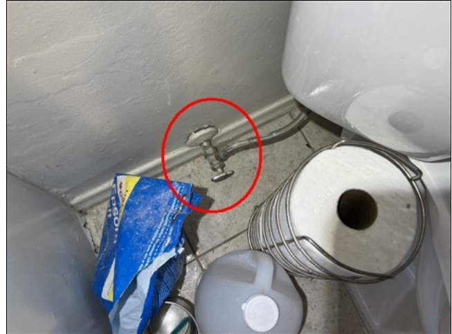
6.4 Item 2(Picture) unit 4772: aged water supply valves/hoses observed
