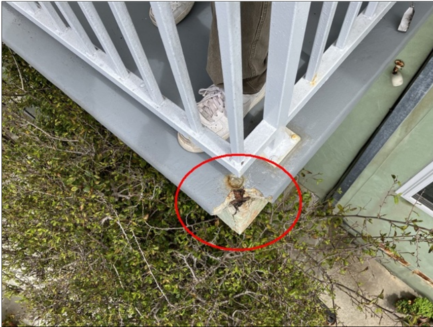
2.3 Item 4(Picture) concrete spalling visible / recommend further evaluation and correction as needed
