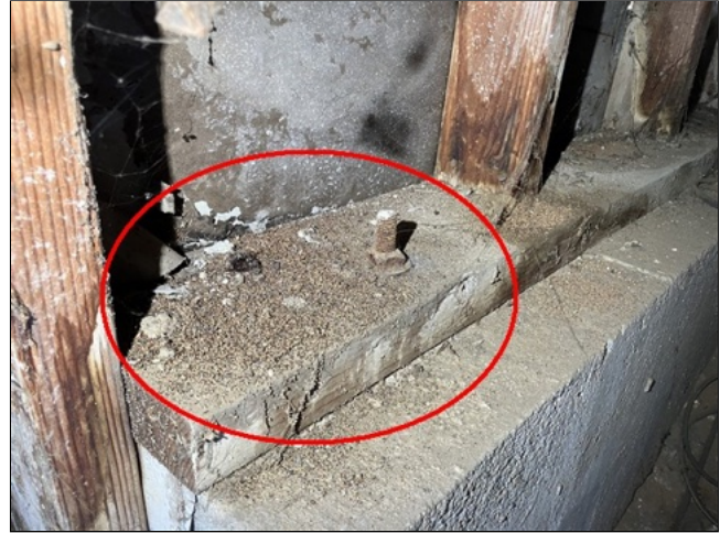
5.3 Item 5(Picture) subfloor area: possible WDO evidence or damage observed
