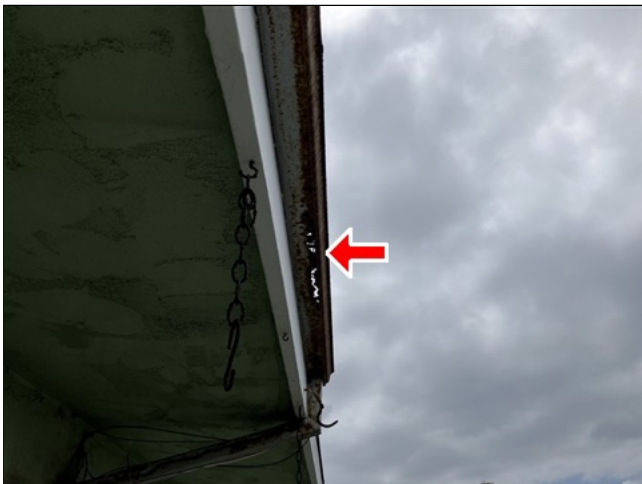
1.1 Item 1(Picture) oxidation defects visible at rain gutters
