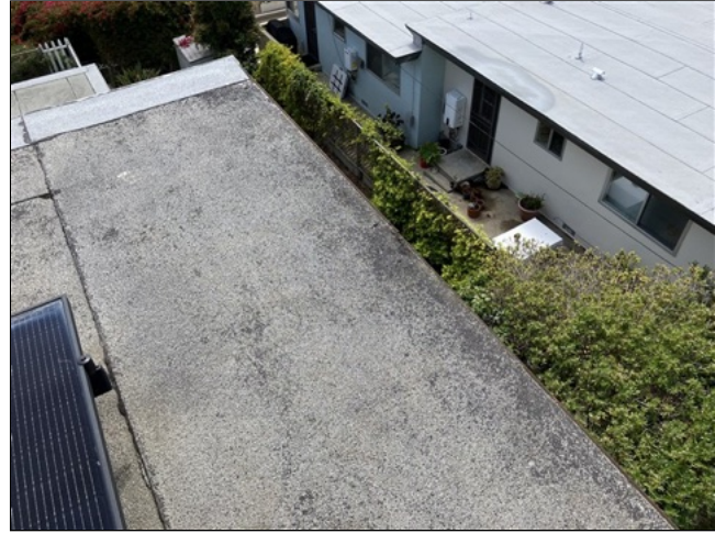
1.0 Item 9(Picture) roll roofing deterioration visible / recommend further evaluation and correction as needed
