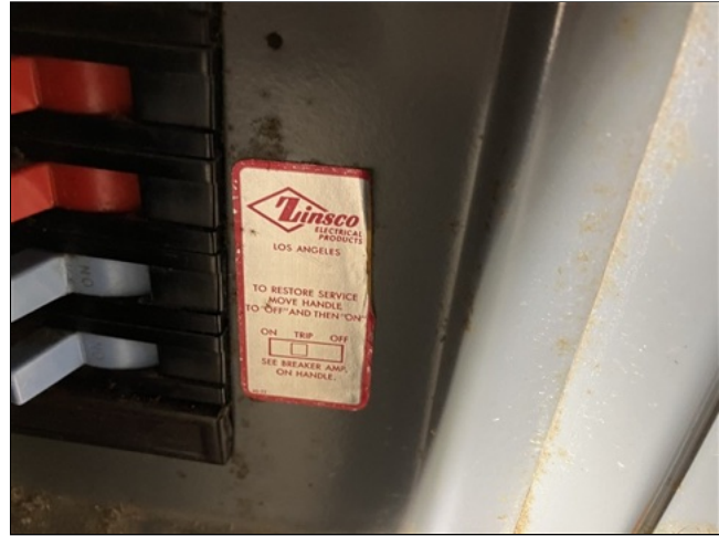
7.3 Item 2(Picture) unit 4770: a Zinsco panel performance and safety inspection by a qualified person is recommended
