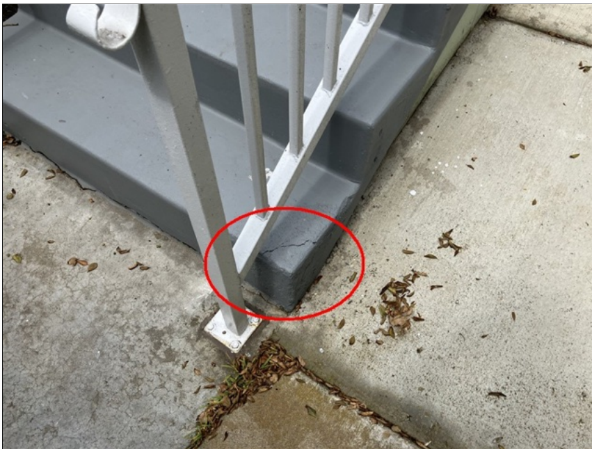
2.3 Item 8(Picture) cracks visible at concrete stairs
