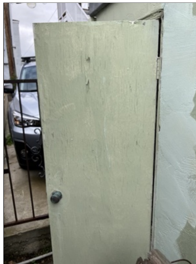
2.1 Item 4(Picture) stairwell storage area door defects observed
