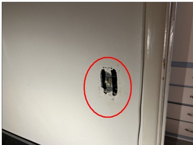
7.5 Item 3(Picture) unit 4772: missing switch cover
