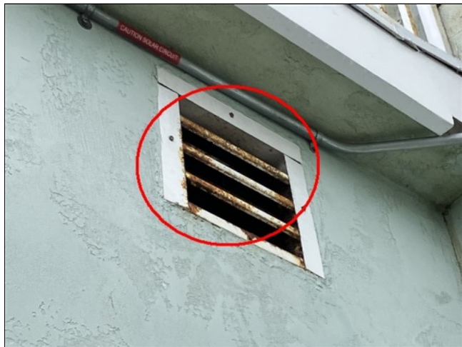
9.2 Item 1(Picture) deterioration/oxidation visible at vent screens
