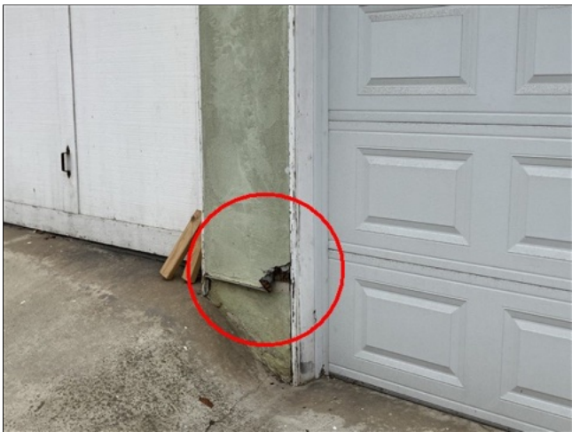
2.0 Item 1(Picture) stucco damage/defect visible // maintenance/repairs needed
