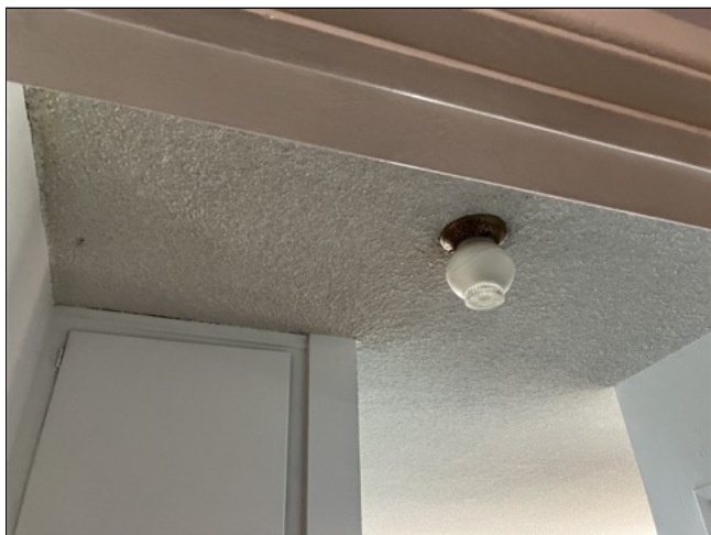
7.7 Item 3(Picture) unit 4768 hallway: missing smoke and CO detector
