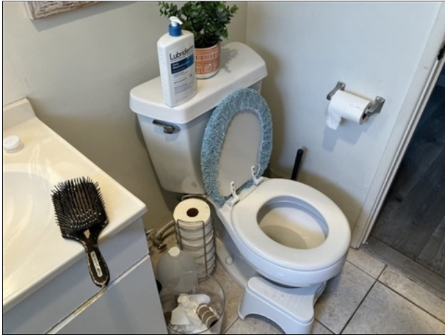
6.5 Item 1(Picture) unit 4772: loose toilet / flushing mechanism did not operate properly when tested / toilet did not appear to be 1.6 gpf
