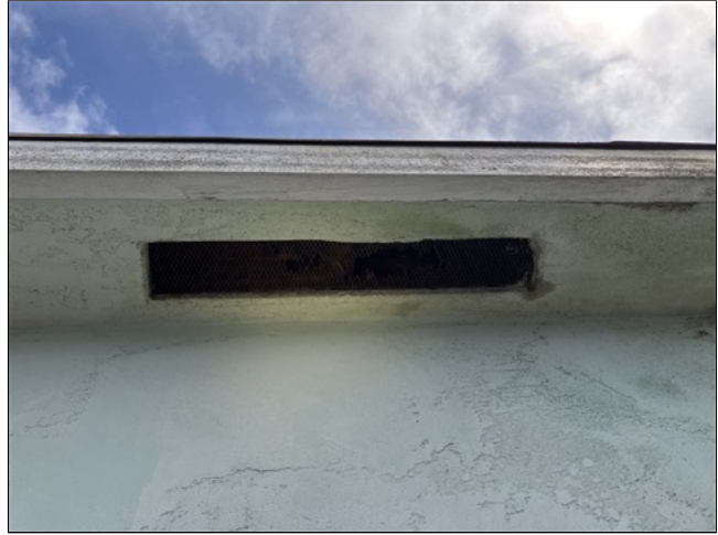
9.2 Item 4(Picture) deterioration/oxidation visible at vent screens
