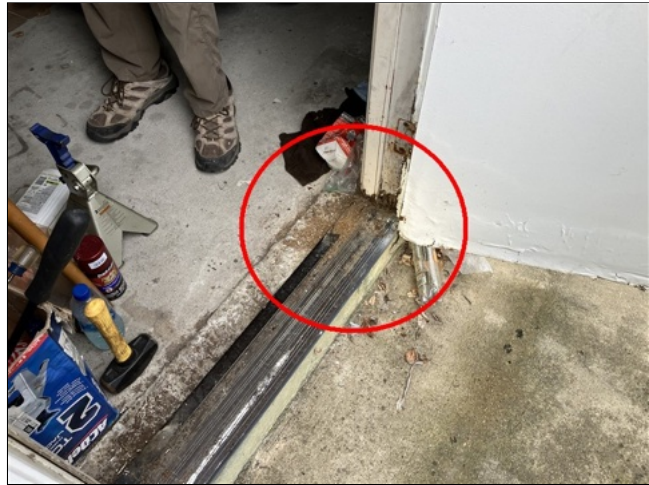
2.1 Item 2(Picture) garage occupant door: possible WDO evidence or damage observed
