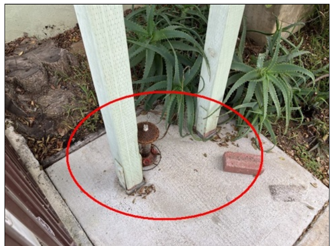
2.3 Item 10(Picture) substandard deck stair support installation observed
