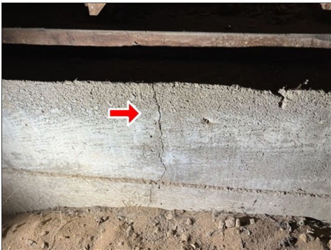
5.0 Item 2(Picture) crack visible at foundation stem wall
