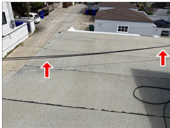
1.7 Item 1(Picture) tripping hazard
