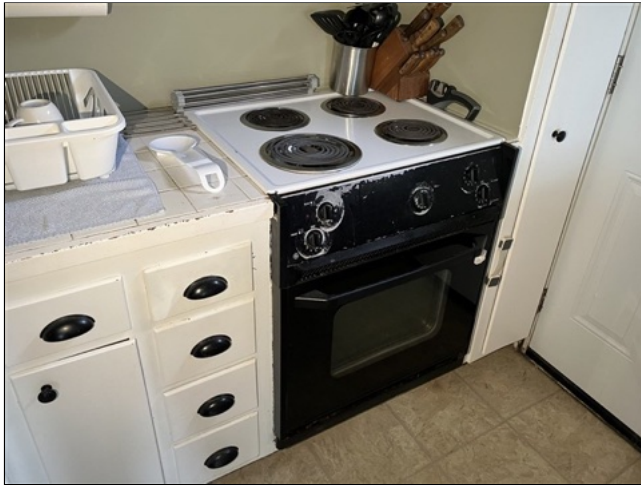
10.7 Item 1(Picture) unit 4768: aged range oven
