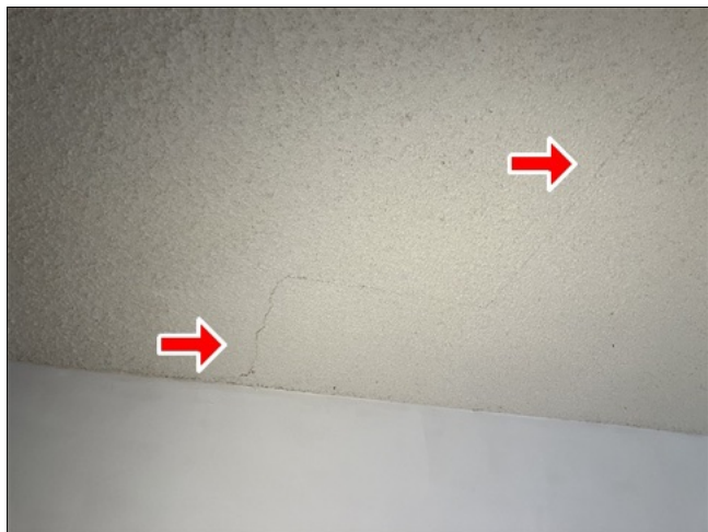
4.0 Item 1(Picture) unit 4768: cracks in ceiling observed
