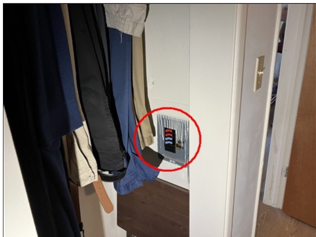
7.2 Item 1(Picture) unit 4768: electrical panel location upgrade recommended
