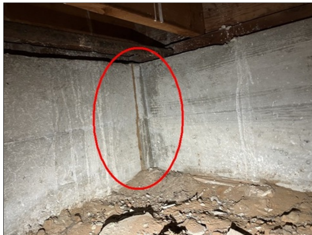
5.2 Item 2(Picture) possible WDO evidence or damage observed
