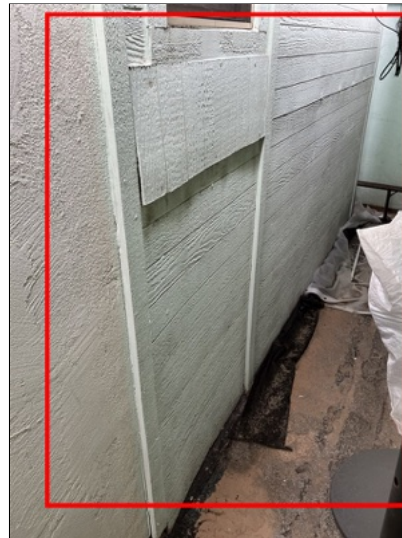
2.0 Item 8(Picture) view from second floor patio: substandard siding installation / recommend further evaluation and correction as needed
