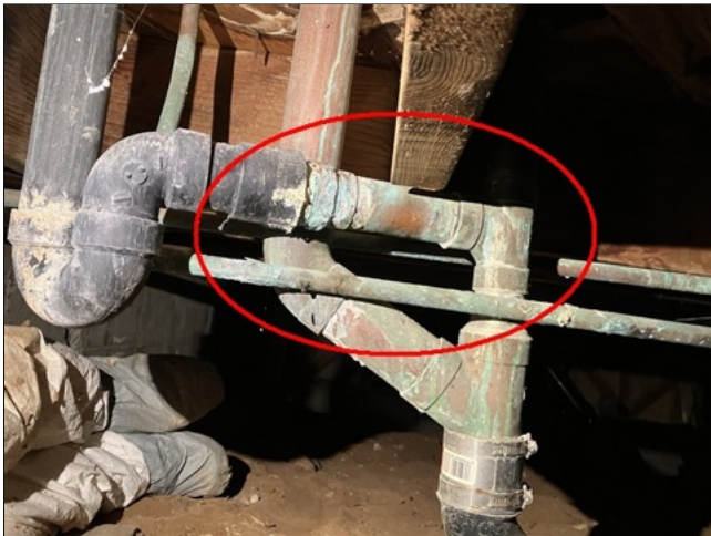
6.3 Item 6(Picture) subfloor area: oxidation visible at copper branch drain
