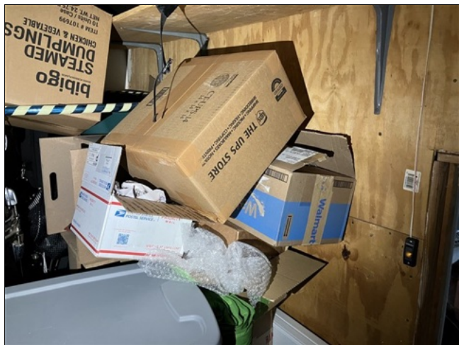
3.1 Item 2(Picture) unit 4770 garage: firewall upgrades recommended
