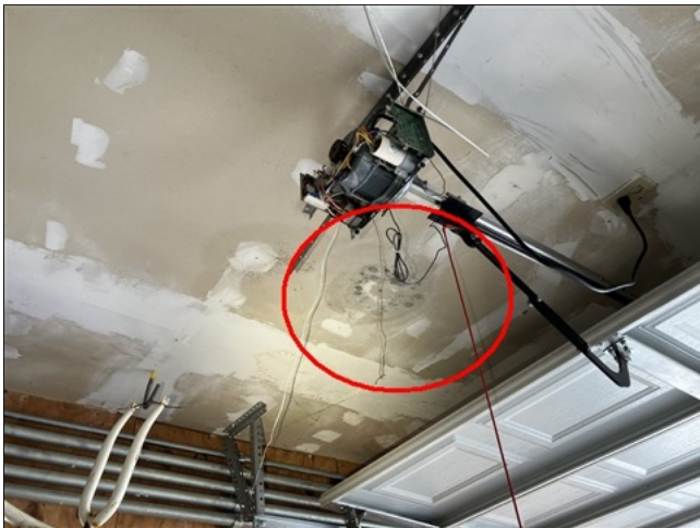
3.2 Item 3(Picture) unit 4772 alley side: moisture stains or damage visible / recommend further evaluation and correction as needed
