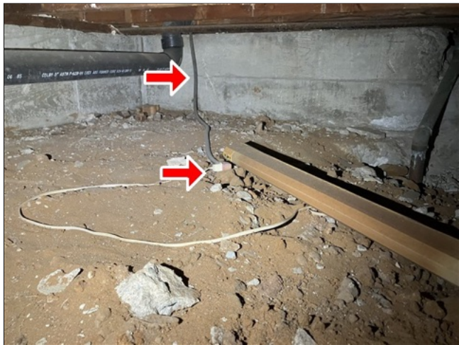
7.8 Item 4(Picture) subfloor area: unidentified extension cord observed / recommend further evaluation
