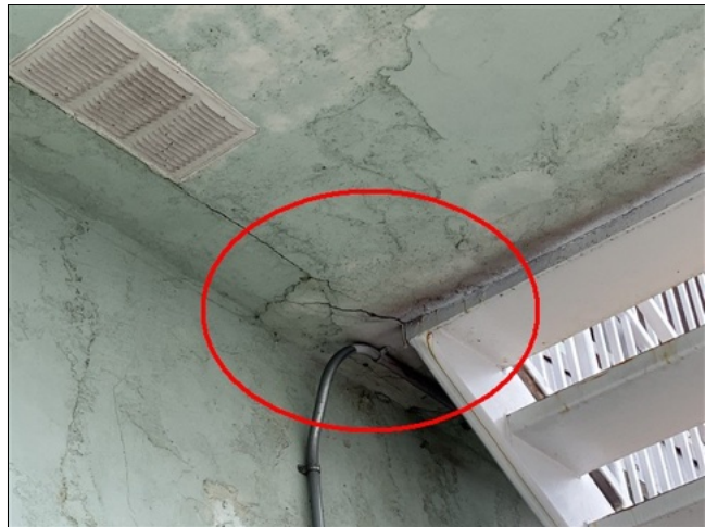
2.3 Item 2(Picture) stucco cracks visible near stair attached to the deck / recommend further evaluation and correction as needed
