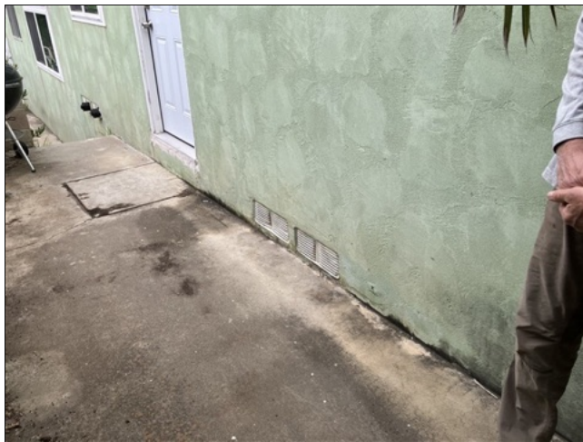
2.4 Item 3(Picture) grading or drainage improvements/ corrections are recommended to achieve positive slope away from the property
