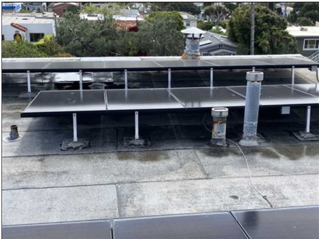
1.0 Item 6(Picture) roll roofing deterioration visible / recommend further evaluation and correction as needed
