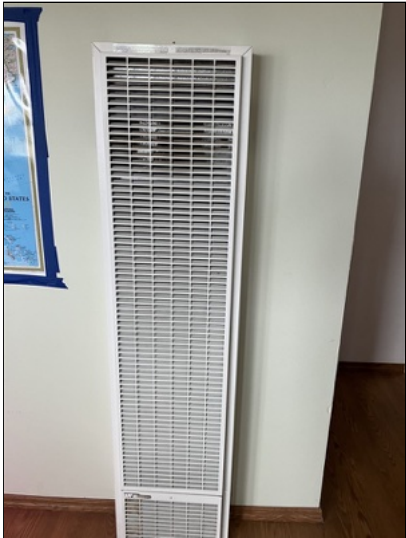
8.2 Item 1(Picture) unit 4768 wall furnace: no visible maintenance record observed
