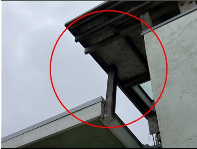
5.7 Item 1(Picture) possible evidence of modifications to original construction observed / substandard installation or building material was observed / recommend further evaluation
