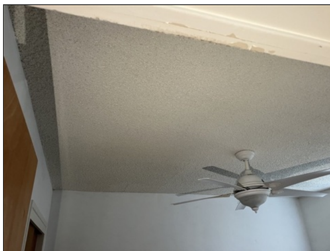
7.7 Item 2(Picture) unit 4768 bedrooms: missing smoke detectors
