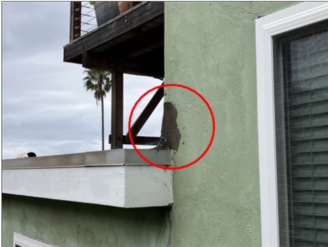
1.2 Item 1(Picture) possible evidence of repairs observed / recommend further evaluation of repair
