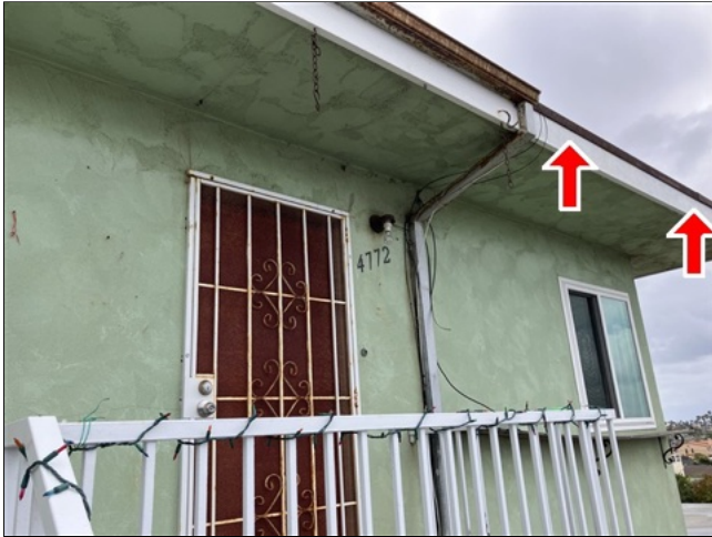
1.2 Item 2(Picture) oxidized flashings observed
