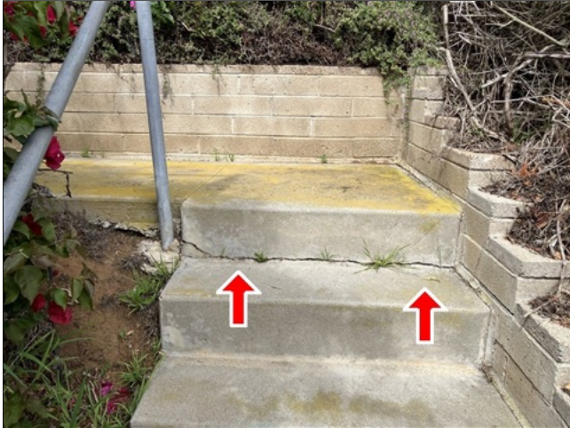
2.4 Item 5(Picture) crack visible at concrete stair
