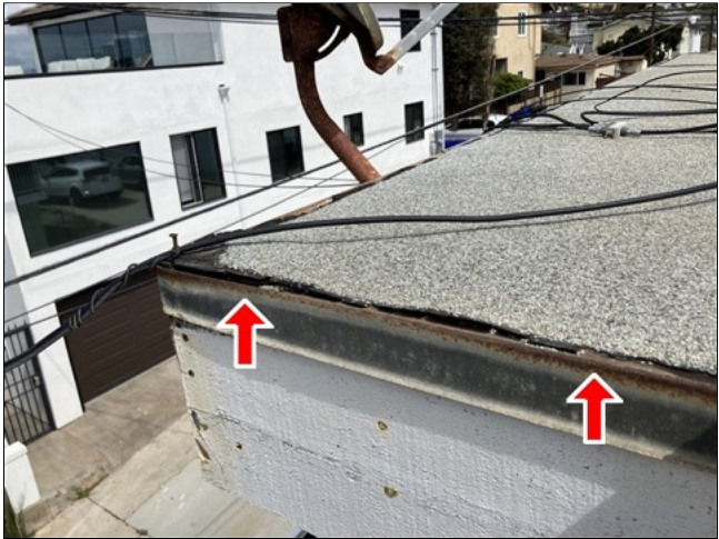
1.0 Item 4(Picture) roll roofing defects observed around the perimeter
