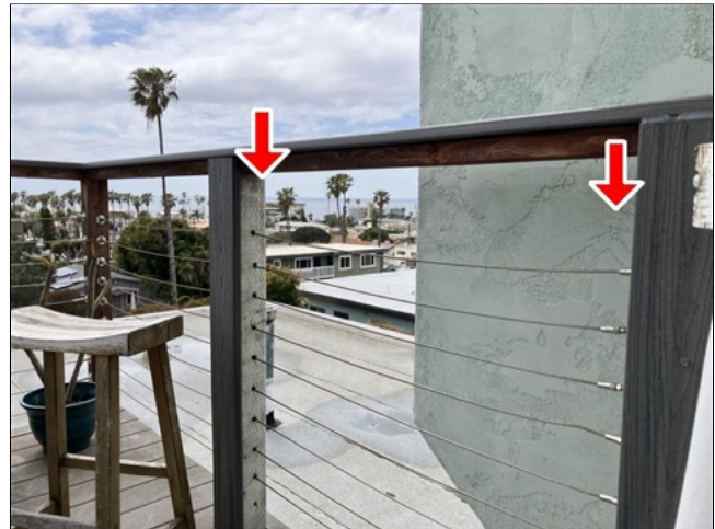
2.3 Item 19(Picture) unit 4772: missing cable railing / loose cable railings
