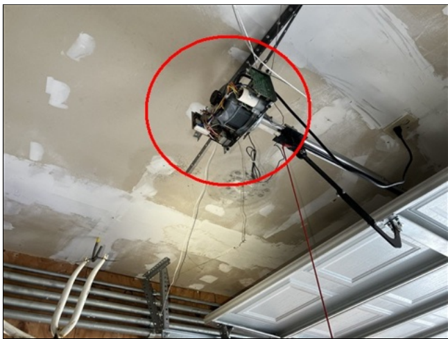
3.5 Item 2(Picture) unit 4772 (alley side): garage door opener cover was missing
