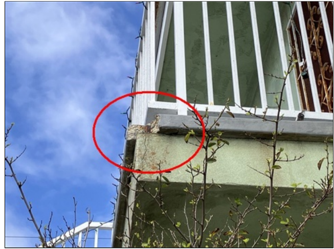
2.3 Item 17(Picture) concrete deck: spalling observed
