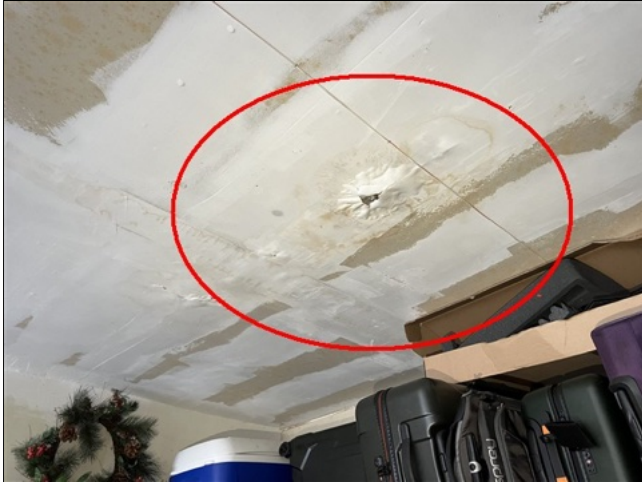
3.2 Item 1(Picture) unit 4770 garage: moisture stains or damage visible / recommend further evaluation and correction as needed
