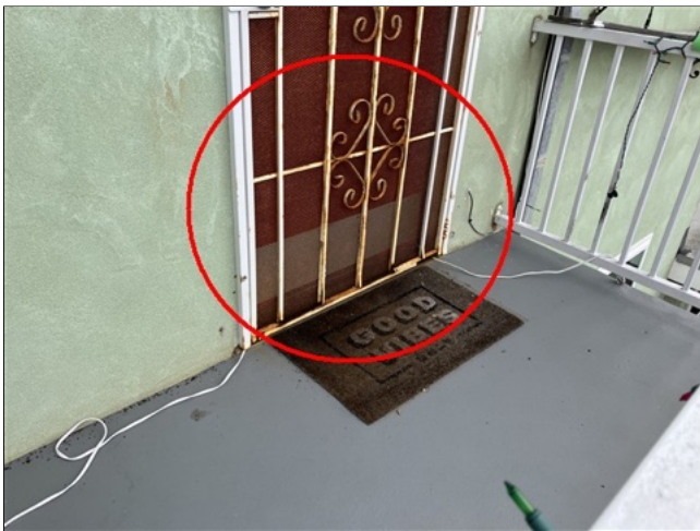
2.1 Item 3(Picture) unit 4772: oxidation visible at security door
