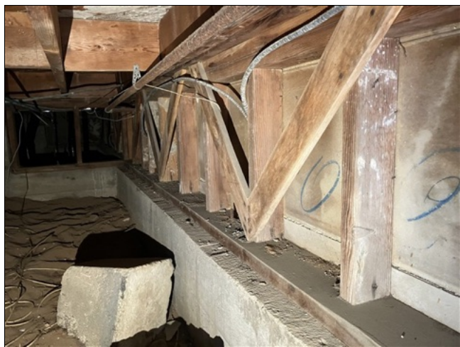
5.3 Item 2(Picture) cripple wall bracing upgrades recommended
