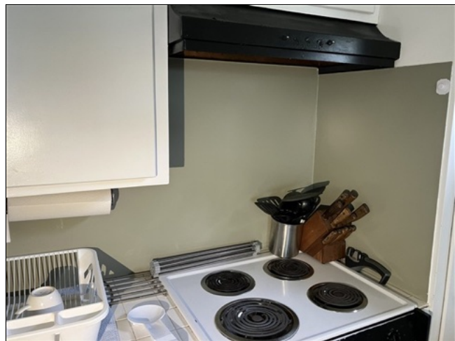
10.1 Item 2(Picture) unit 4768: non-combustible backsplash needed
