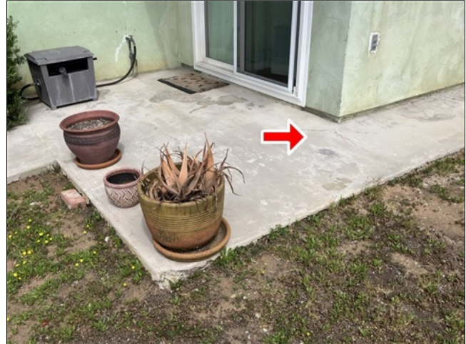
2.4 Item 6(Picture) cracks visible at concrete patio
