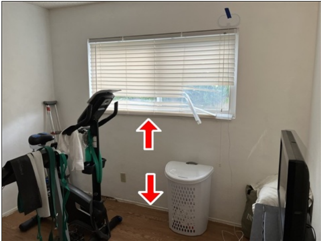
4.5 Item 2(Picture) unit 4768: bedroom window egress upgrades recommended
