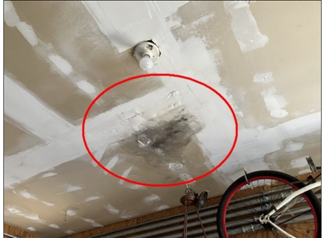
3.2 Item 2(Picture) unit 4772 alley side: moisture stains or damage visible / recommend further evaluation and correction as needed
