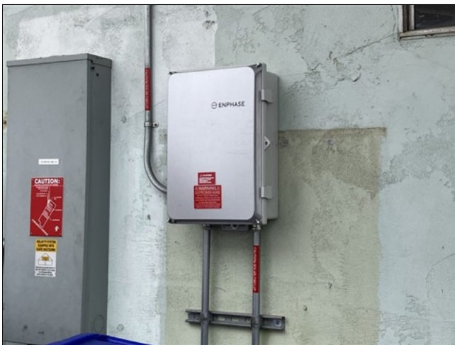
7.8 Item 1(Picture) solar system and components were not inspected or tested as part of the scope of this inspection
