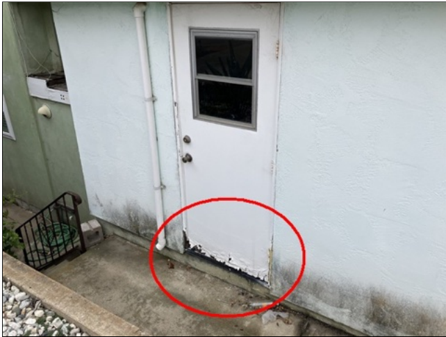
2.1 Item 1(Picture) possible WDO evidence or damage observed / maintenance / repairs / or replacement needed
