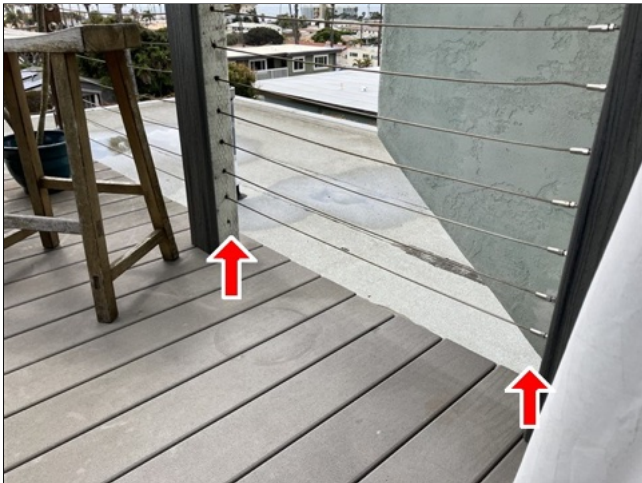
2.3 Item 18(Picture) unit 4772: missing cable railing / loose cable railings
