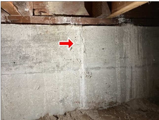
5.0 Item 1(Picture) crack visible at foundation stem wall
