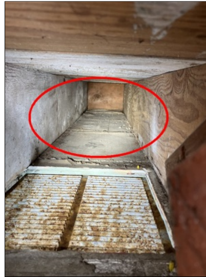
2.3 Item 12(Picture) stairwell storage area: possible WDO evidence or damage observed / moisture stains or damage visible
