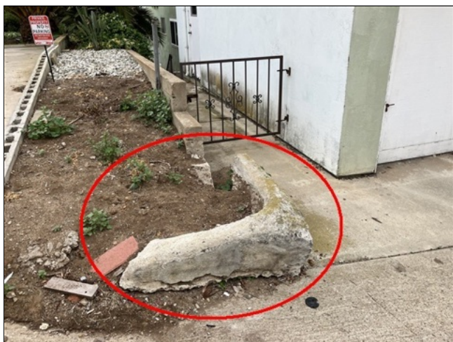
2.6 Item 1(Picture) concrete wall maintenance / repairs / or replacement needed
