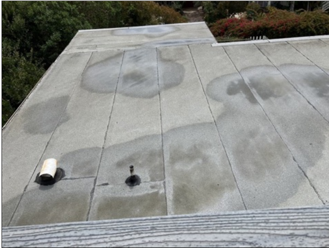
1.1 Item 3(Picture) ponding visible at roof covering / evidence of possible inadequate drainage
