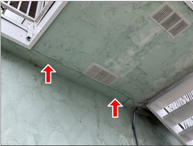
2.0 Item 7(Picture) cracks visible at stucco
