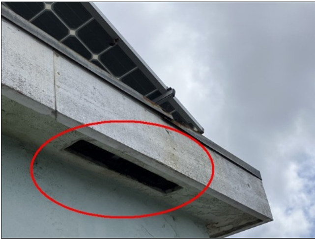
9.2 Item 5(Picture) deterioration/oxidation visible at vent screens
