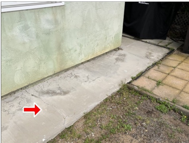
2.4 Item 7(Picture) cracks visible at concrete walkway
