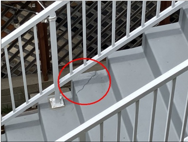
2.3 Item 6(Picture) crack visible at concrete stair
