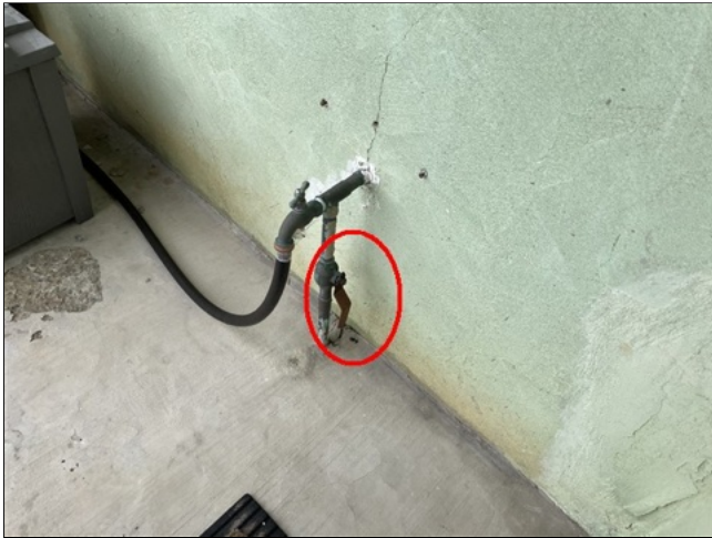
6.1 Item 1(Picture) near unit 4768: water shut off valve for all units
