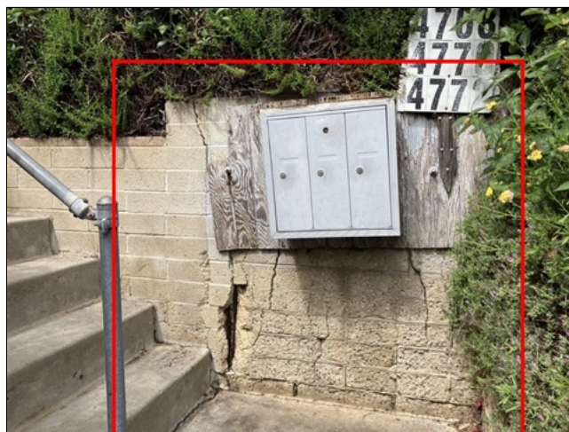
2.6 Item 2(Picture) retaining wall defects observed
