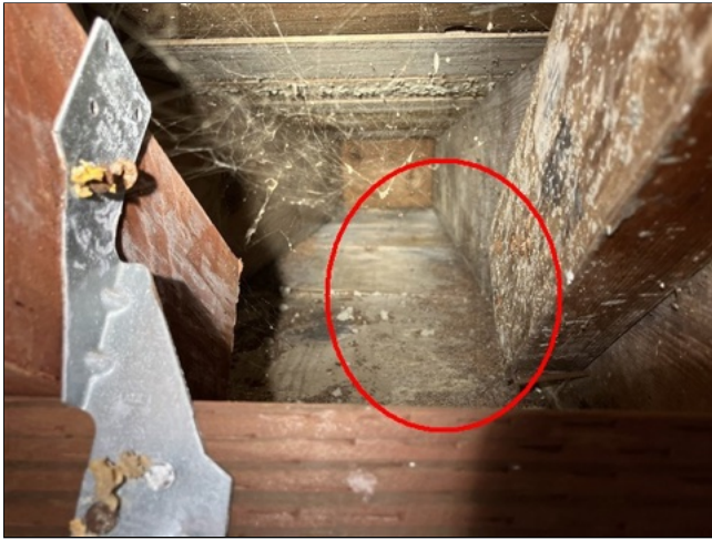
2.3 Item 11(Picture) stairwell storage area: possible WDO evidence or damage observed
