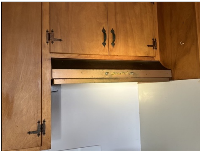
10.7 Item 3(Picture) unit 4772: aged range hood
