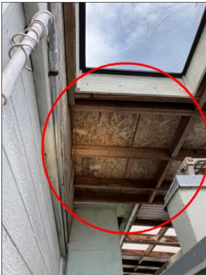
1.0 Item 2(Picture) view from second floor patio: substandard roof covering construction observed / recommend further evaluation and correction as needed
