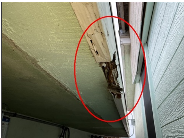
2.5 Item 1(Picture) unit 4772: possible WDO evidence or damage observed
