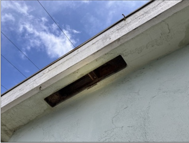
9.2 Item 3(Picture) deterioration/oxidation visible at vent screens
