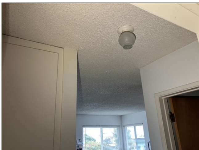
7.7 Item 1(Picture) unit 4768 hallway: missing smoke and CO detector
