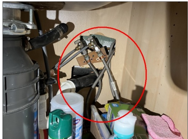
6.4 Item 4(Picture) unit 4772 (alley side): double-hoses observed
