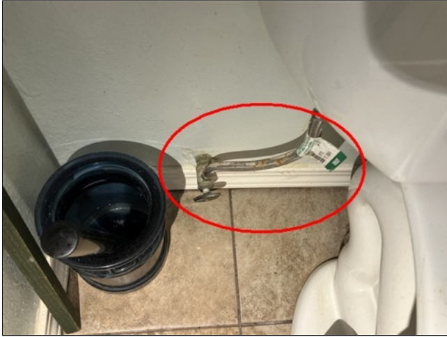
6.4 Item 5(Picture) unit 4772 (alley side): oxidation visible at valve/hose
