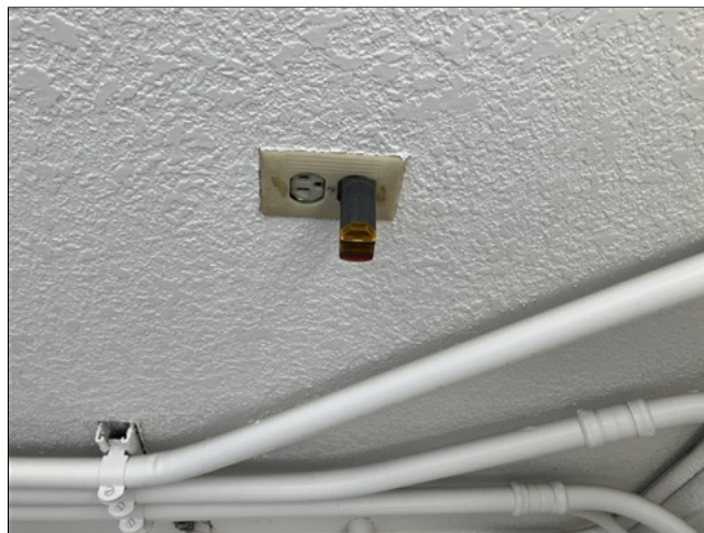
7.5 Item 4(Picture) laundry room: no power at outlet
