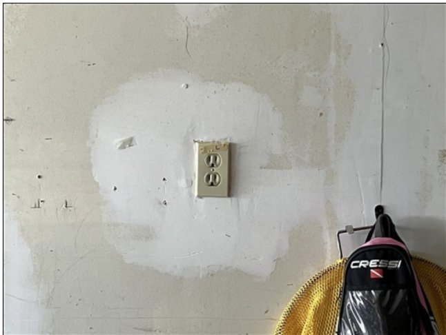
7.6 Item 2(Picture) unit 4770 garage: recommend evaluation and upgrade of any non-GFCI outlets
