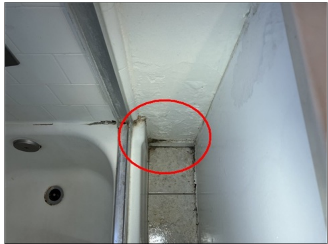
4.6 Item 3(Picture) unit 4772: moisture stains or damage visible
