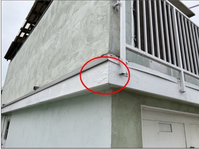
2.3 Item 3(Picture) possible WDO evidence or damage observed
