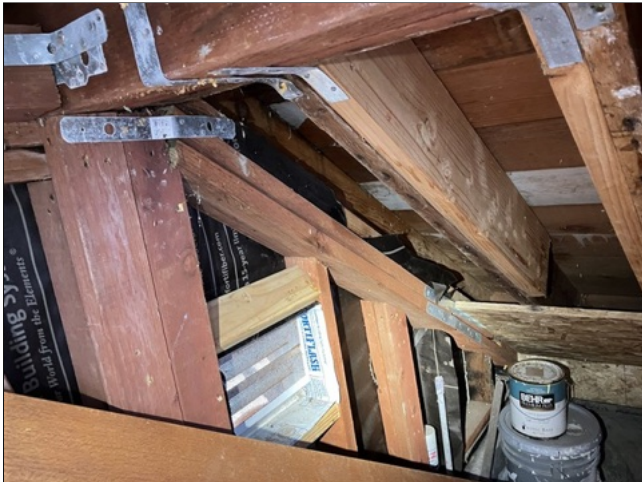
2.3 Item 13(Picture) stairwell storage area: possible evidence of substandard repairs observed / recommend further evaluation of repair
