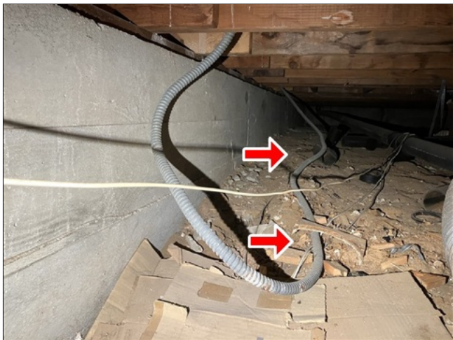
7.4 Item 2(Picture) subfloor area: conduit should be secured to the framing and off of the ground
