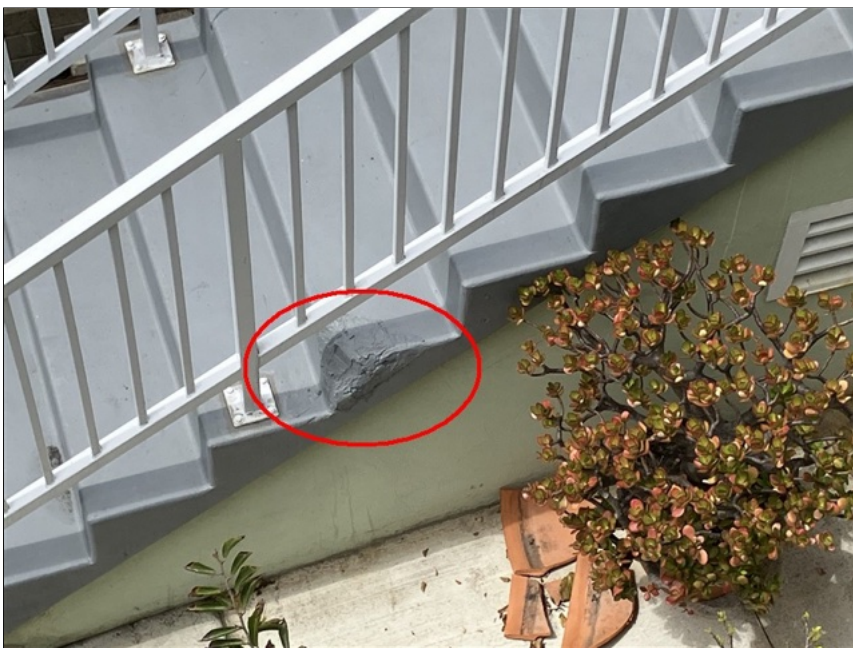
2.3 Item 5(Picture) possible evidence of repairs observed / recommend further evaluation of repair
