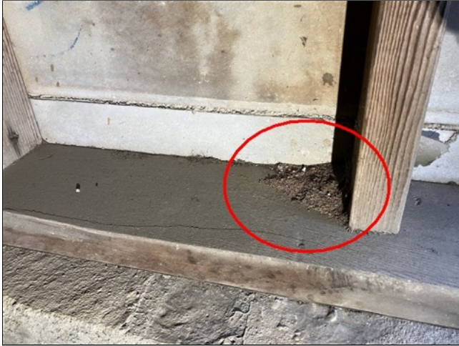
5.3 Item 4(Picture) subfloor area: possible WDO evidence or damage observed
