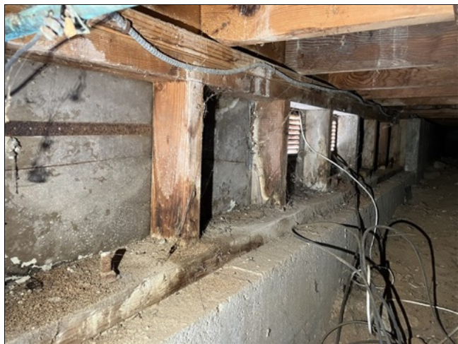
5.3 Item 3(Picture) cripple wall bracing upgrades recommended
