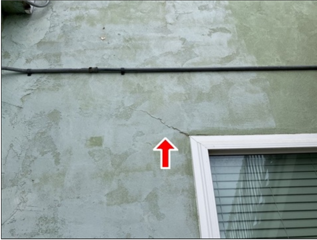
2.0 Item 5(Picture) cracks visible at stucco
