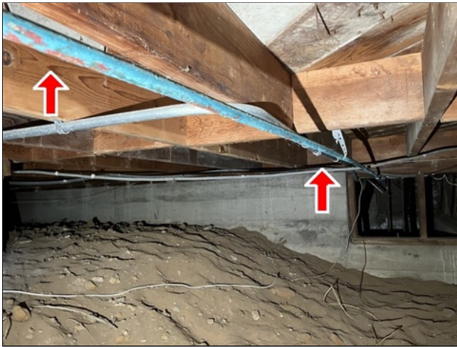
6.4 Item 7(Picture) subfloor area: oxidation visible at water supply pipe
