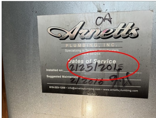
6.0 Item 3(Picture) installed 2015
