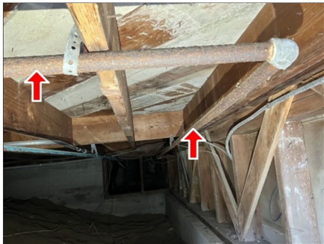
6.6 Item 1(Picture) subfloor area: oxidation visible at gas supply
