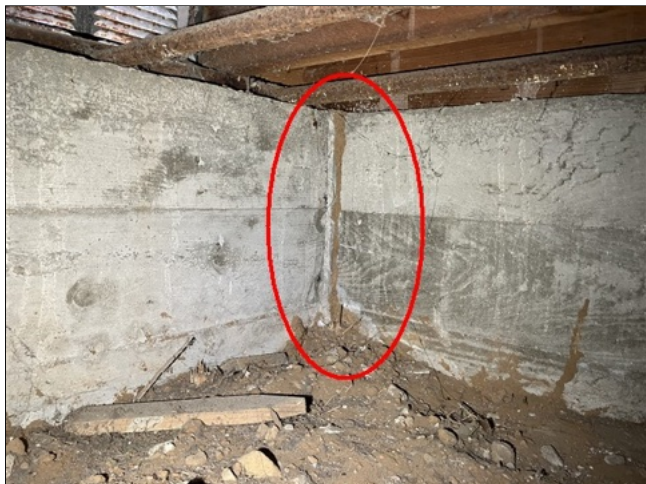
5.2 Item 1(Picture) possible WDO evidence or damage observed
