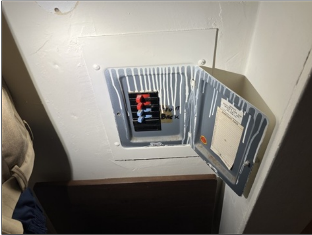
7.3 Item 1(Picture) unit 4768: a Zinsco panel performance and safety inspection by a qualified person is recommended
