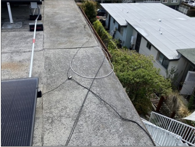
1.0 Item 8(Picture) roll roofing deterioration visible / recommend further evaluation and correction as needed
