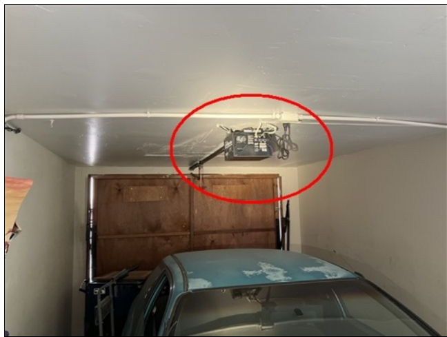
3.5 Item 1(Picture) garage door operator did not operate properly when tested
