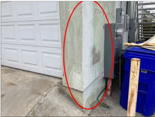
2.0 Item 3(Picture) stucco surface and paint maintenance/repairs needed
