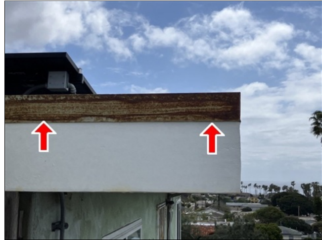
1.2 Item 3(Picture) oxidized flashings observed
