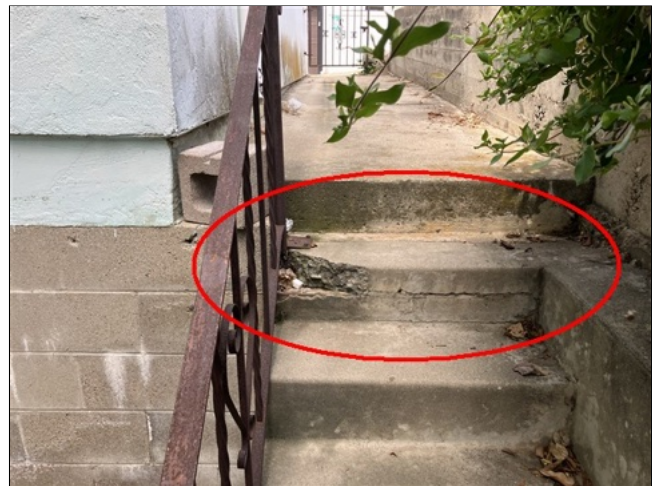
2.4 Item 8(Picture) concrete spalling at stairs observed
