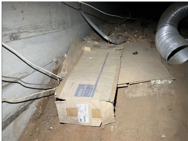
5.7 Item 4(Picture) subfloor area: debris removal needed
