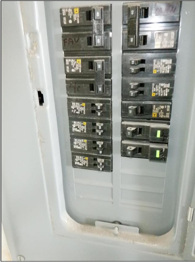
8.0 Item 3(Picture) Circuit breakers
