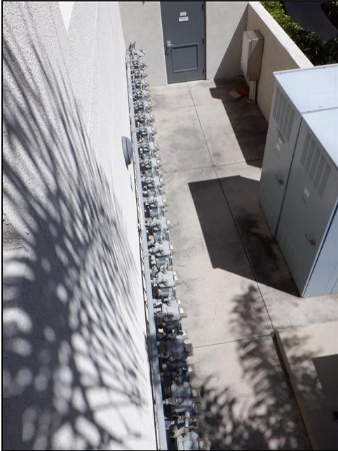
7.3 Item 1(Picture) Gas meters and shut off
