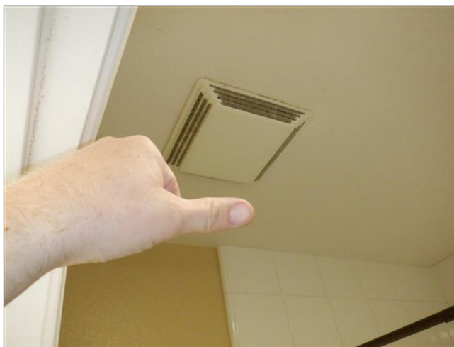
5.8 Item 2(Picture) Loud exhaust fan
