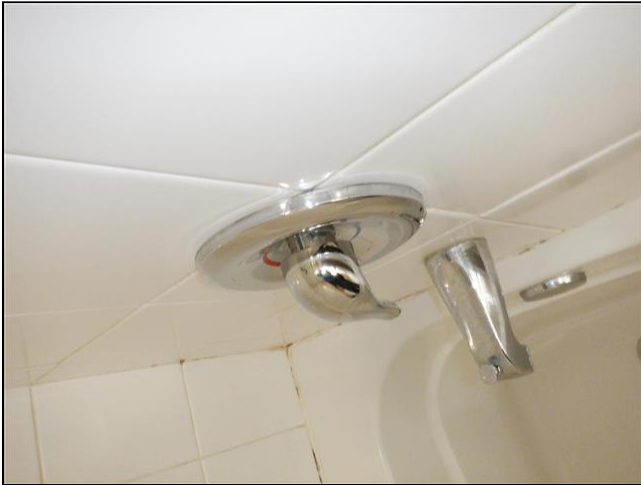
5.6 Item 9(Picture) Fixtures not sealed
