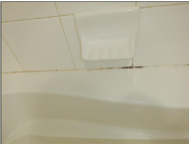
5.6 Item 7(Picture) Worn caulking
