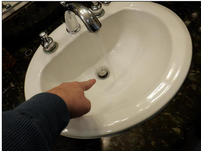
5.5 Item 8(Picture) Foul smell from top floor bathrooms sinks
