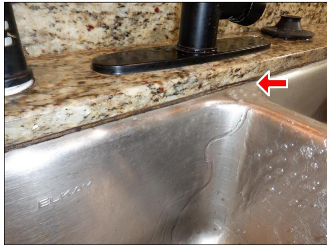
3.5 Item 2(Picture) Sink not sealed
