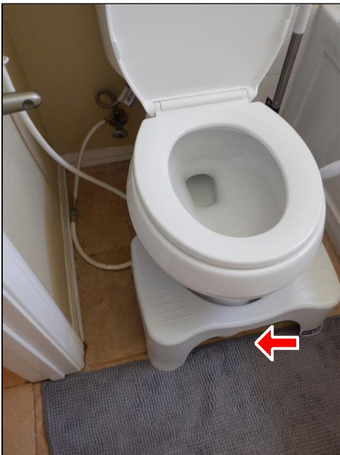
5.6 Item 13(Picture) Loose toilet
