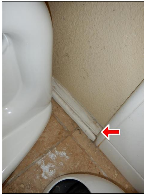
5.2 Item 2(Picture) Damaged baseboards behind top floor toilet
