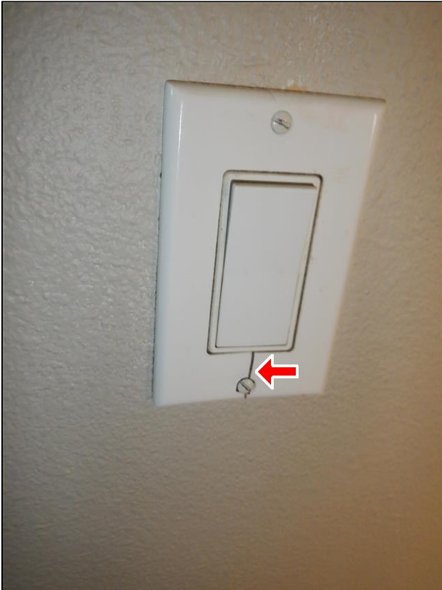
4.6 Item 1(Picture) Cracked cover plate in hallway
