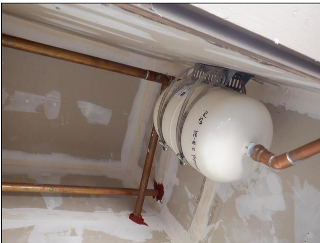
7.0 Item 3(Picture) Expansion tank
