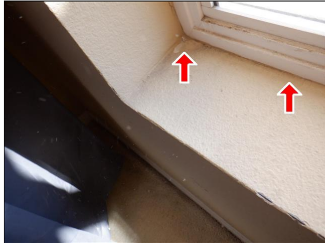
4.5 Item 2(Picture) Cracking in window sills
