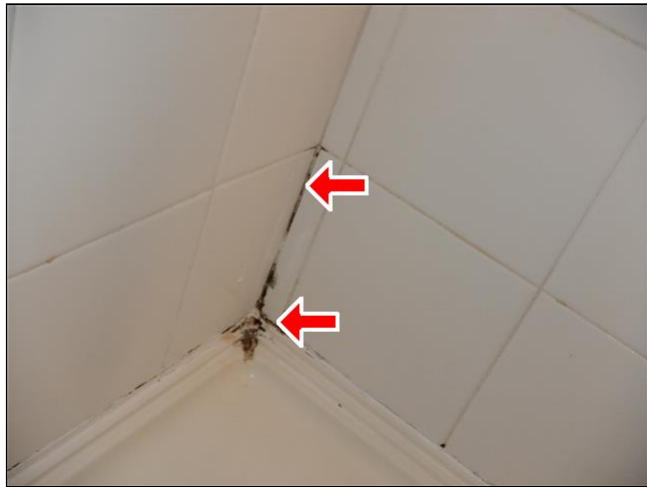
5.6 Item 20(Picture) Worn caulking in shower
