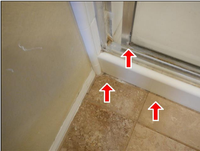
5.6 Item 11(Picture) Shower door not sealed
