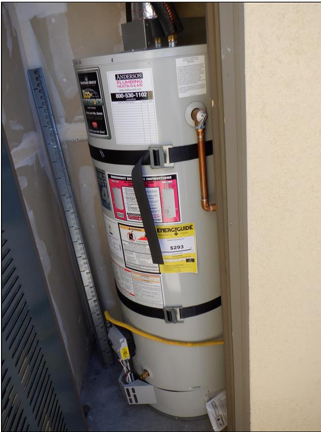
7.0 Item 1(Picture) Water heater
