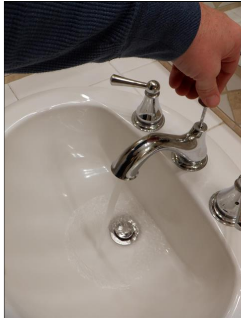
5.5 Item 2(Picture) Top floor bathroom sink stopper not attached
