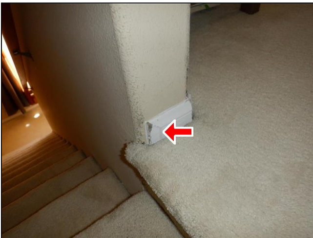
4.2 Item 1(Picture) Damaged baseboards
