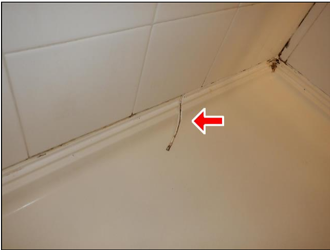
5.6 Item 19(Picture) Loose silicone
