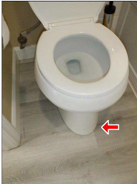
5.6 Item 4(Picture) Loose toilet
