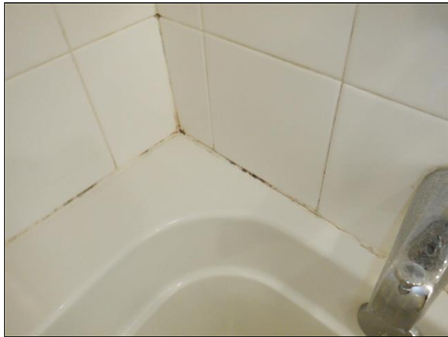
5.6 Item 6(Picture) Worn caulking
