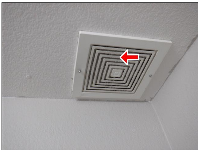
5.8 Item 1(Picture) Dirty exhaust fan
