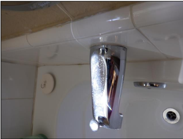
5.6 Item 15(Picture) Fixtures not sealed
