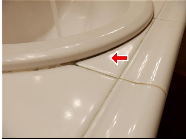
5.6 Item 2(Picture) Sink not sealed
