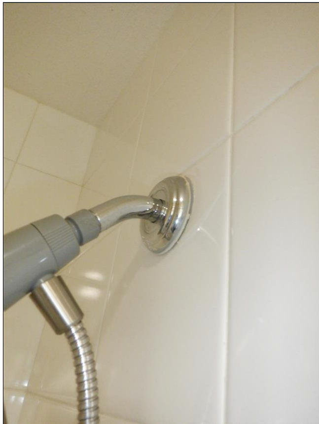
5.6 Item 8(Picture) Fixtures not sealed
