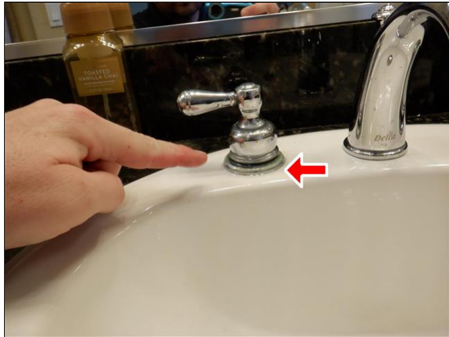
5.6 Item 12(Picture) Faucet leaks
