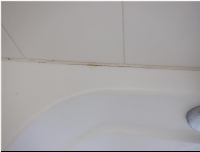
5.6 Item 17(Picture) Worn caulking
