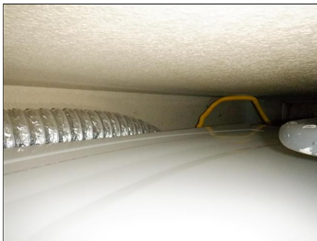
3.12 Item 4(Picture) Gas connection for dryer
