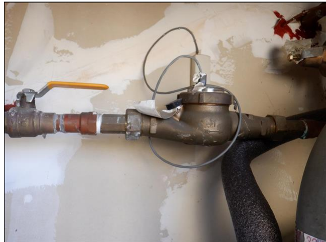
7.0 Item 6(Picture) Water lines
