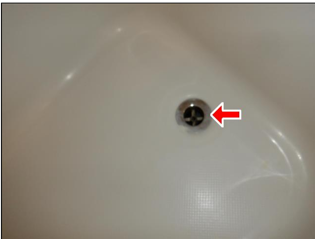
5.5 Item 5(Picture) Missing tub stopper
