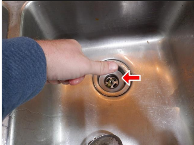
3.4 Item 2(Picture) Sink drains slowly
