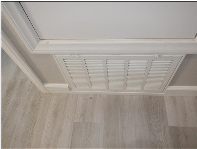
9.0 Item 3(Picture) Intake filter
