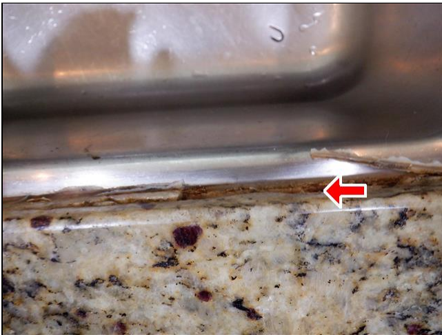
3.5 Item 3(Picture) Worn caulking on sink
