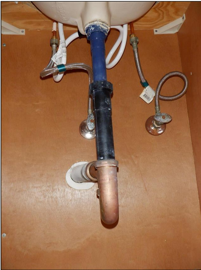
5.5 Item 3(Picture) Bathroom sink plumbing
