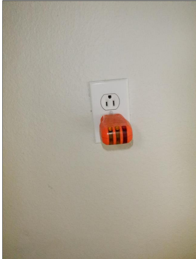
4.6 Item 2(Picture) Upside down receptacles
