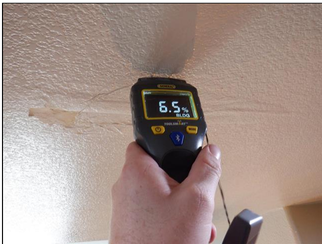
3.0 Item 3(Picture) Moisture test at repair in kitchen ceiling
