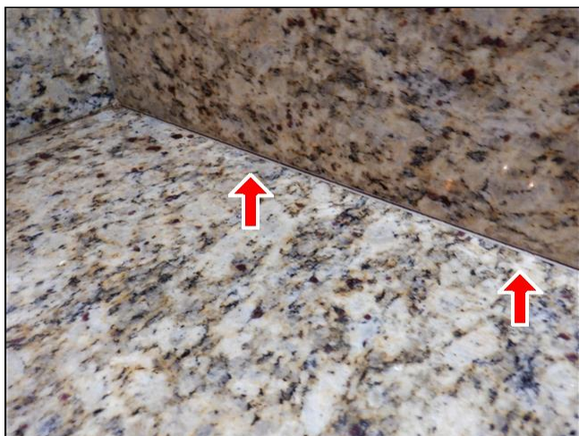
3.3 Item 1(Picture) Worn grout
