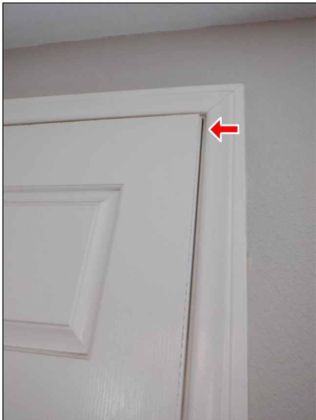
2.1 Item 1(Picture) Front door rubs door frame
