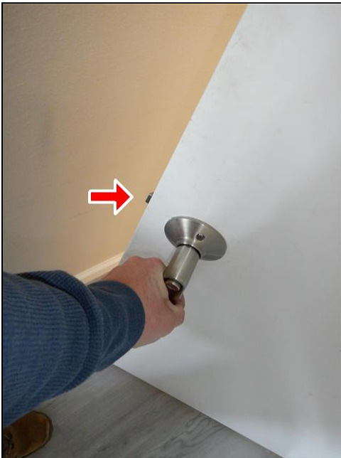
4.4 Item 1(Picture) Stairway door latch does not fully disengage
