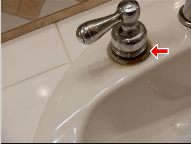
5.6 Item 1(Picture) Faucet leaks / corrosion
