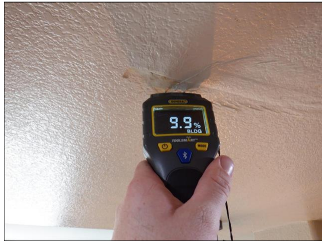
3.0 Item 2(Picture) Moisture test at repair in kitchen ceiling
