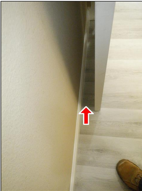
5.3 Item 1(Picture) Missing door stop
