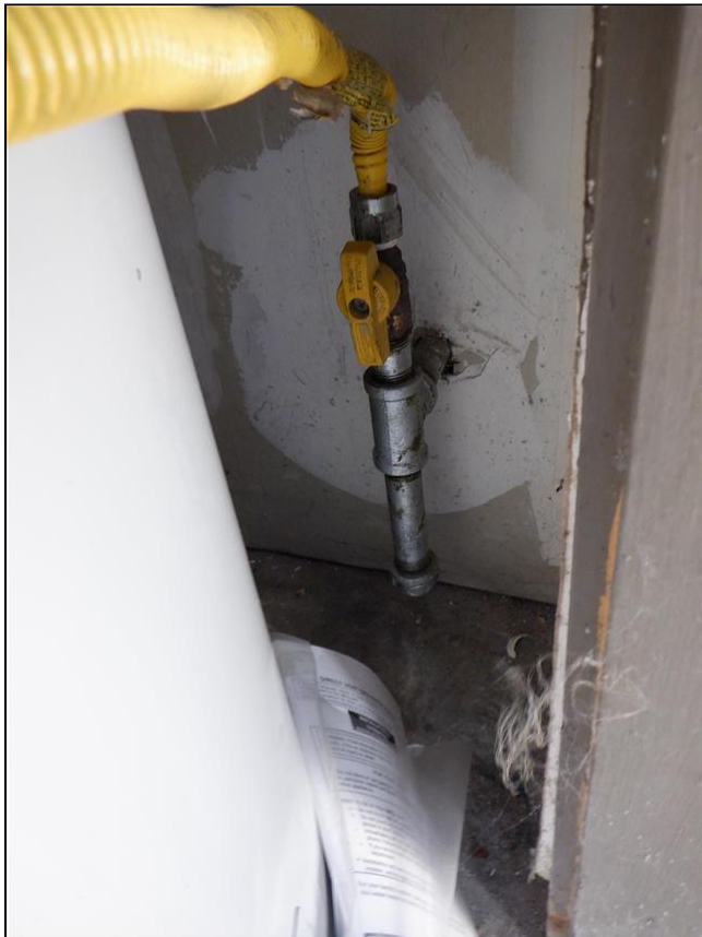
7.0 Item 5(Picture) Sediment trap
