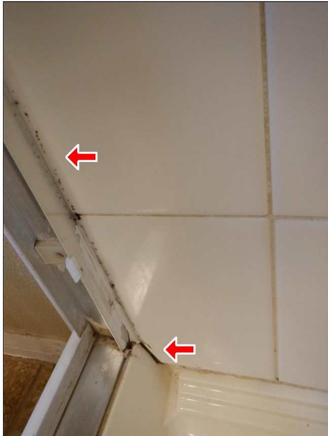
5.6 Item 18(Picture) Worn / missing caulking
