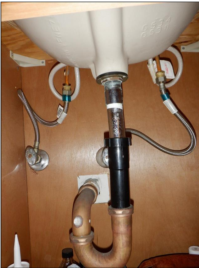
5.5 Item 9(Picture) Sink plumbing
