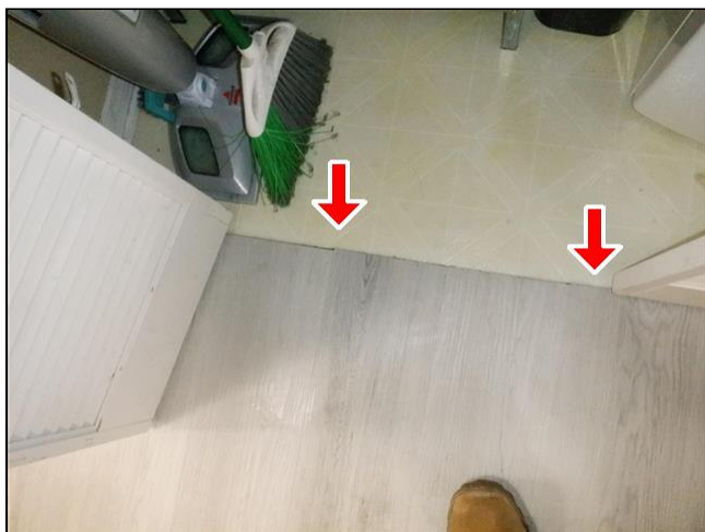
3.12 Item 5(Picture) Missing transition
