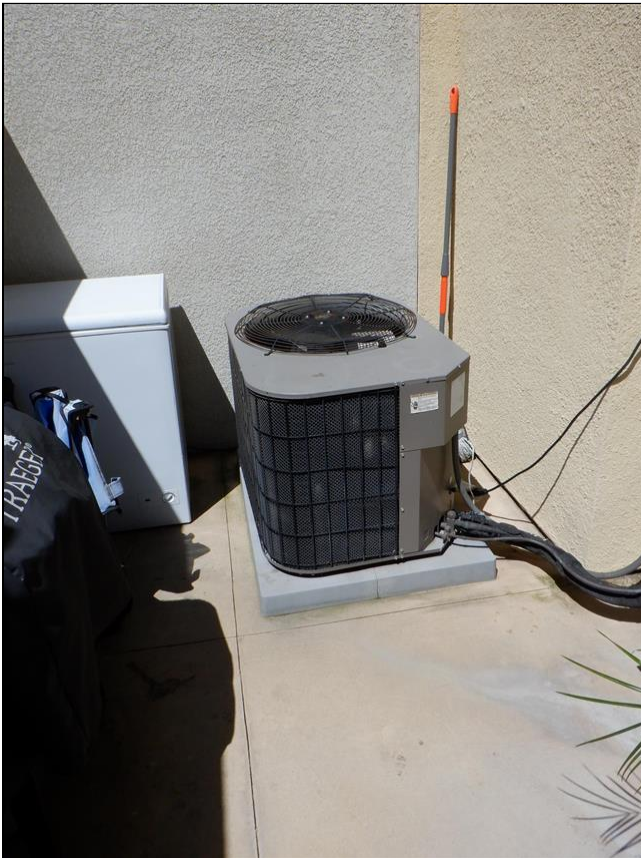
9.5 Item 1(Picture) Condenser
