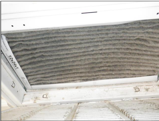
9.3 Item 1(Picture) Filter needs replacement
