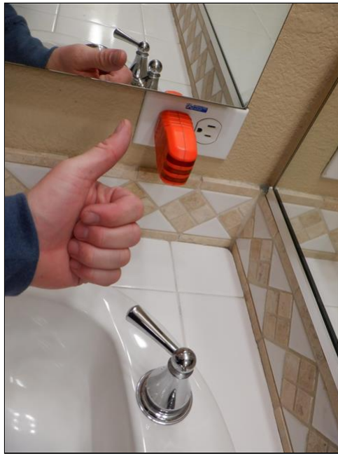
5.7 Item 2(Picture) GFCI protected
