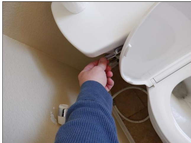
5.6 Item 14(Picture) Loose toilet handle
