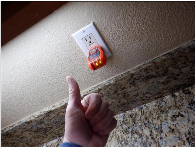
3.6 Item 1(Picture) Good GFCI
