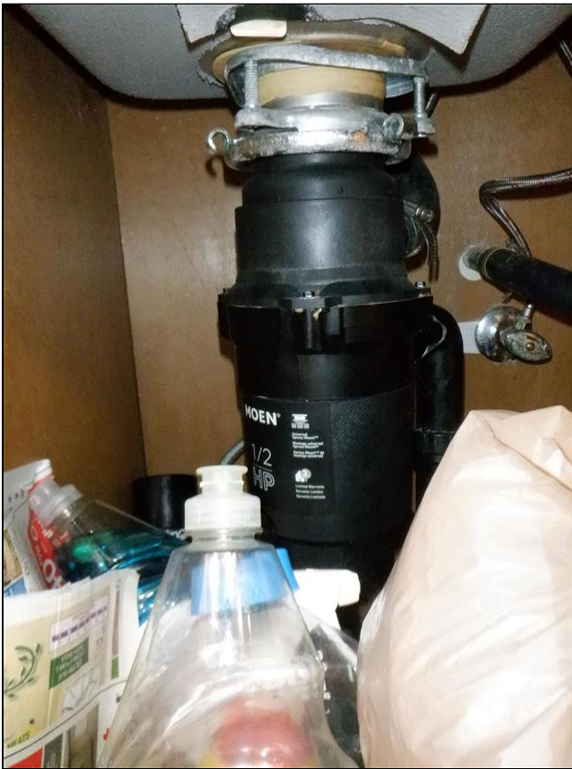
3.10 Item 1(Picture) Garbage disposal
