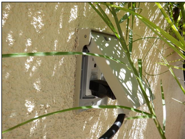
2.6 Item 1(Picture) Good GFCI
