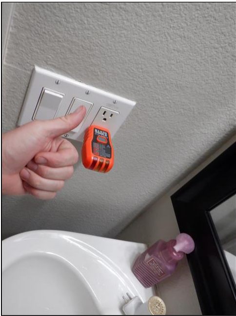
5.7 Item 1(Picture) GFCI protected
