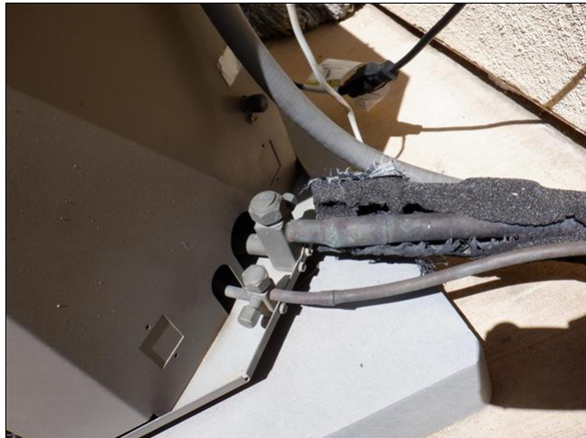
9.5 Item 2(Picture) Worn insulation
