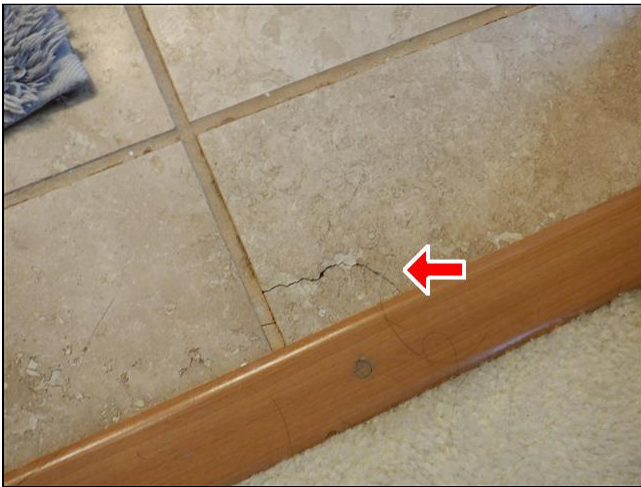
5.2 Item 1(Picture) Cracked tile in top floor bathroom
