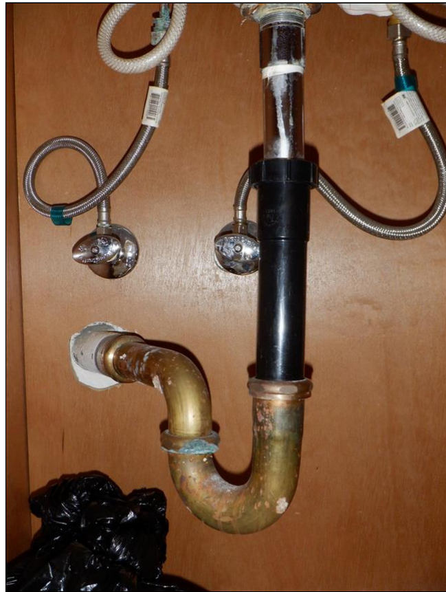
5.5 Item 4(Picture) Bathroom sink plumbing
