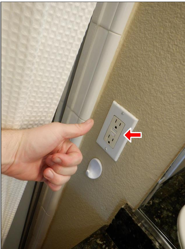
5.7 Item 3(Picture) Master GFCI for all bathrooms
