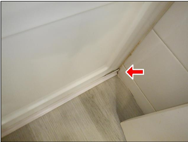
5.6 Item 5(Picture) Loose trim at base of tub
