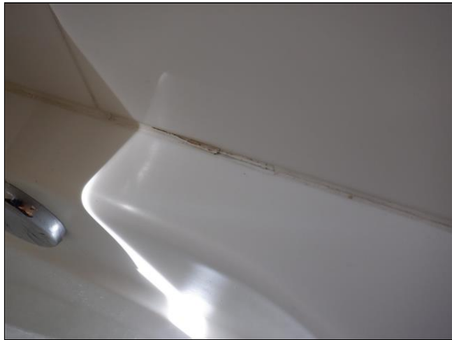
5.6 Item 16(Picture) Worn caulking
