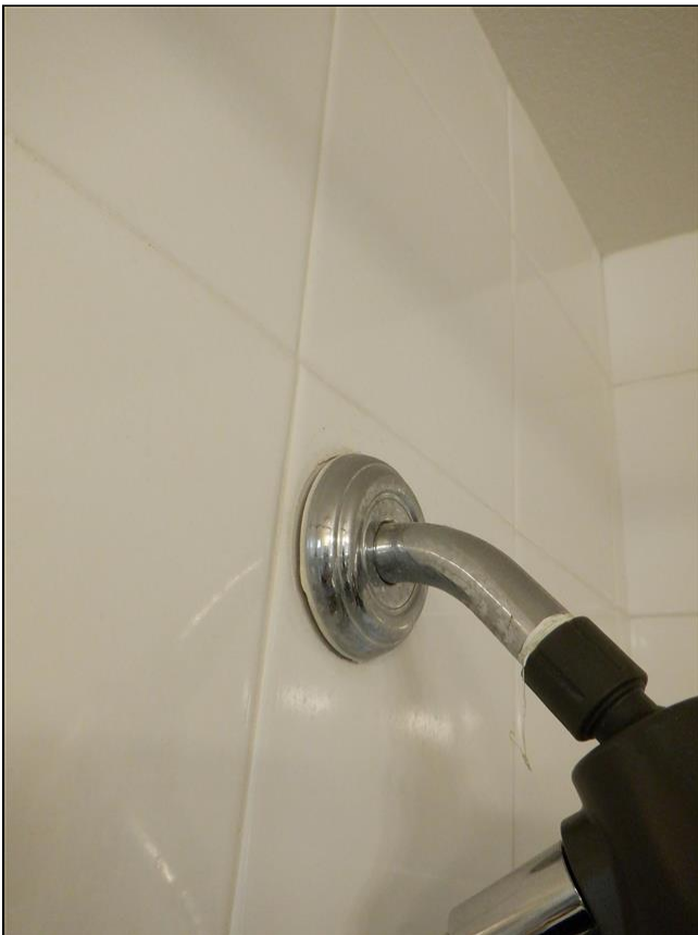
5.6 Item 21(Picture) Showerhead not sealed
