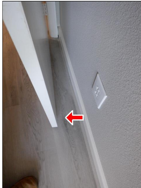
4.4 Item 2(Picture) Missing door stops
