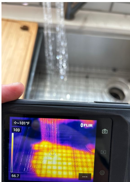
Thermal image(s) showing the water heater(s) producing hot water at the time of the inspection.
