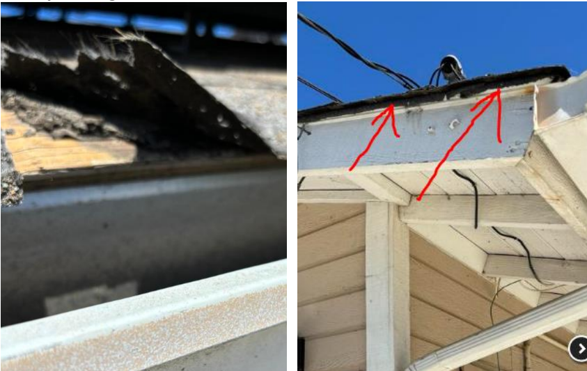
Examples of missing edge metal
