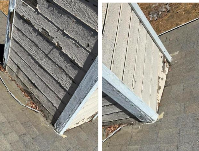
Examples of improper flashing at chimney
