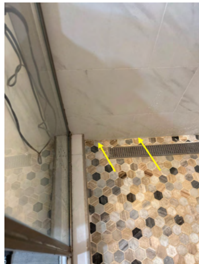
The floor of the shower is in need of additional grout and or sealant at the floor to wall intersection. Location: Bathroom 3.
