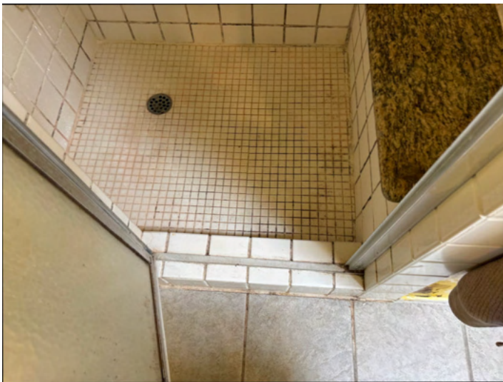
The shower wall grout, tile and shower base are in need of cleaning. Location: Masterbathroom.
