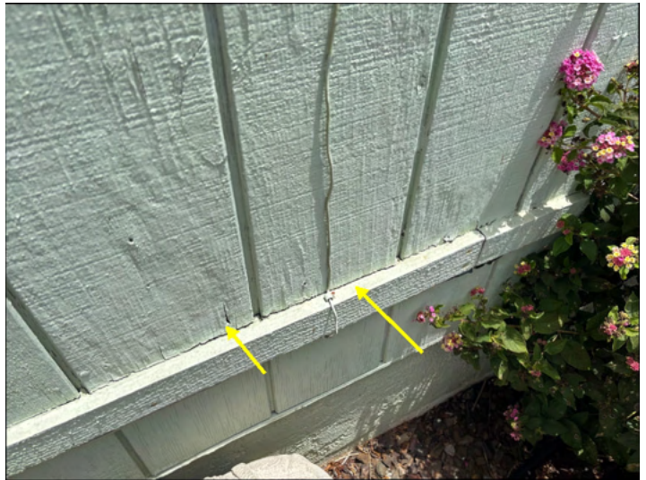
There is wood siding on the right side of the home. This siding shows signs of insect and or water damage. This condition should be noted and may require future maintenance. Please review the termite report regarding this condition as Home Inspections San Diego doesn't perform any insect and or water damage inspections.
