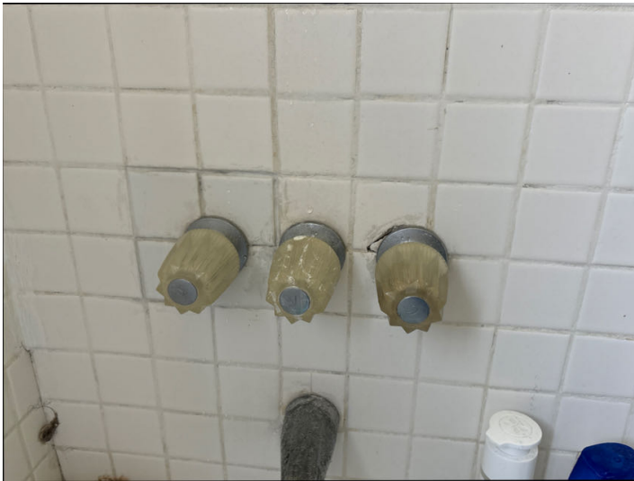
The shower wall is in need of additional grout and or sealant at the bathtub intersection as the current seal is worn. Location: Bathroom 2.
