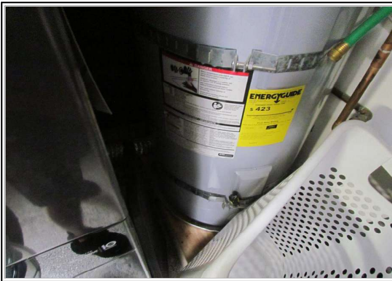
WATER HEATER DOUBLE STRAPPED
