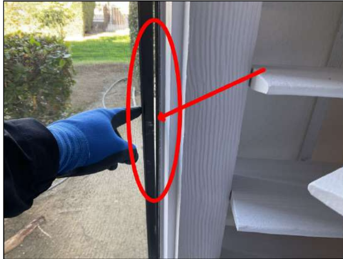
Window screen bent/damaged. Recommend Repair/Replace. Location: Bedroom
