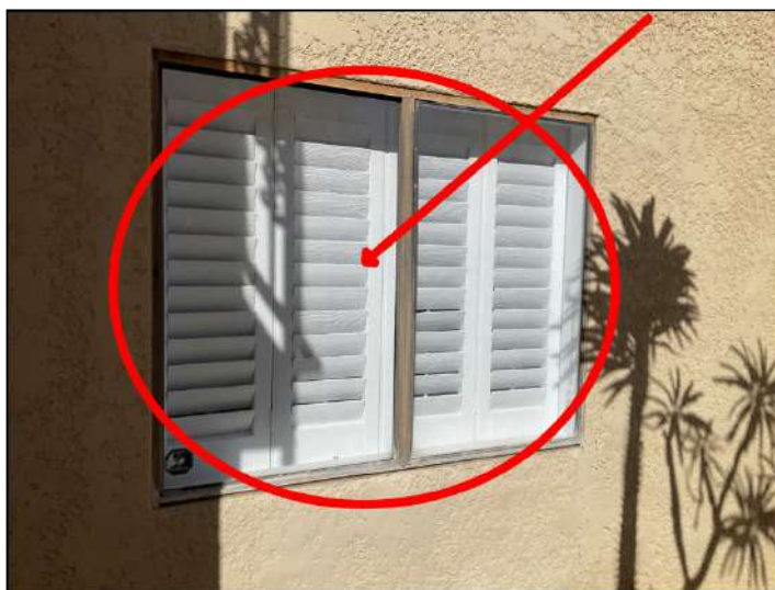
Missing window screen(s). Location: Dining room
