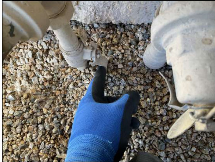
Main water shut of valve.
