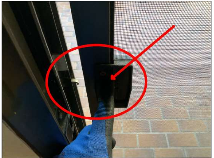
Missing screen door locking mechanism. Recommend licensed technician Repair/Replace.
