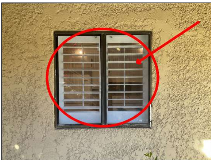
Missing window screen(s). Location: Kitchen
