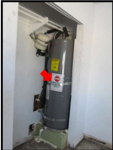
Improper Strapping noted.
