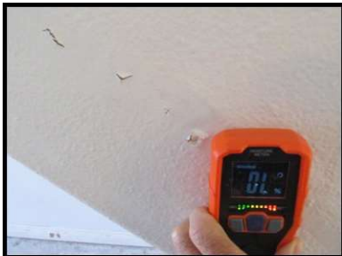
Wet Staircase drywall noted.
