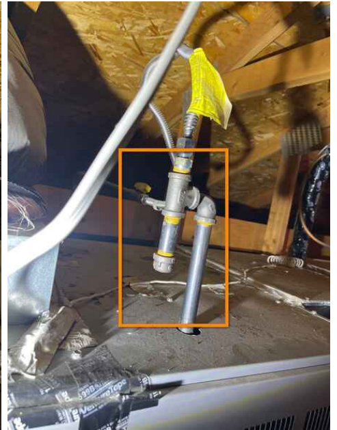
Here is the second furnace that has the sediment trap.
