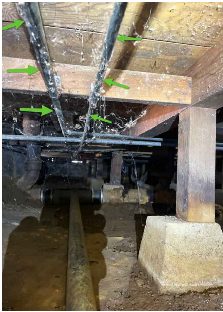
This house had the original galvanized iron water pipes which appeared to be in good condition
