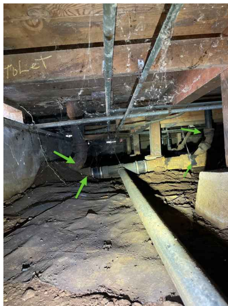
The remaining original cast iron drain lines looked to be in good condition
