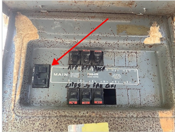
Main electrical shutoff
