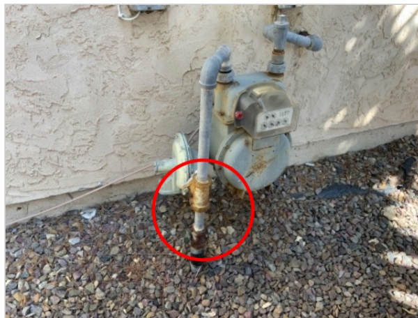
Main gas shutoff
