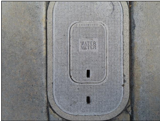
Main water meter.
