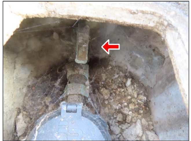
Main water meter.
