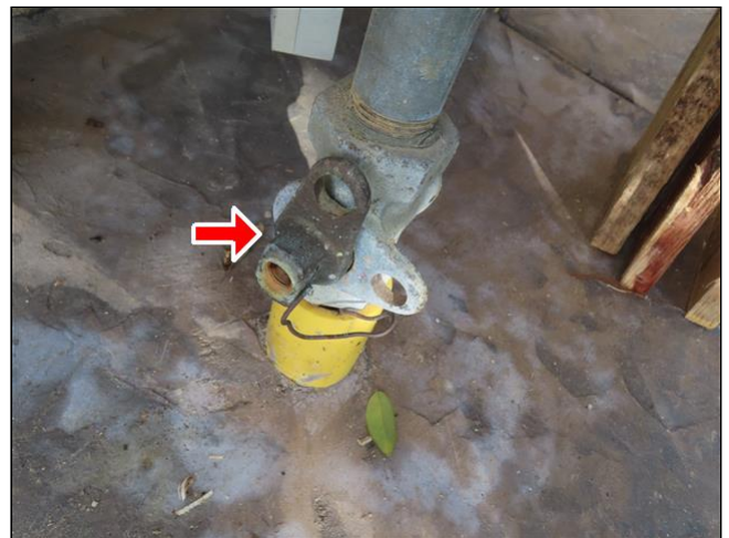
Main gas shut-off.
