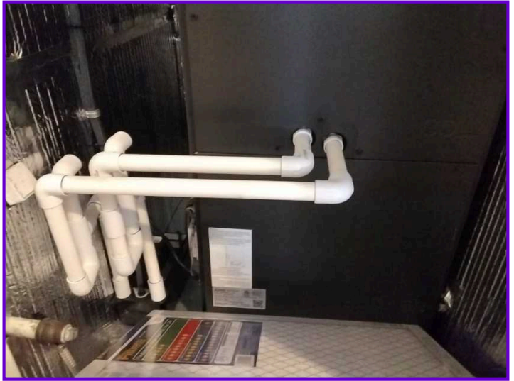
Heat Pump Heat and AC
