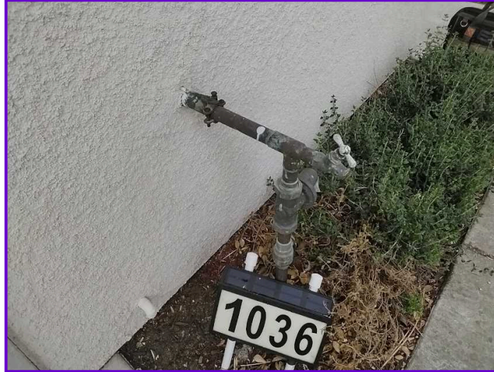
Water Supply System Water Main
