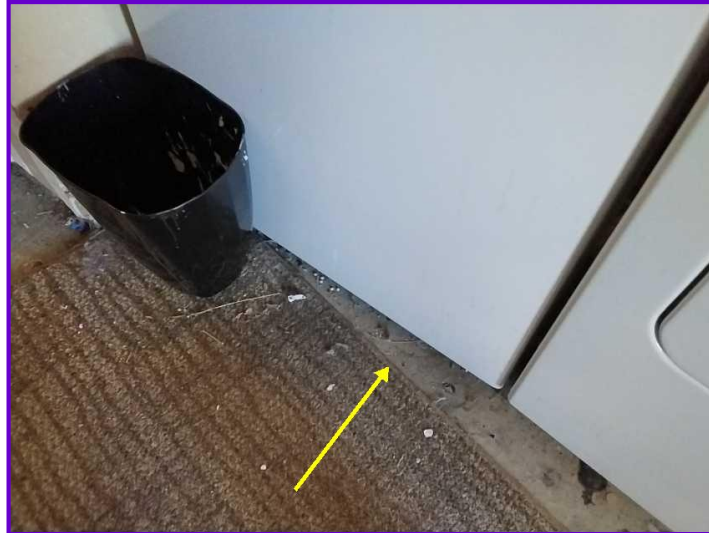
Laundry Provisions Washer Drain Pan
