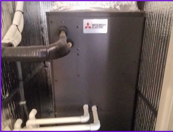
Heat Pump Heat and AC
