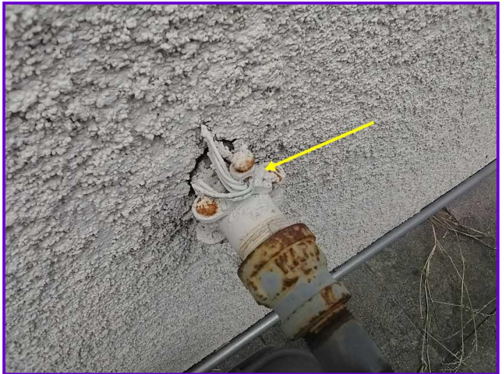
Main Panel Grounding Electrode System
