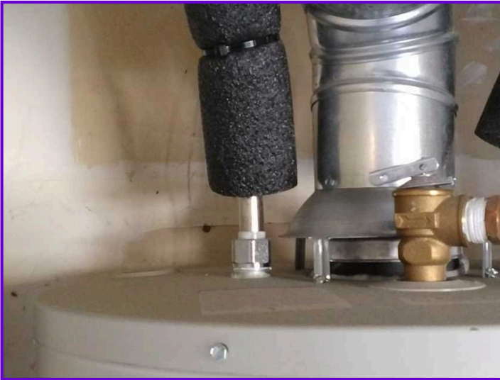
Water Heater Water Line Connectors
