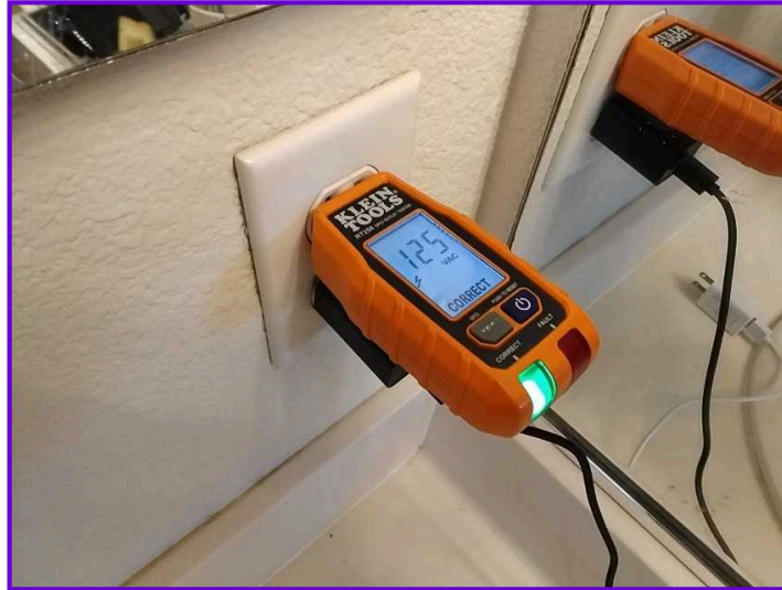
Receptacle Outlets Interior Outlets
