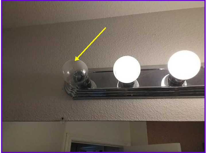
Lights and Switches Interior
