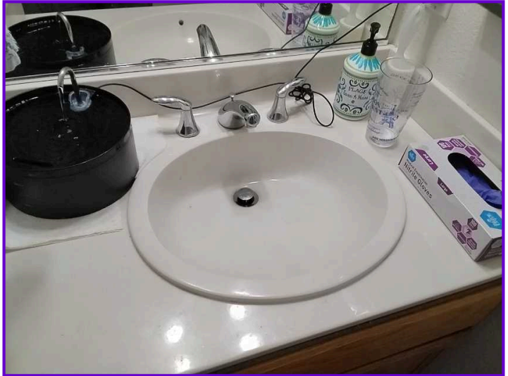
Plumbing Fixtures Sinks
