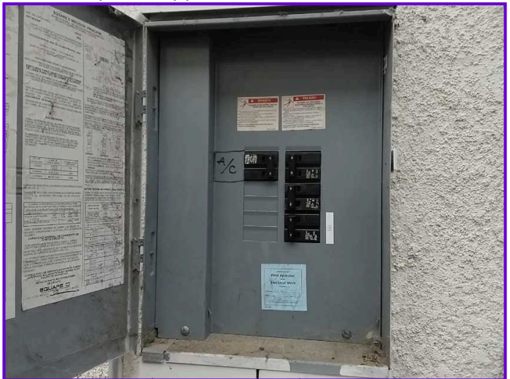
Main Panel Panel Covers
