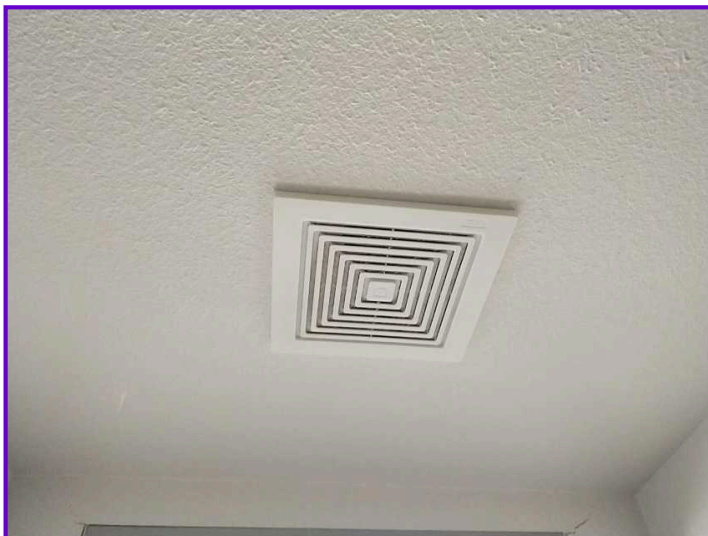
Ventilation and Exhaust Bathroom
