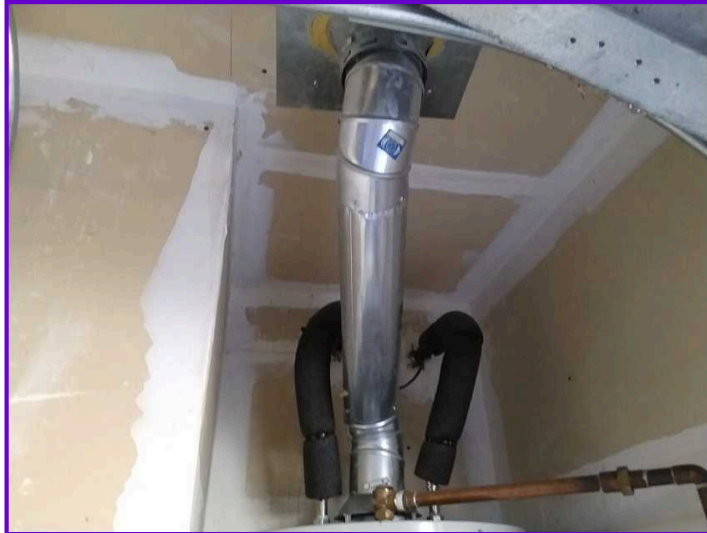
Water Heater Venting Provisions
