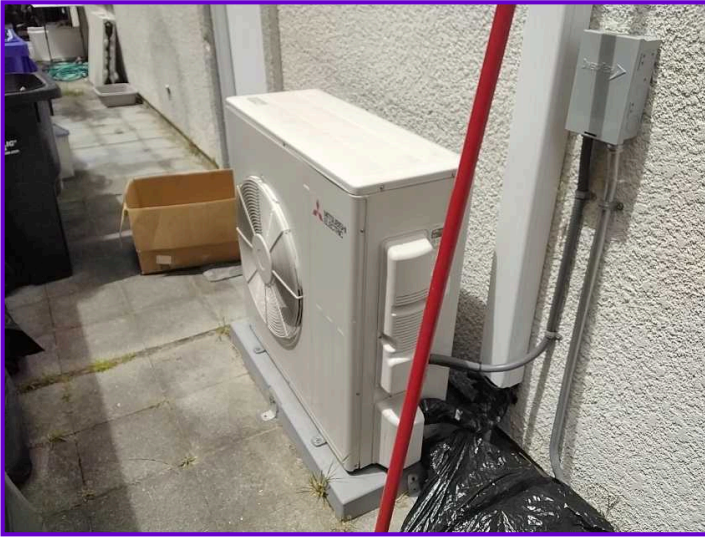
Heat Pump Heat and AC
