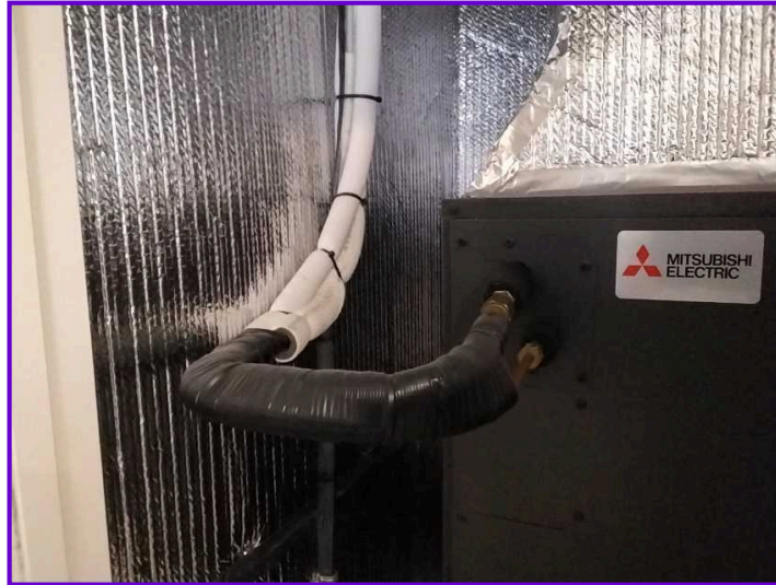
Heat Pump Refrigerant Lines
