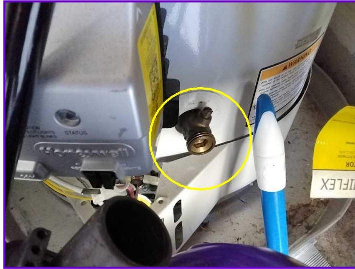
Water Heater Drain Valve
