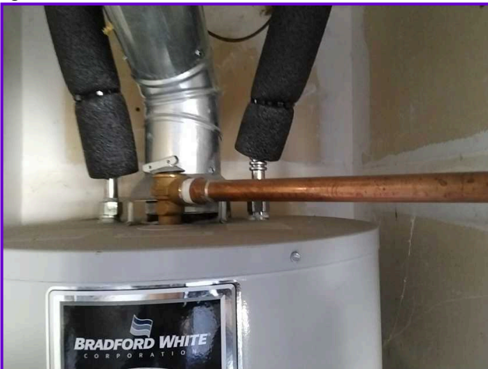
Water Heater TPR Valve
