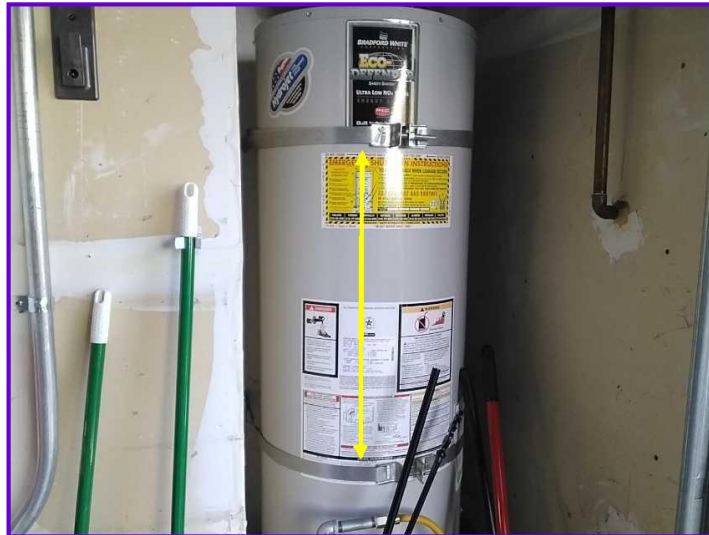
Water Heater Seismic Bracing
