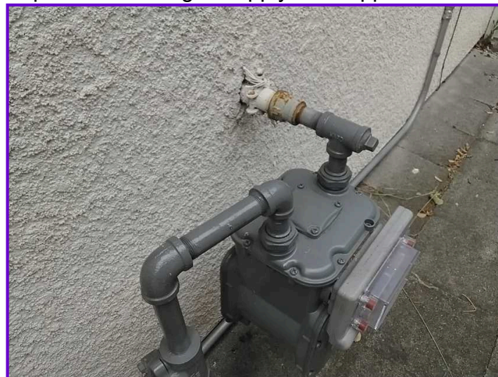
Gas Supply System Lines and Valves
