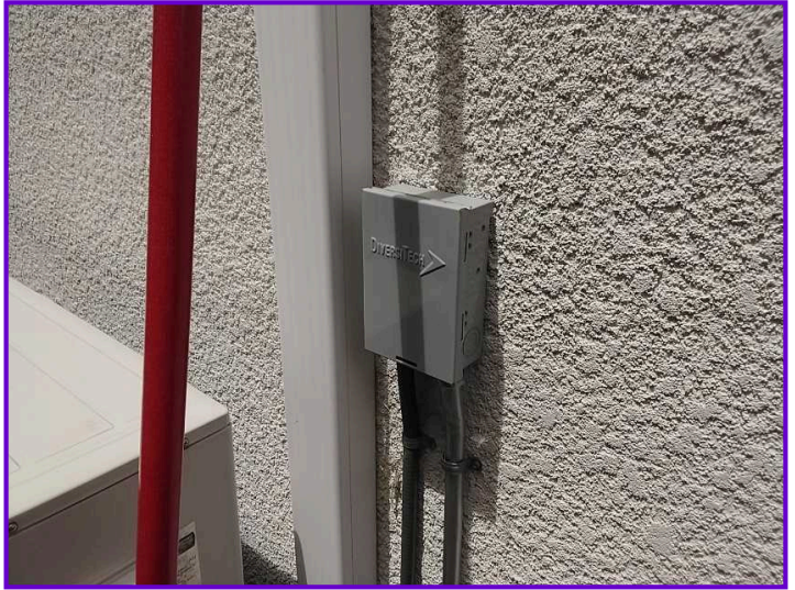
Heat Pump Heat and AC
