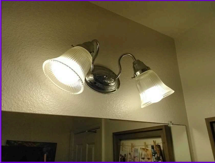
Lights and Switches Interior
