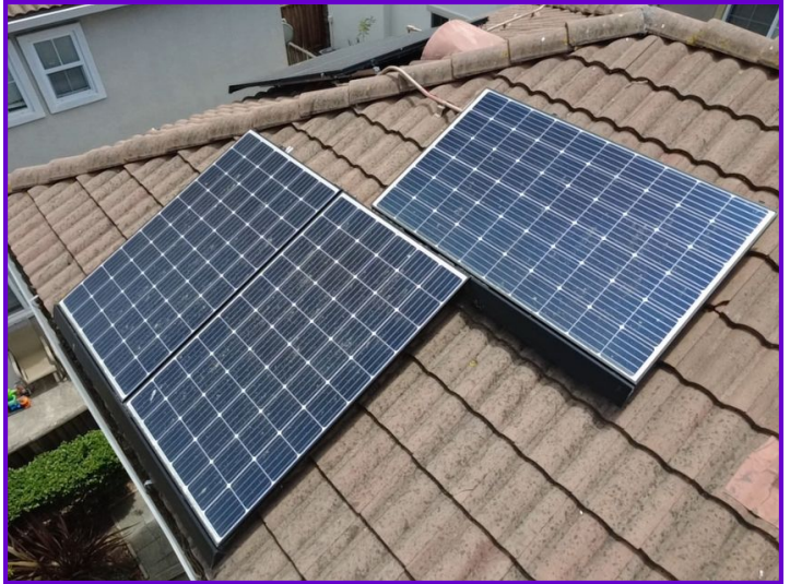
Photovoltaic System Photovoltaic System
