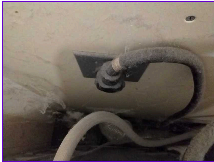
Laundry Provisions Electrical Supply
