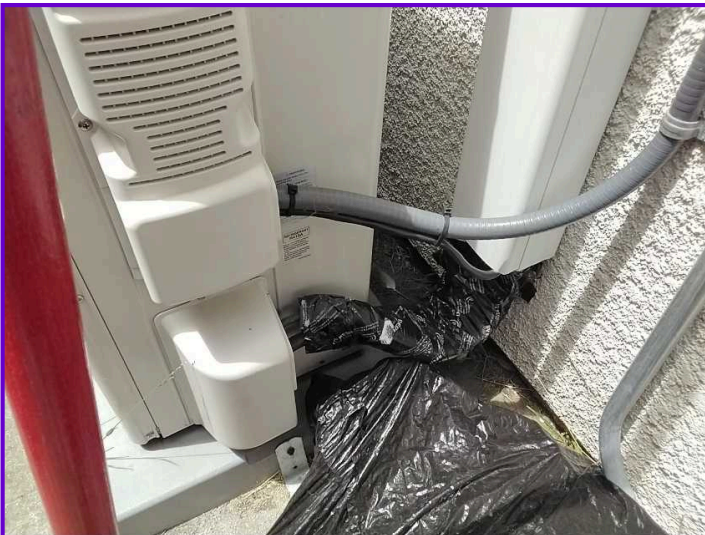
Heat Pump Heat and AC
