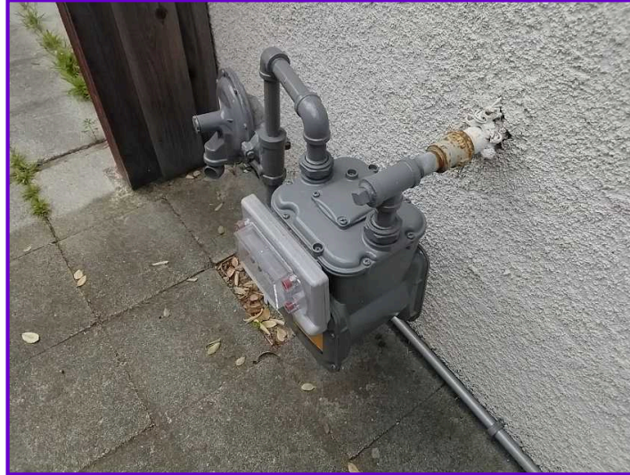
Gas Supply System Meter and Main
