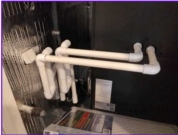
Heat Pump Condensate Drainage
