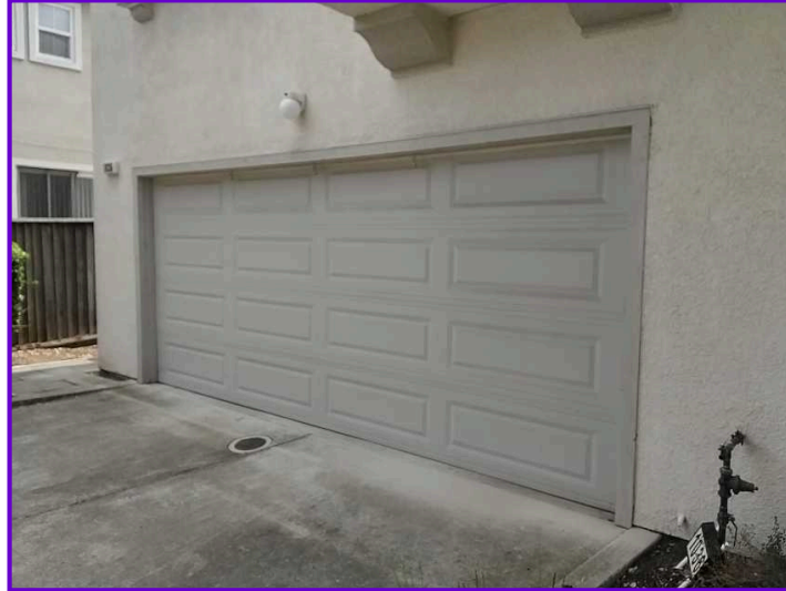
Vehicle Doors Vehicle Doors
