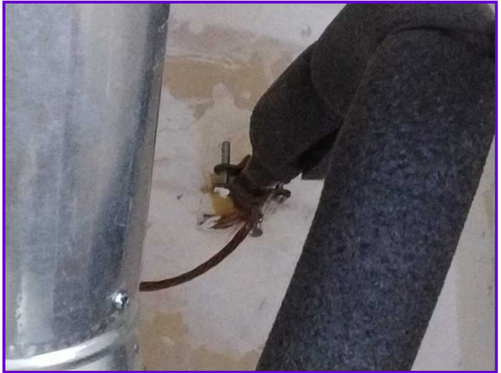
Water Heater Water Line Connectors
