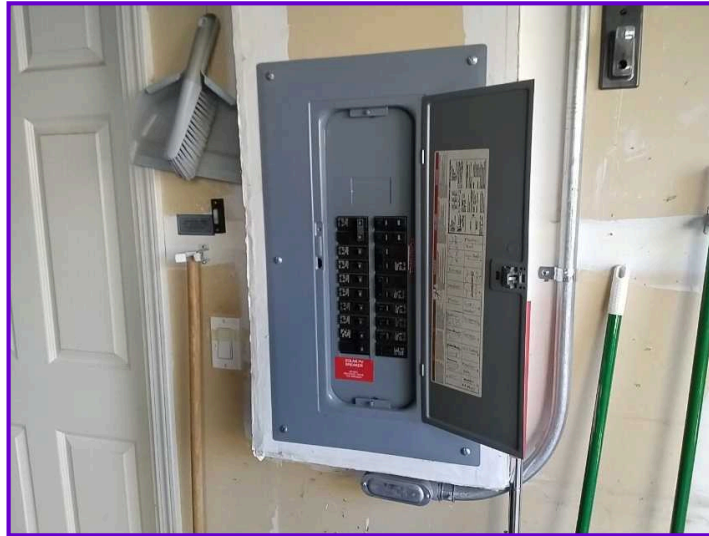
Sub Panel Sub Panel
