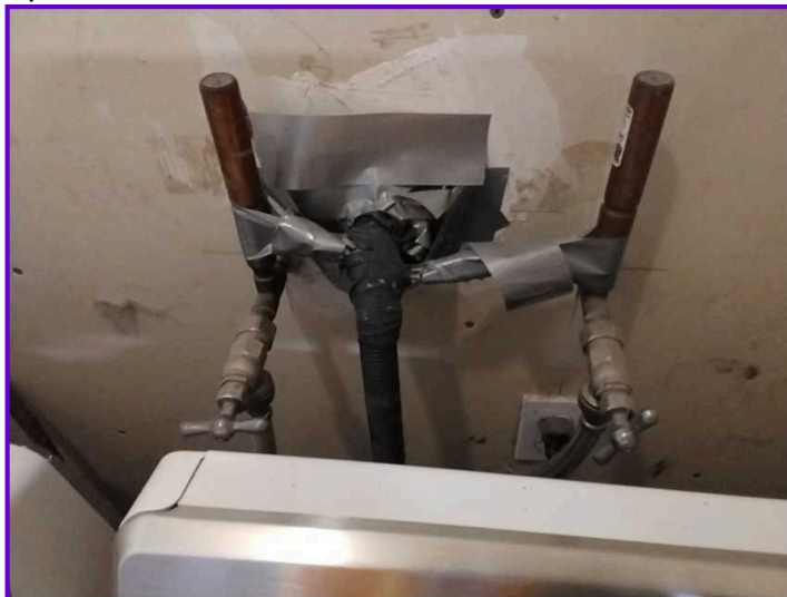
Laundry Provisions Washer Water Supply
