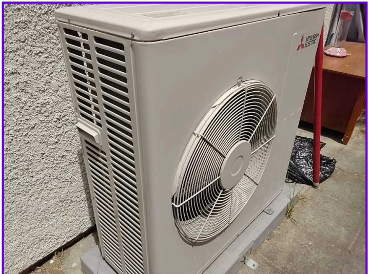
Heat Pump Heat and AC
