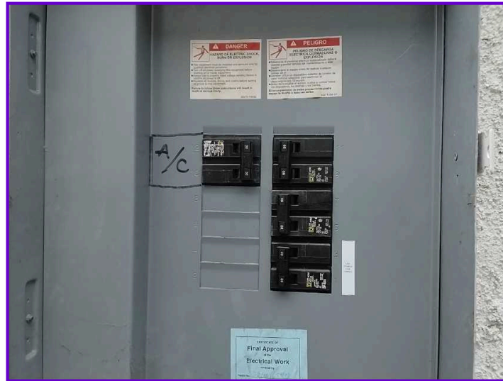
Main Panel Circuit Breakers
