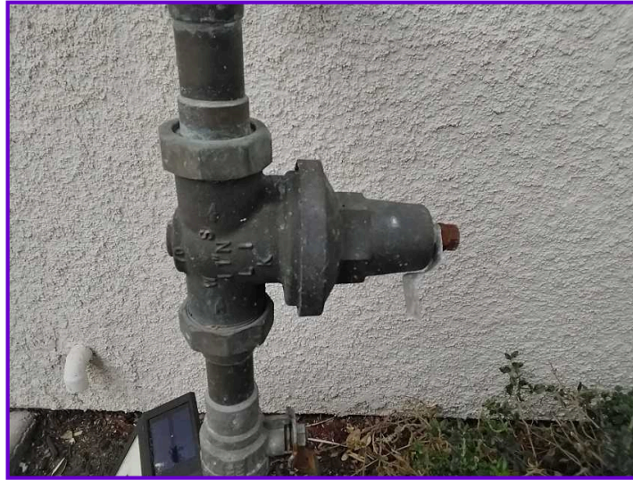
Water Supply System Pressure Regulator
