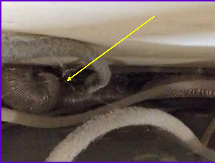
Laundry Provisions Dryer Venting
