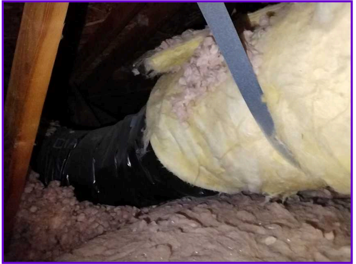
Heat Pump Distribution System
