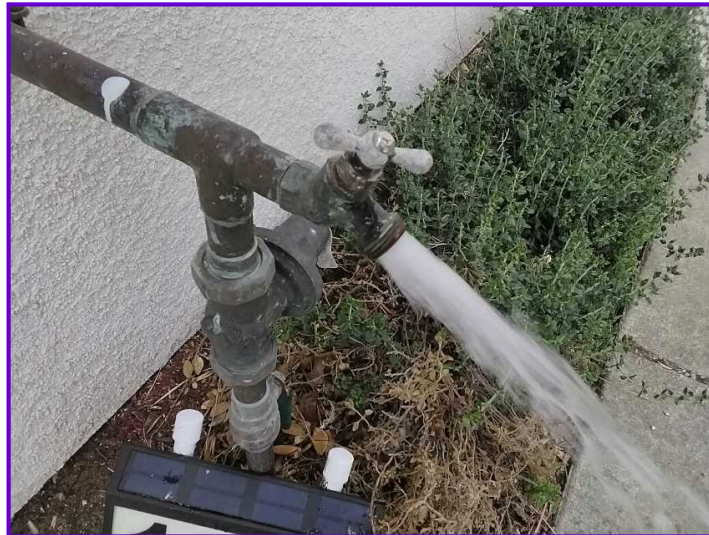
Water Supply System Hose Bibs
