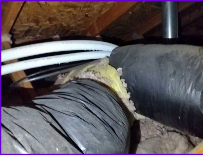
Heat Pump Distribution System
