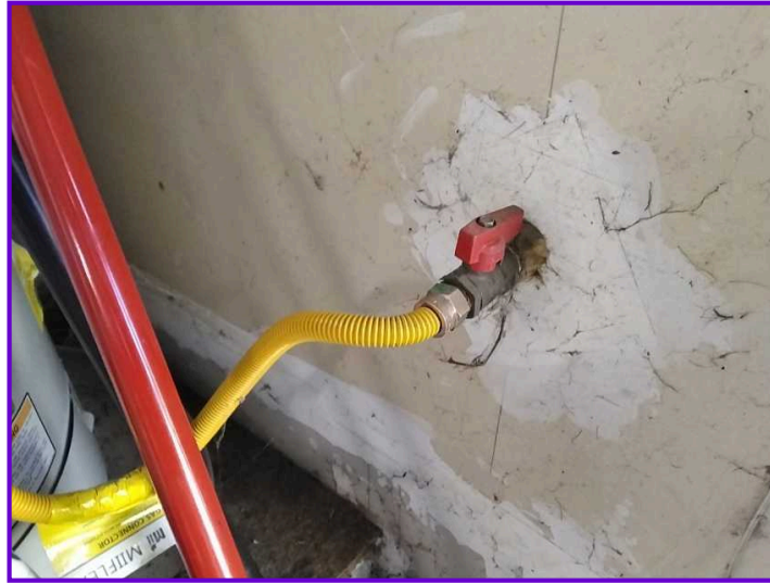
Water Heater Gas Shut-Off Valve
