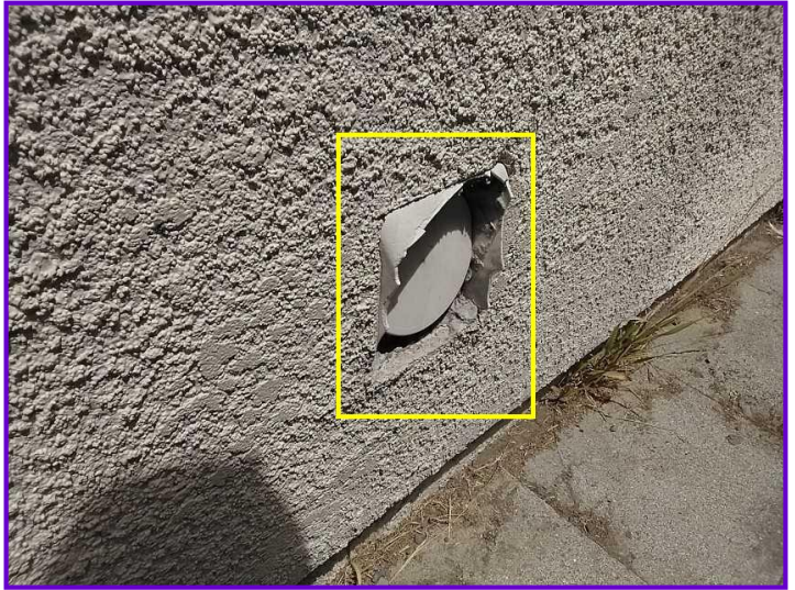
Laundry Provisions Dryer Venting
