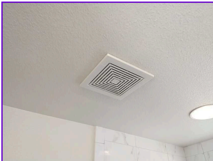
Ventilation and Exhaust Bathroom
