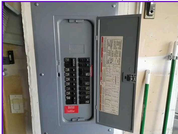
Sub Panel Panel Covers
