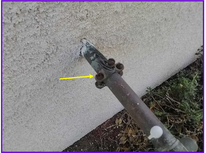
Sub Panel Grounding
