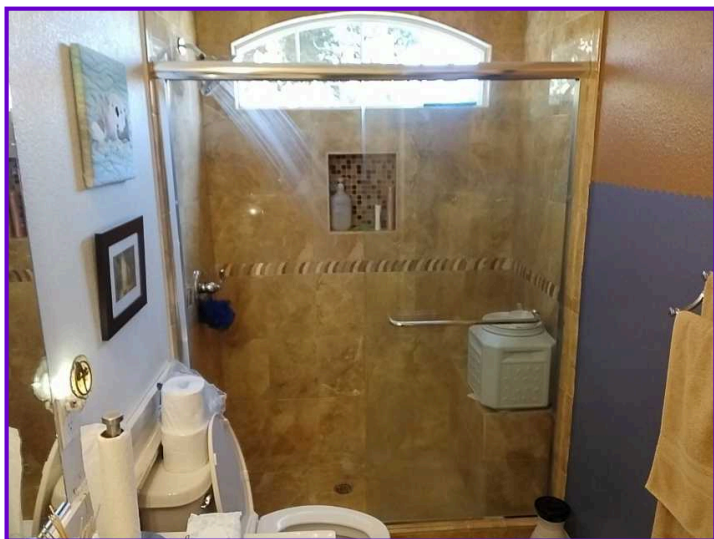
Plumbing Fixtures Stall Showers
