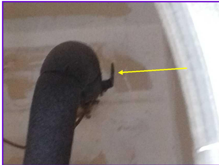
Water Heater Water Shut-Off Valve
