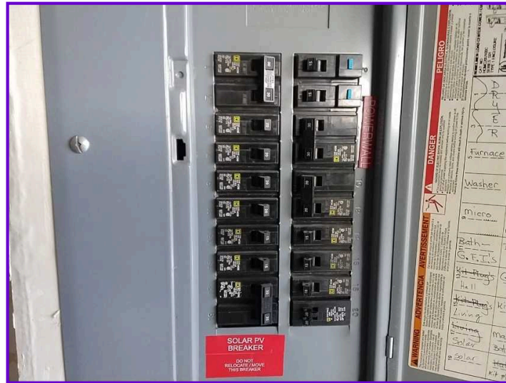
Sub Panel Circuit Breakers
