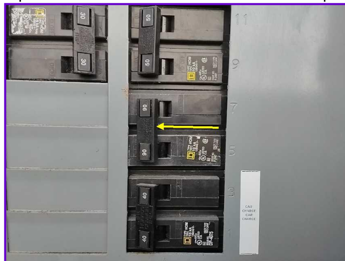
Main Panel Main Disconnect
