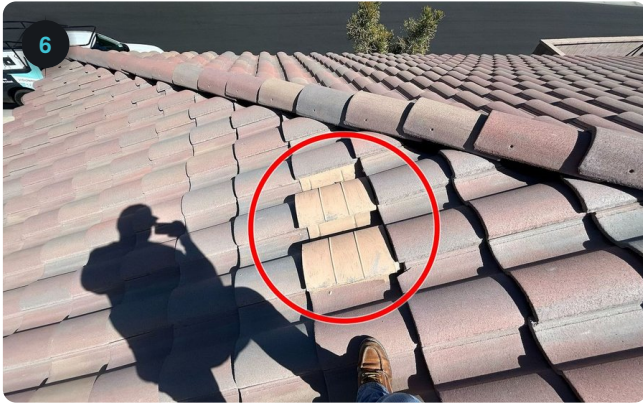
Figure 6 — Worn paint, tile field
