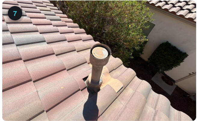
Figure 7 — Worn paint, vent flashing
