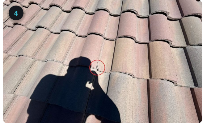
Figure 4 — Chipped tile, close-up
