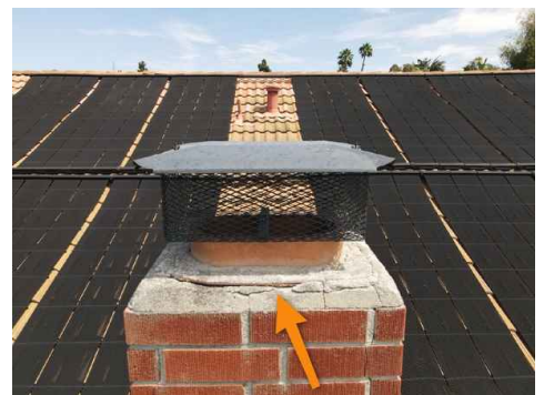
Example Noted At Roof
