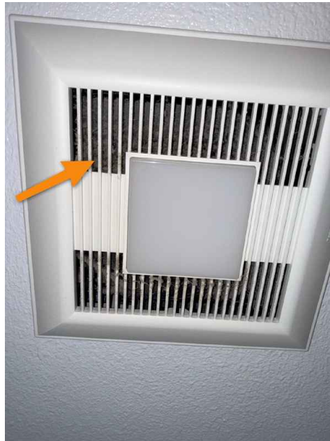
Example Noted At Primary Bathroom
