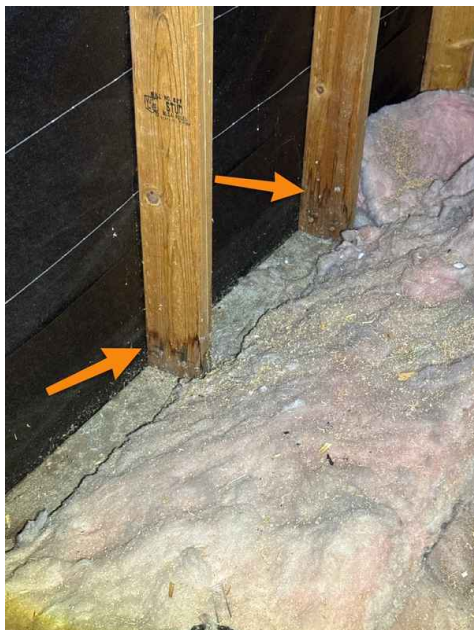
Example Noted At Attic
