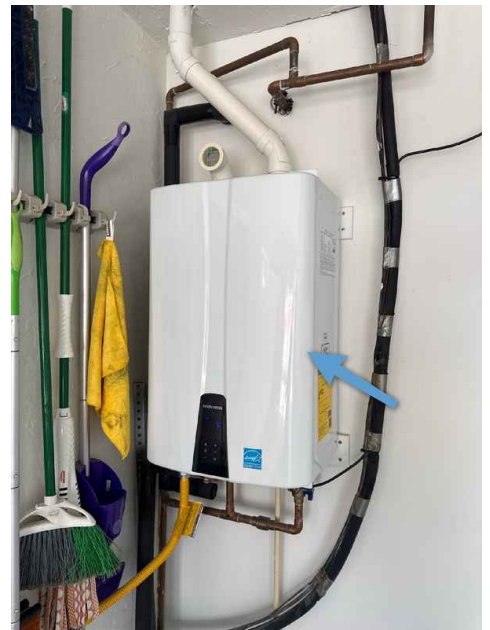
Example Noted At Water Heater
