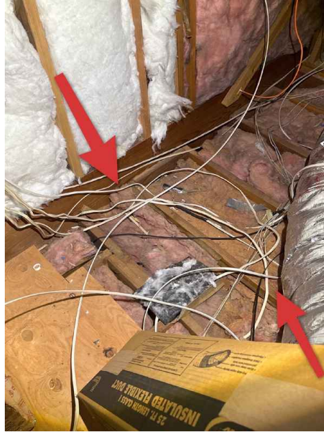
Example Noted At Attic
