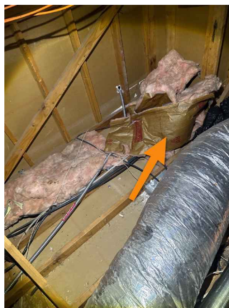
Example Noted At Attic
