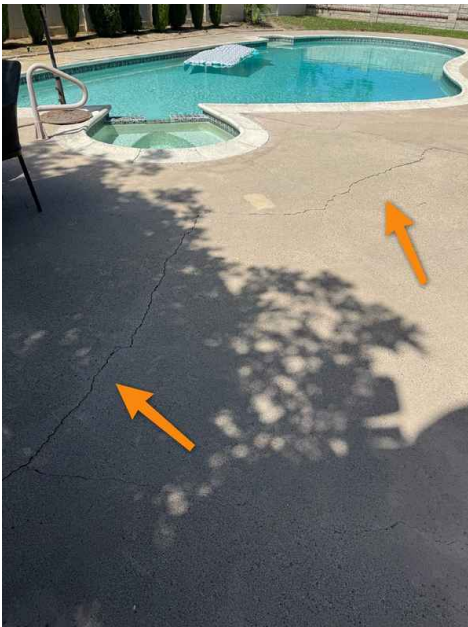
Example Noted At Rear Side Of Home
