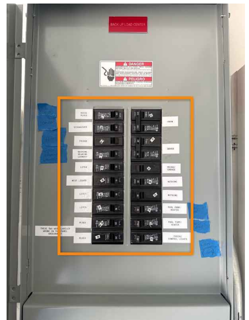
Example Noted At Sub Panel
