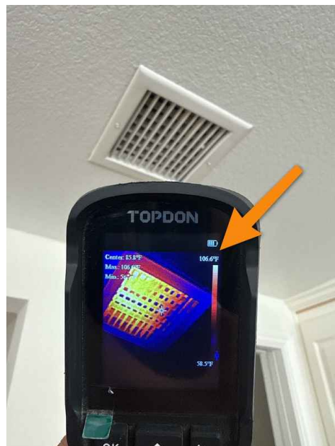
Example Noted At Kitchen
