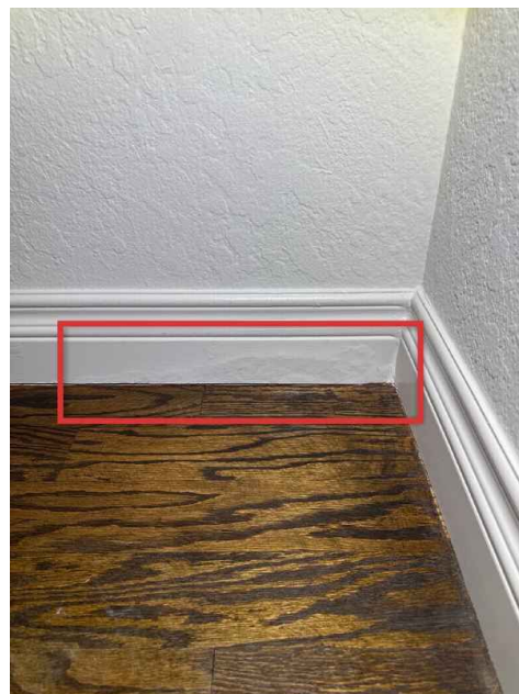
Example Noted At Dining Room
