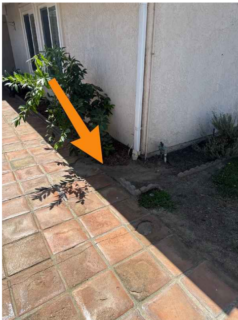
Example Noted At Front Of Home
