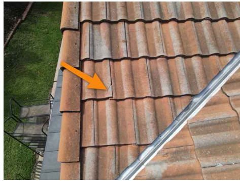
Example Noted At Roof
