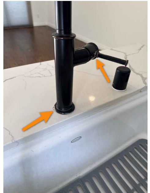
Example Noted At Kitchen
