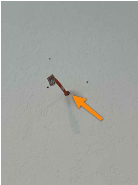
Example Noted At Living Room
