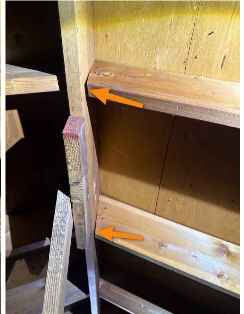
Example Noted At Attic
