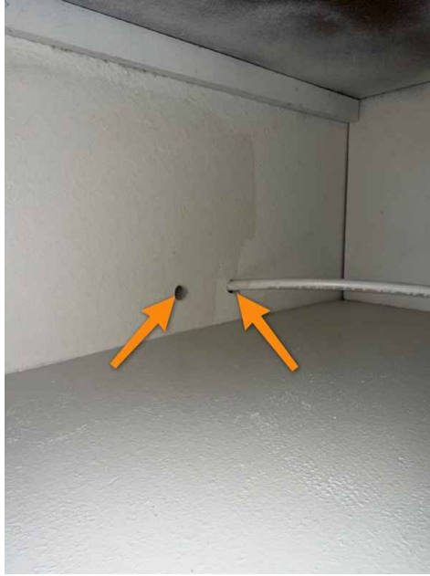
Example Noted At Kitchen
