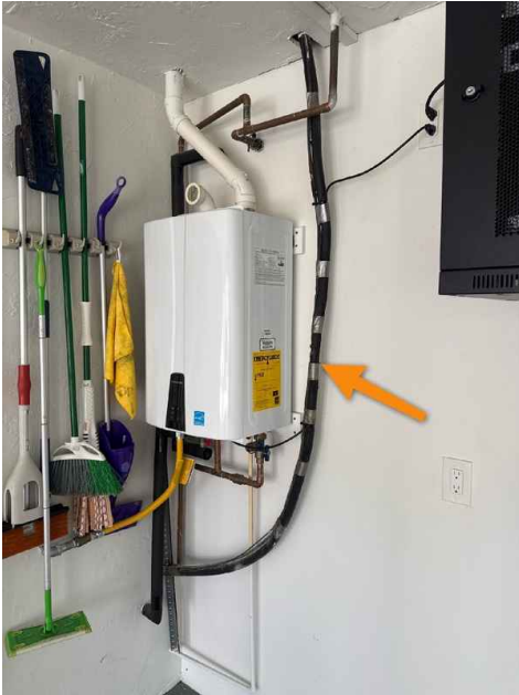
Example Noted At Garage
