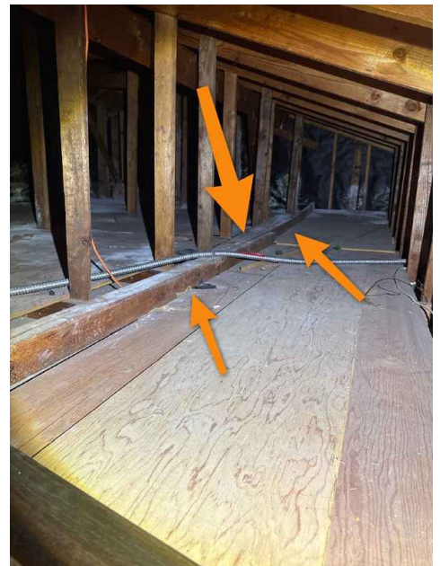
Example Noted At Garage Attic
