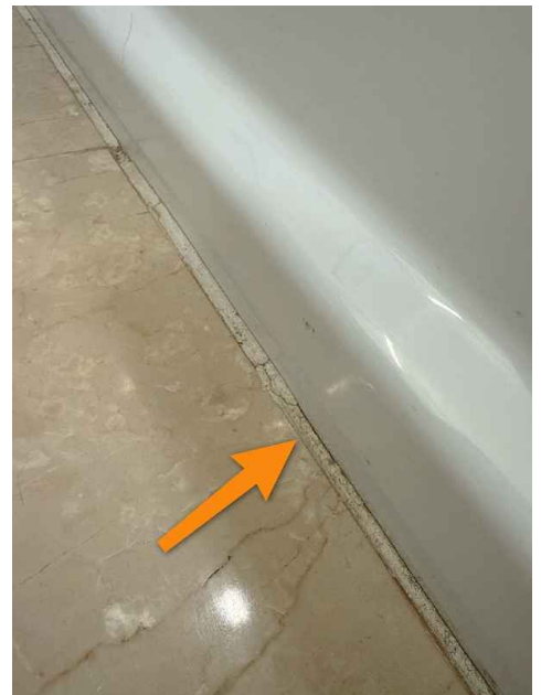
Example Noted At Hallway Bathroom
