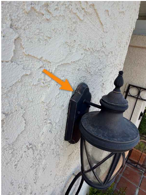
Example Noted At Front Of Home
