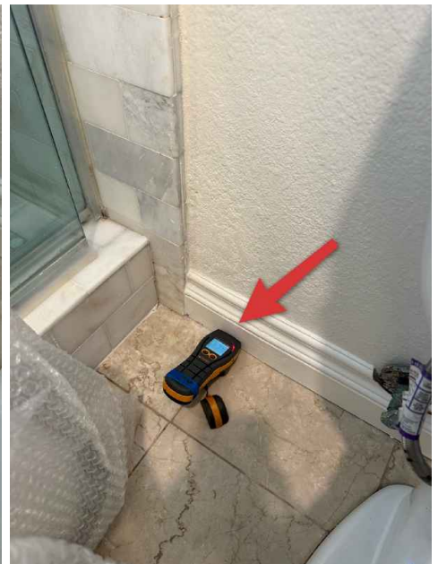
Example Noted At Primary Bathroom
