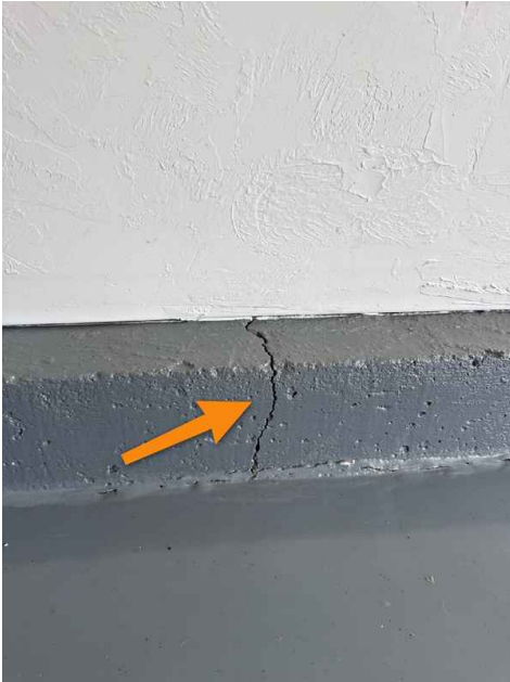
Example Noted At Garage
