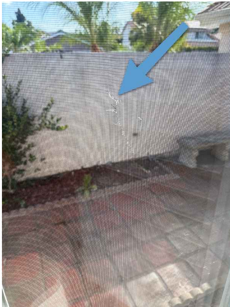
Example Noted At Bedroom 2
