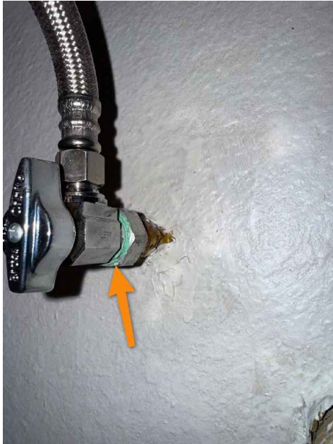
Example Noted At Hallway Bathroom
