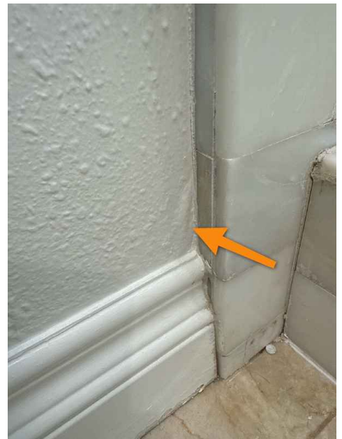
Example Noted At Primary Bathroom
