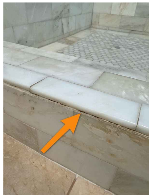
Example Noted At Primary Bedroom
