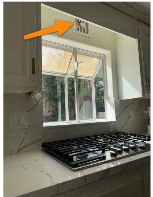
Example Noted At Kitchen
