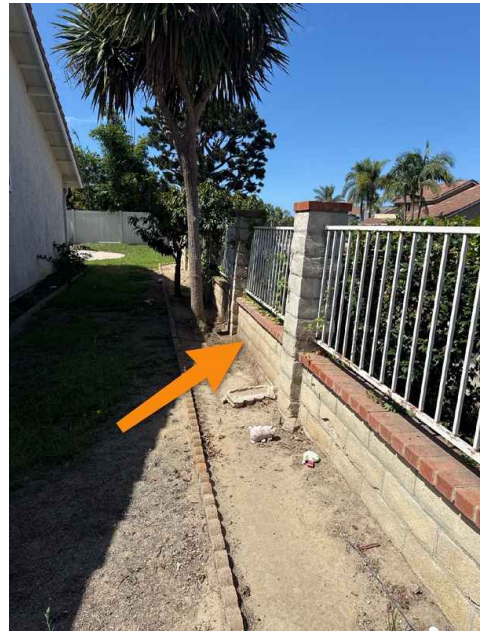
Example Noted At Right Side Of Home
