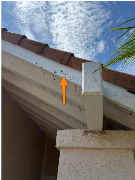
Example Noted At Front Of Home
