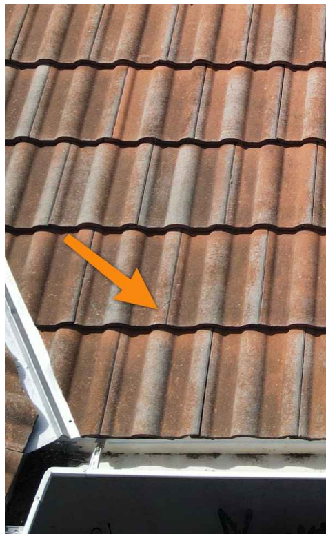
Example Noted At Roof
