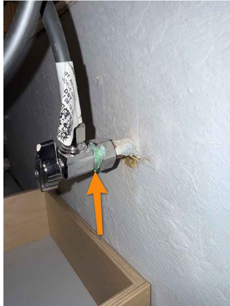
Example Noted At Primary Bathroom
