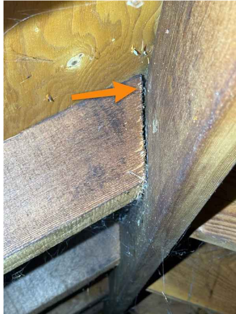
Example Noted At Garage Attic
