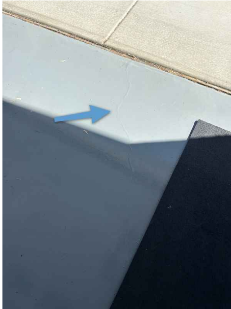
Example Noted At Garage
