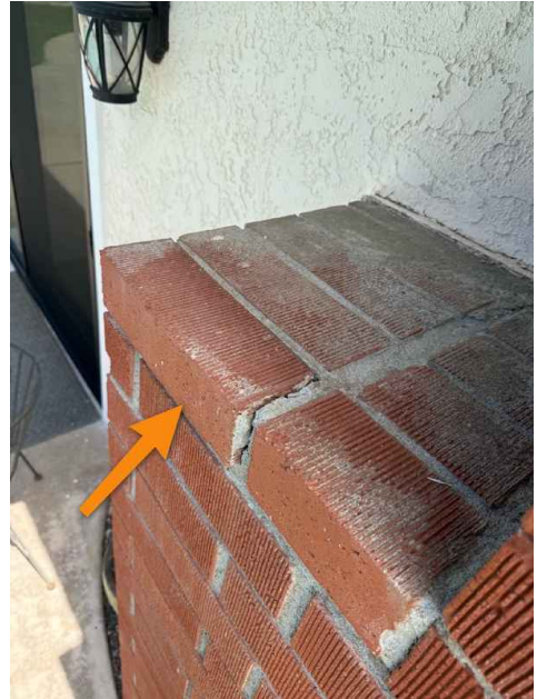
Example Noted At Rear Side Of Home
