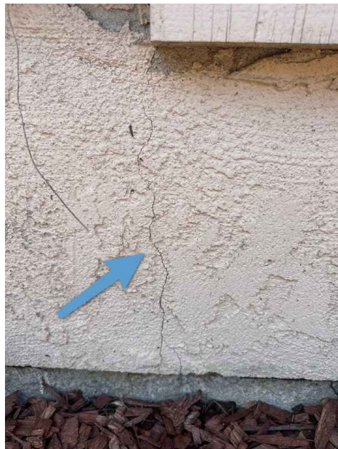
Example Noted At Front Of Home
