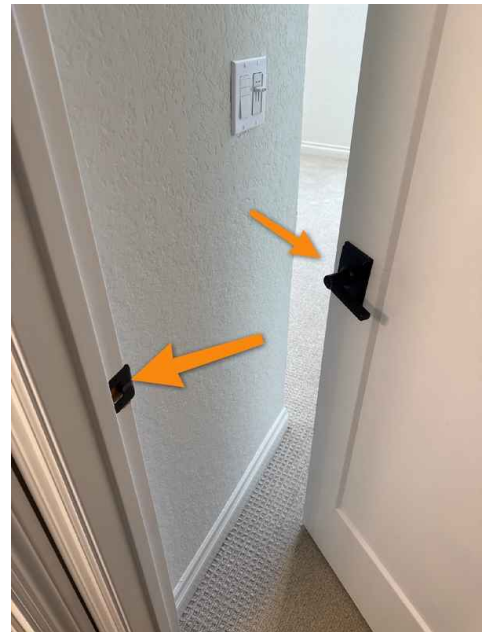
Example Noted At Bedroom 2
