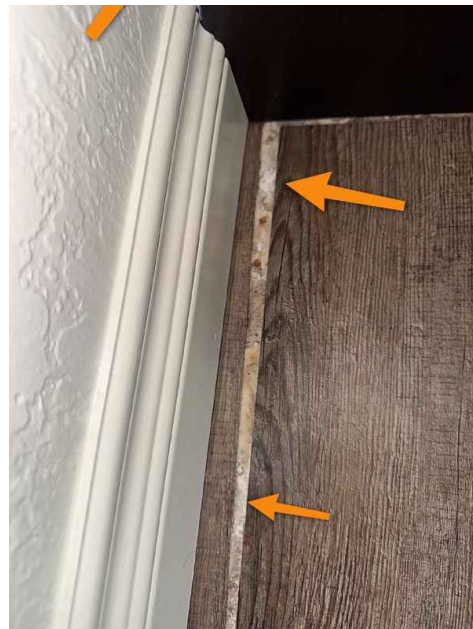
Example Noted At Primary Bedroom Closet
