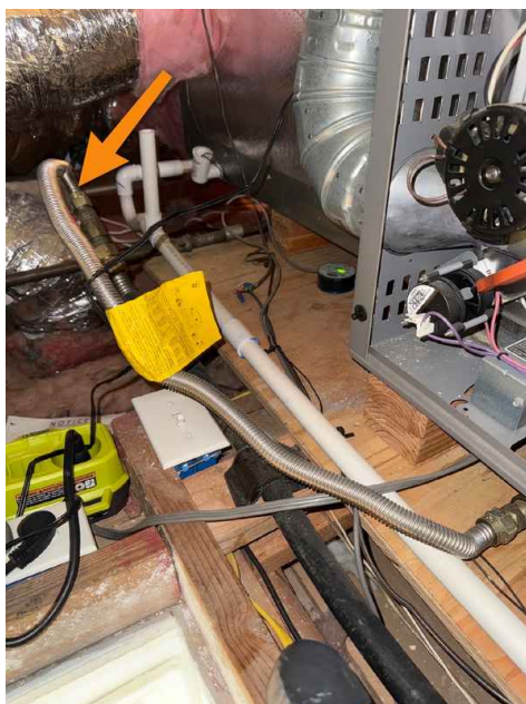
Example Noted At FAU
