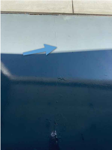
Example Noted At Garage
