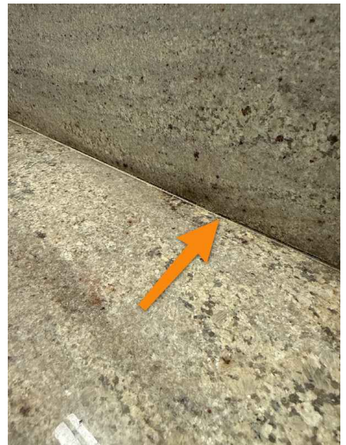
Example Noted At Primary Bathroom
