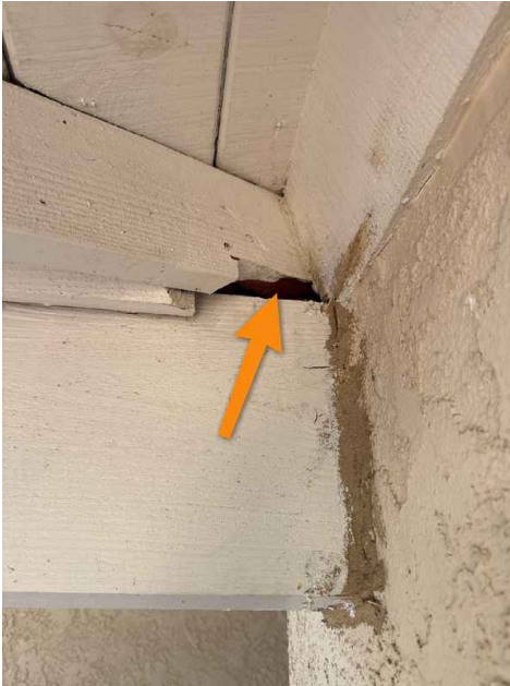
Example Noted At Front Of Home
