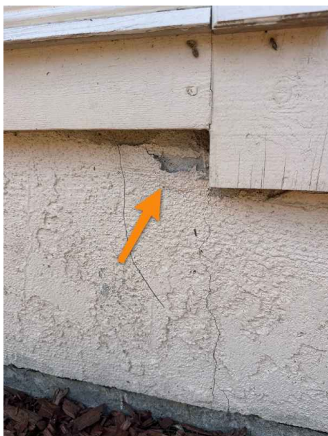
Example Noted At Front Of Home
