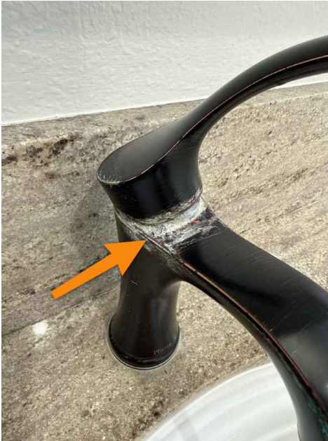
Example Noted At Hallway Bathroom
