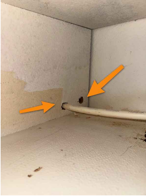
Example Noted At Kitchen
