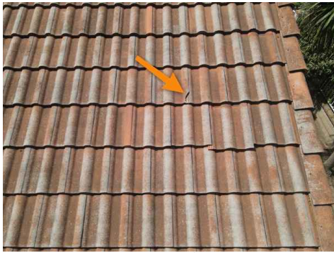
Example Noted At Roof
