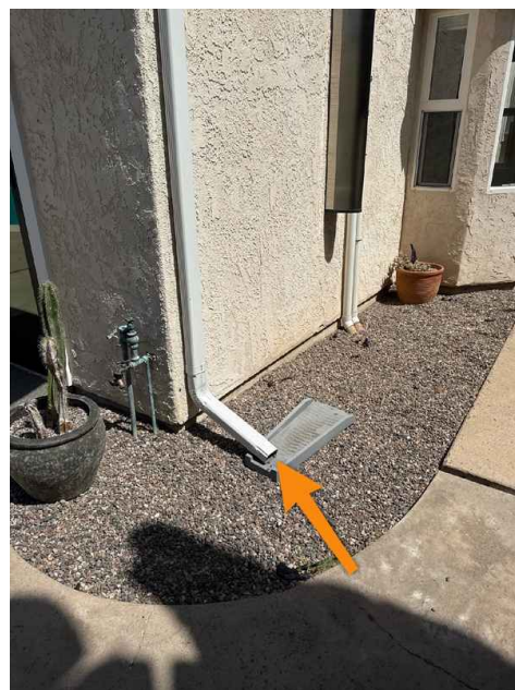
Example Noted At Rear Side Of Home
