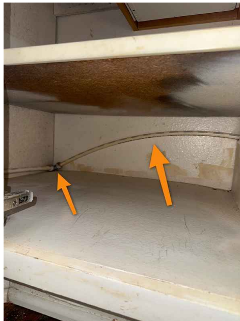
Example Noted At Kitchen
