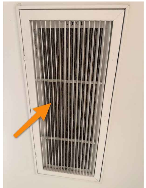
Example Noted At Hallway
