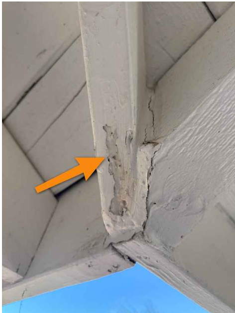
Example Noted At Front Of Home
