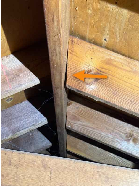
Example Noted At Garage Attic
