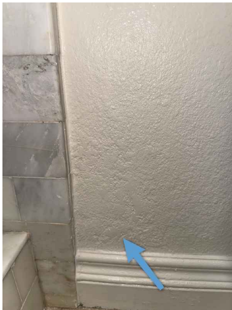
Example Noted At Primary Bathroom
