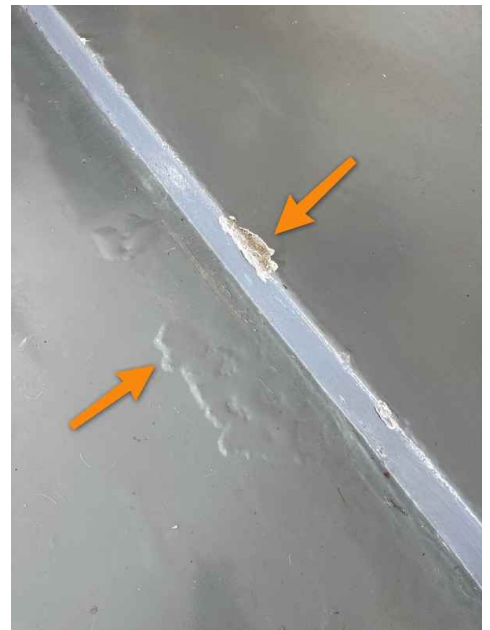
Example Noted At Garage
