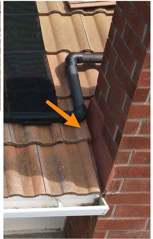
Example Noted At Roof
