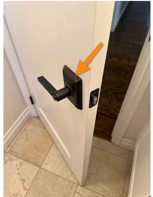
Example Noted At Hallway Bathroom
