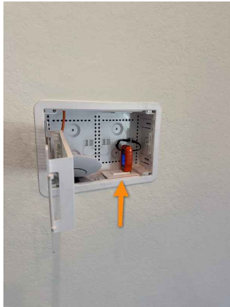
Example Noted At Living Room
