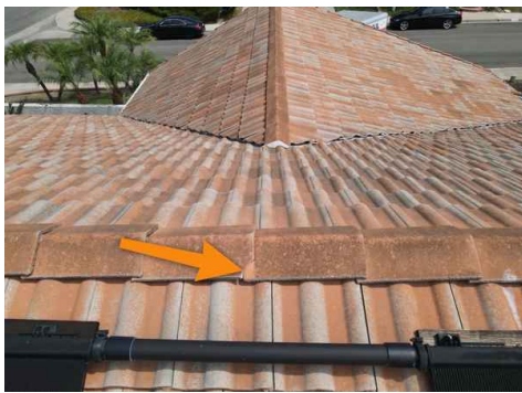
Example Noted At Roof
