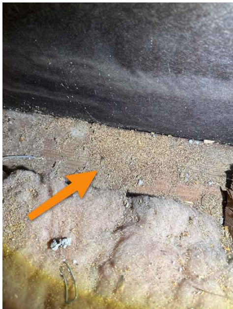
Example Noted At Attic
