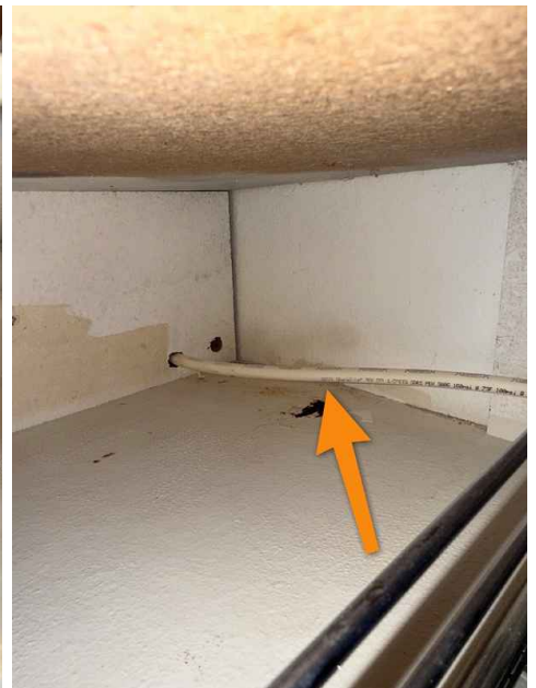
Example Noted At Kitchen
