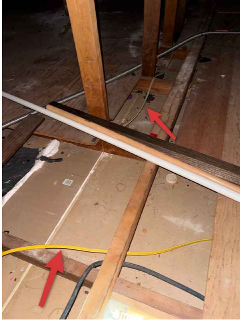
Example Noted At Garage Attic
