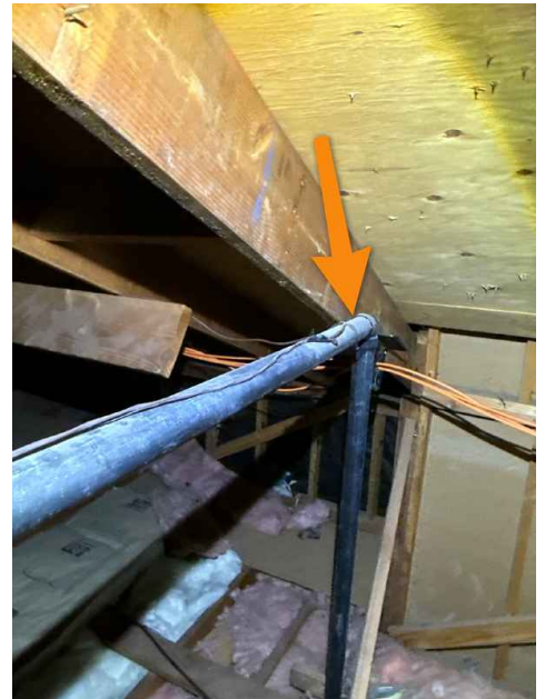
Example Noted At Attic
