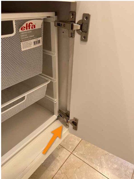
Example Noted At Hallway Bathroom
