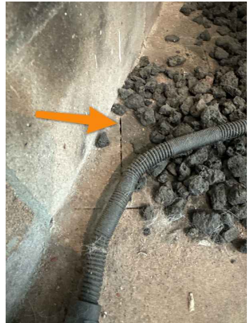
Example Noted At Living Room
