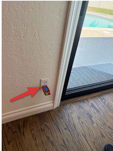
Example Noted At Living Room
