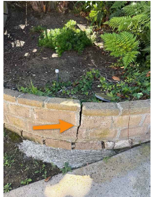
Example Noted At Rear Side Of Home
