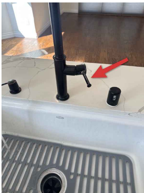
Example Noted At Kitchen
