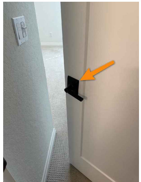
Example Noted At Bedroom 2
