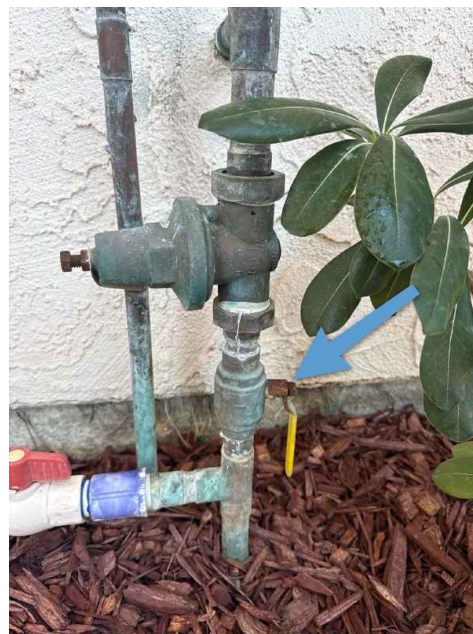
Example Noted At Front Of Home
