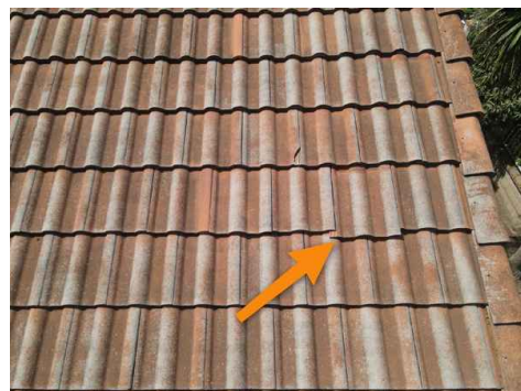
Example Noted At Roof
