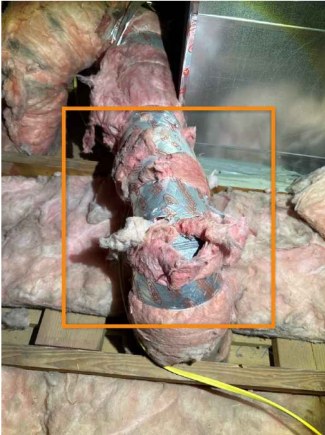
Example Noted At Attic
