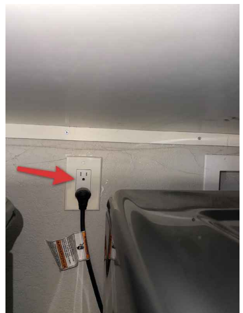
Example Noted At Laundry Room
