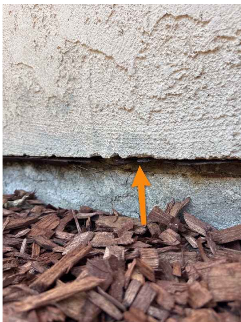
Example Noted At Front Of Home
