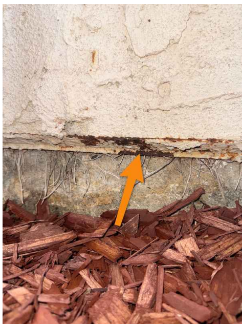
Example Noted At Front Of Home
