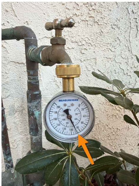
Example Noted At Front Of Home
