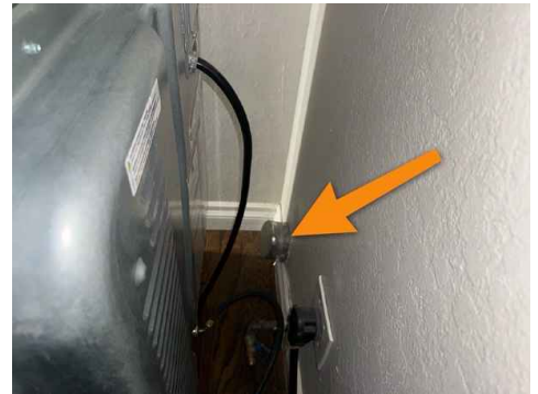
Example Noted At Laundry Room
