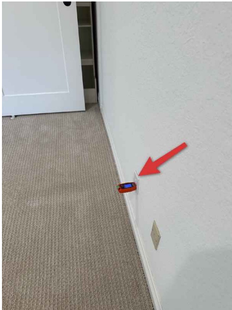
Example Noted At Bedroom 2
