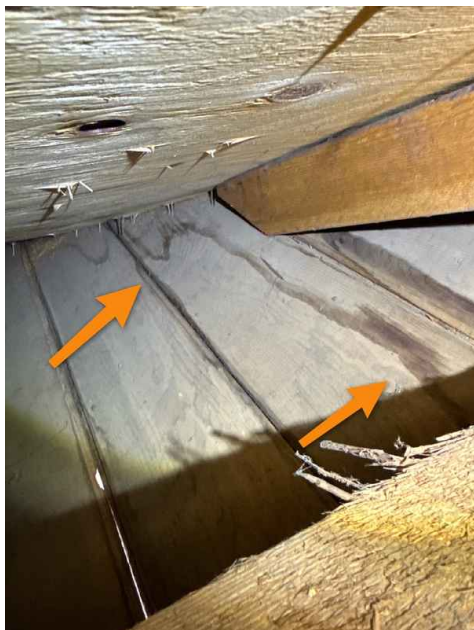
Example Noted At Attic
