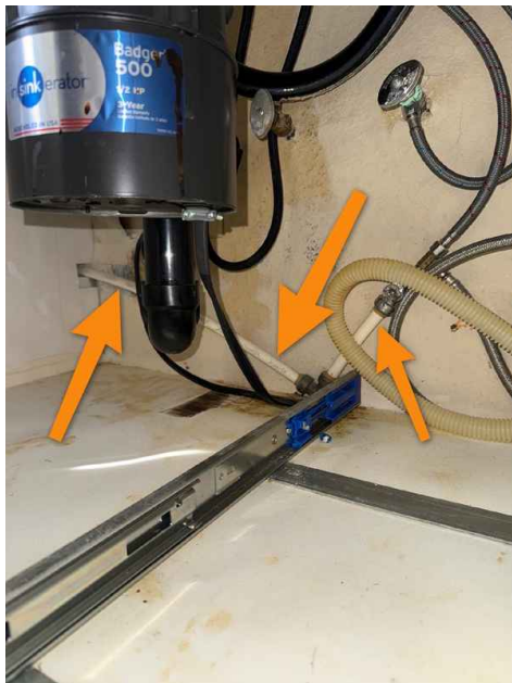
Example Noted At Kitchen
