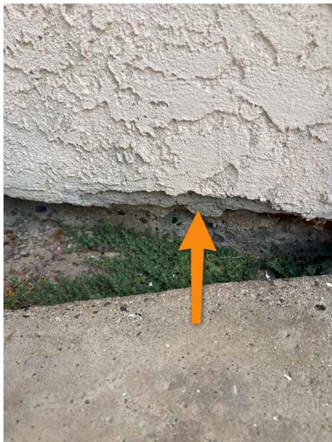
Example Noted At Rear Side Of Home
