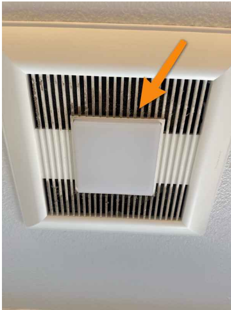
Example Noted At Hallway Bathroom
