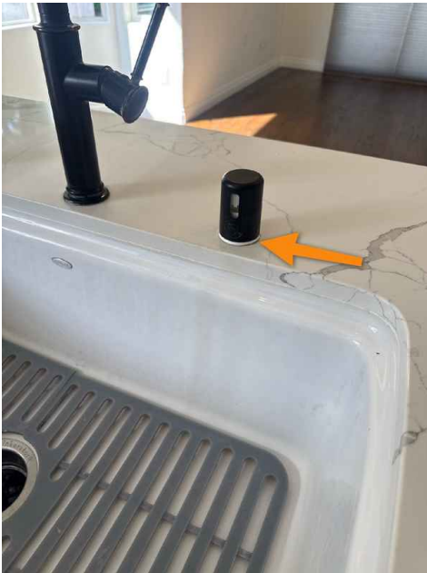
Example Noted At Kitchen
