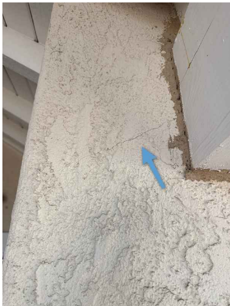
Example Noted At Front Of Home
