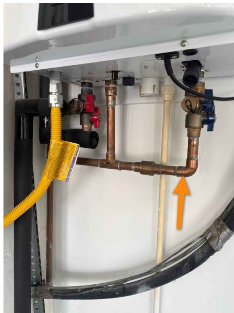
Example Noted At Water Heater
