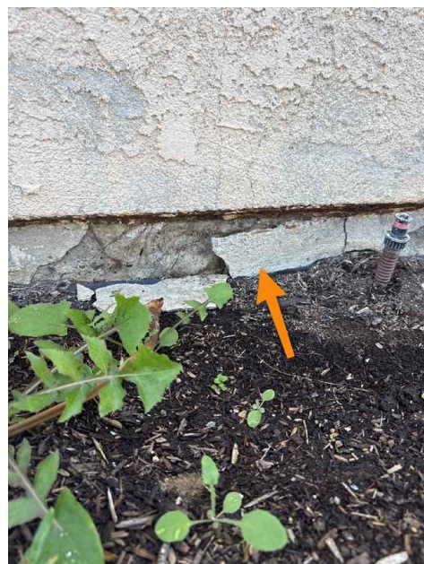
Example Noted At Right Side Of Home
