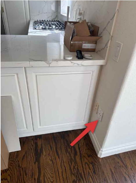
Example Noted At Kitchen
