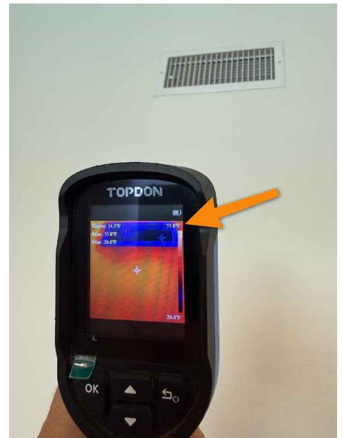
Example Noted At Living Room
