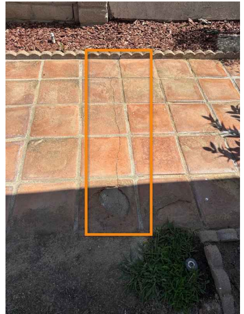
Example Noted At Front Of Home
