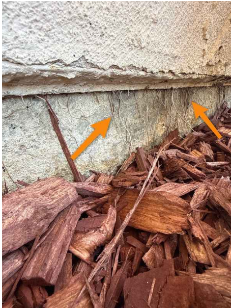
Example Noted At Front Of Home
