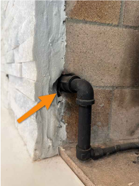
Example Noted At Living Room
