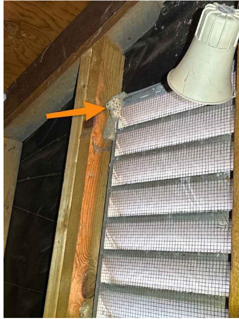
Example Noted At Attic
