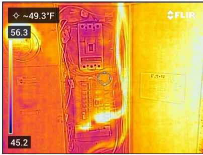
No abnormal heat in electric panels
