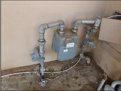
Gas front exterior
