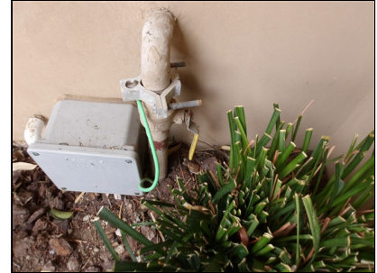
Multiple water shut off valves
