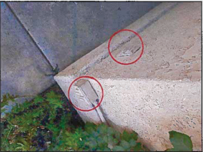
Missing GFCI exterior plugs
