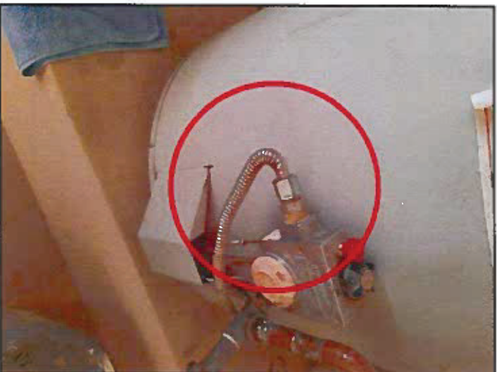
Missing drip leg hot water tank
