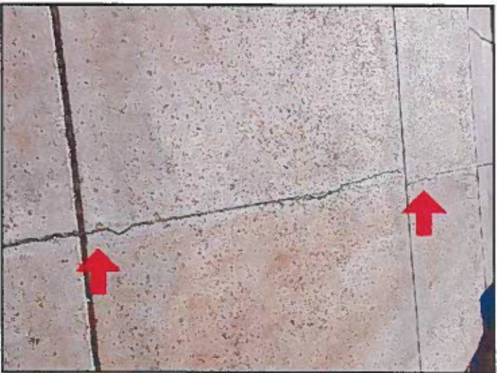
Cracked concrete driveway
