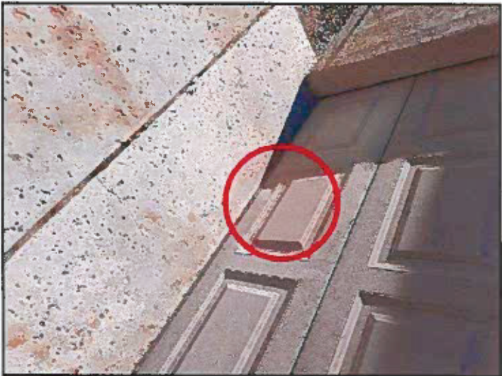
Dent in garage door
