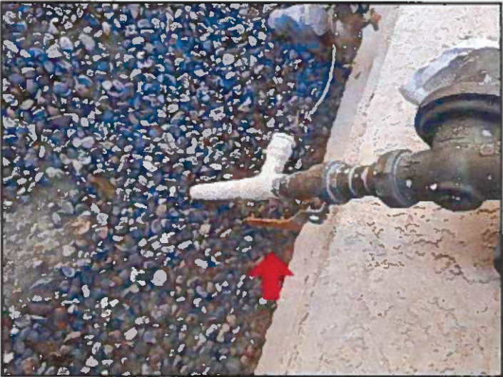
Main shut off for house
