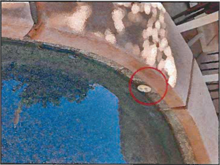
Inoperative controls at spa
