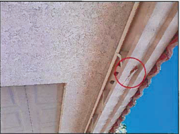
weathered fascia boards
