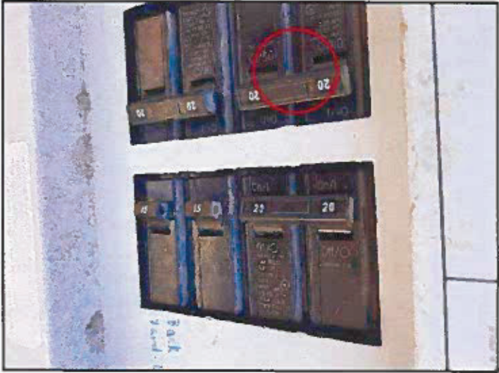
Missing GFCI pool pumps
