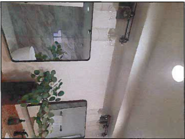
Missing light bulbs
