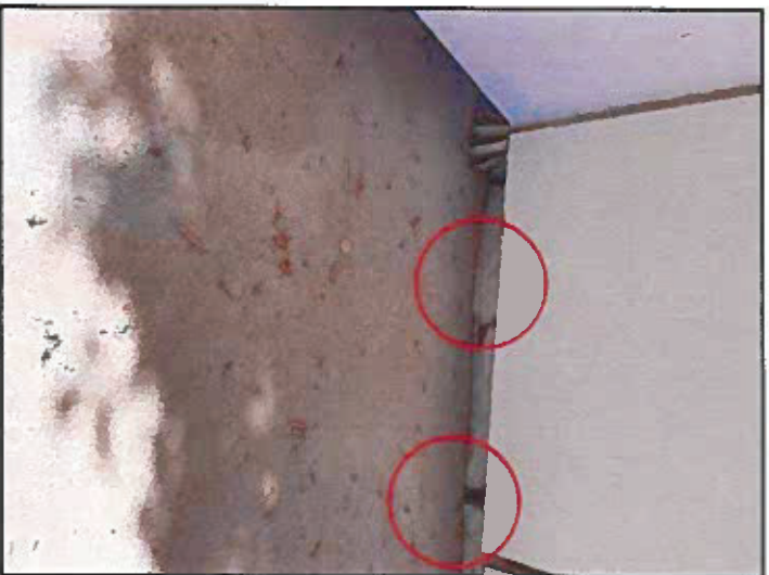
Storage cabinets garage water damaged
