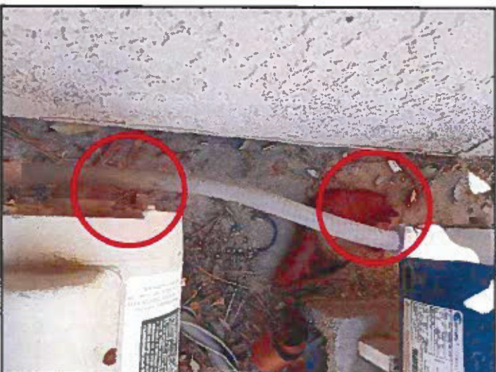
Missing body bond/ground
