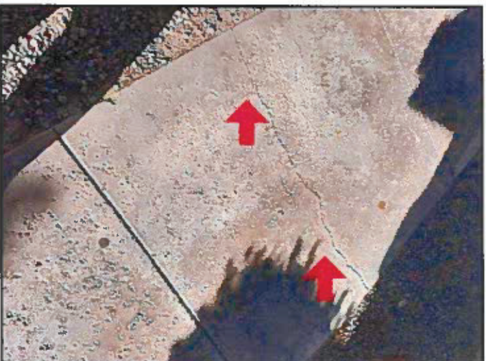
Cracked concrete walkway
