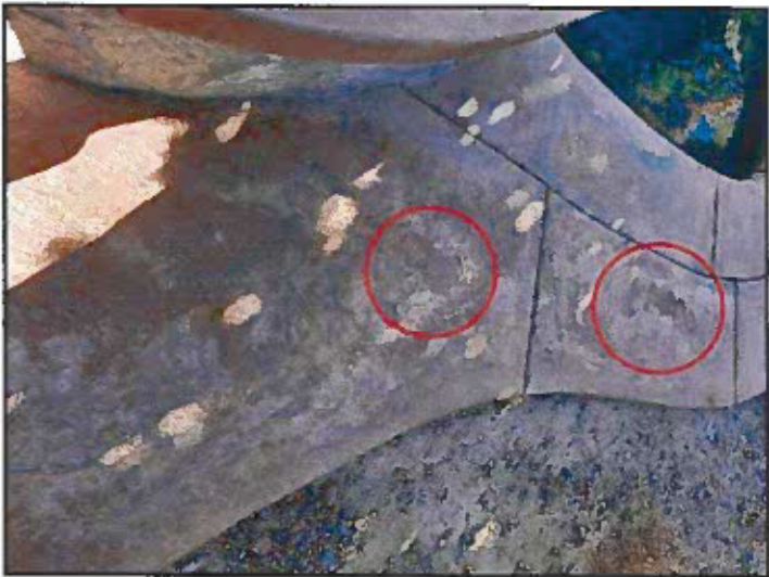
Surface damage pool area
