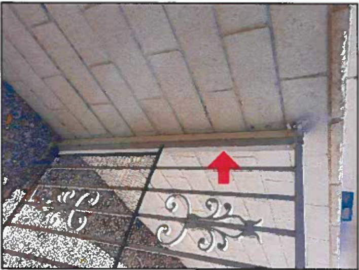
frame loose from wall
