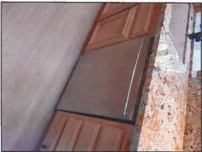
Drain pump is stuck on
