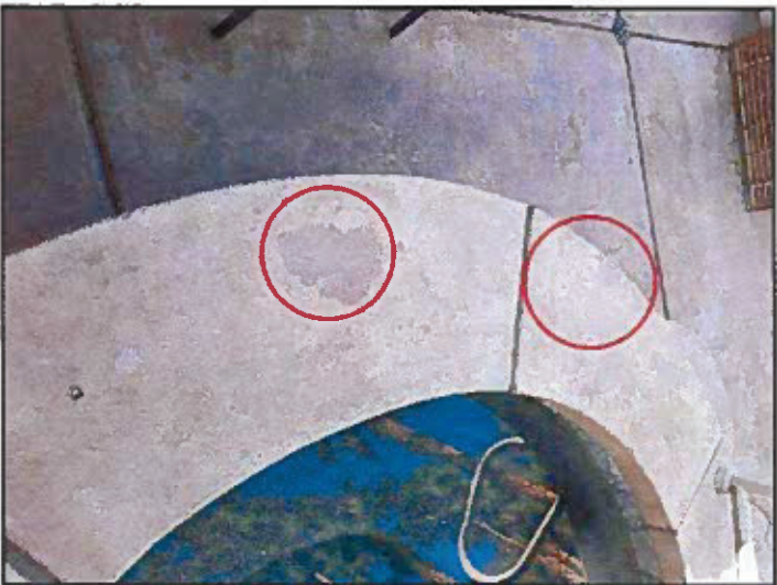
surface damaged pool area
