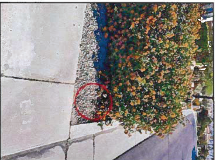
Unknown main meter shut off
