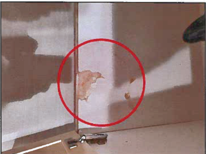
Damaged cabinet bathroom
