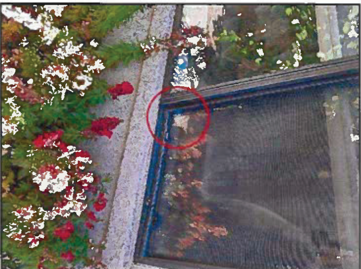
One damaged screen
