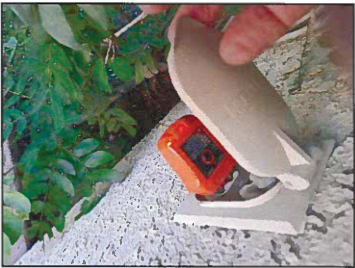
Missing GFCI exterior plug
