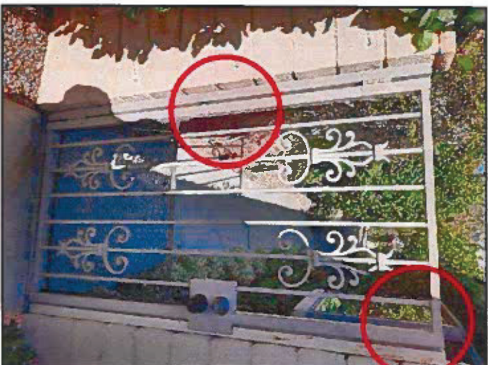
Missing high latch/ self closing spring
