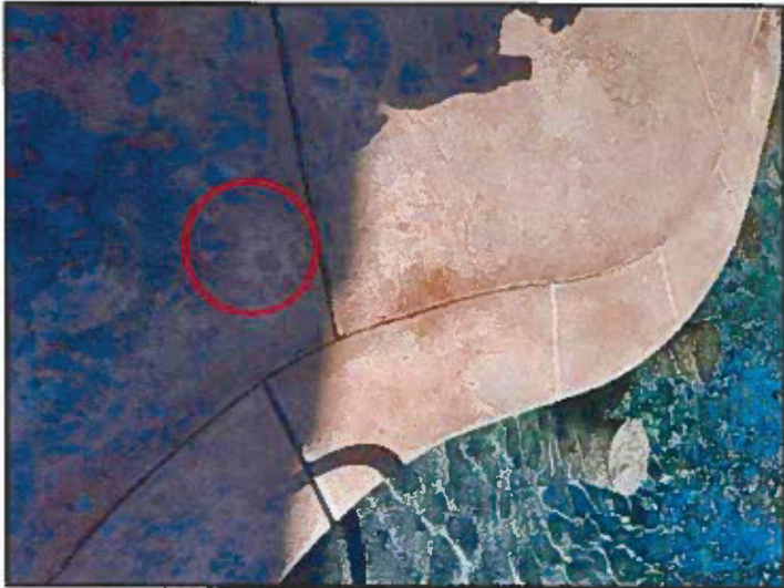
Common cracking pool area
