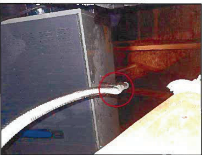
Missing drip leg heater
