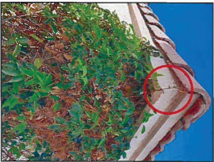
Weathered fascia board
