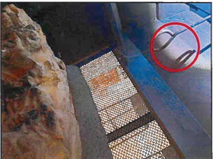
Missing damper clamp
