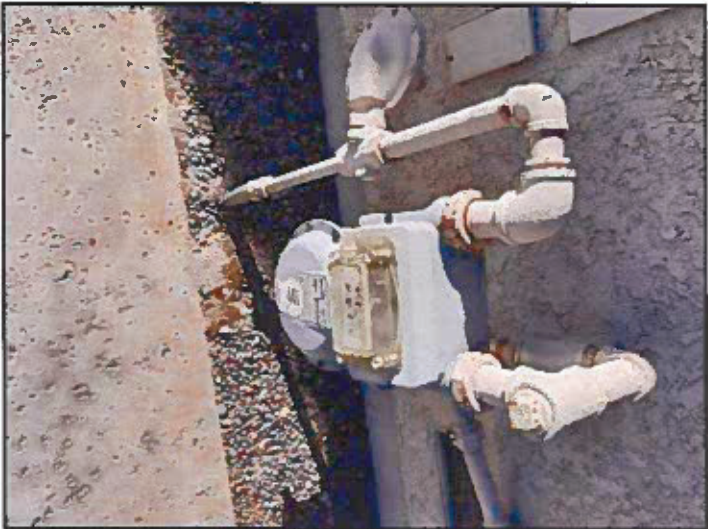
Missing earthquake wrench
