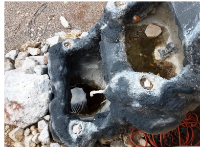
Additional Water Feature - Not Tested - No Water
