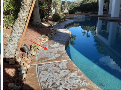
Hard Water Buildup
