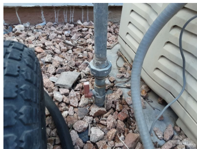
Gas Shutoff Valve
