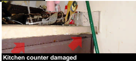
Kitchen counter damaged
