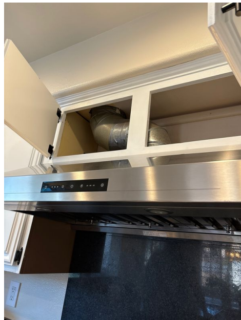
General: Exhaust / Ventilation Type Hood, Vented / Ducted
