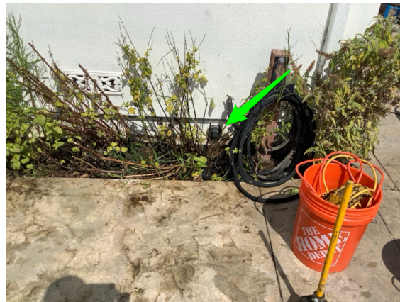
3" abs clean out at the rear of the property
