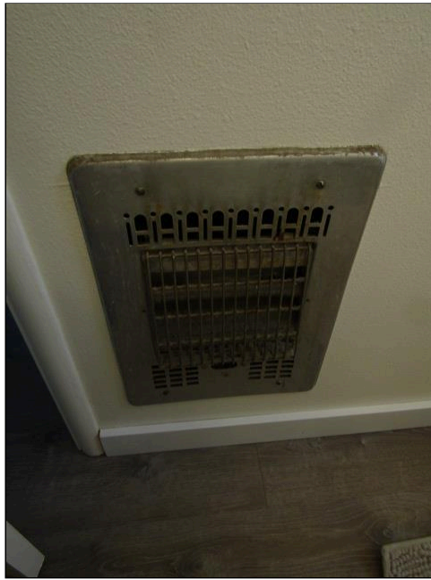
6.8.A HEATER UNIT Item 1(Picture)
