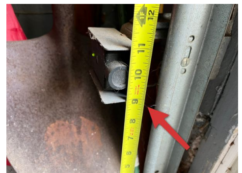
Example Noted at Garage
