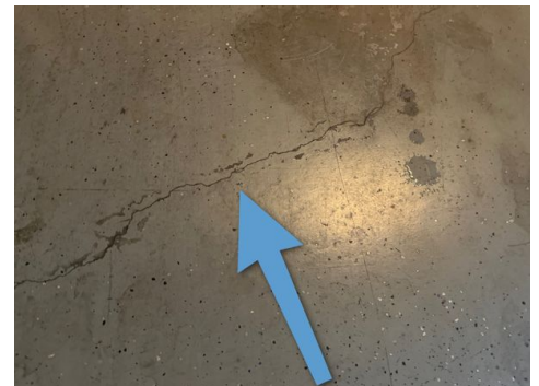
Example Noted at Garage
