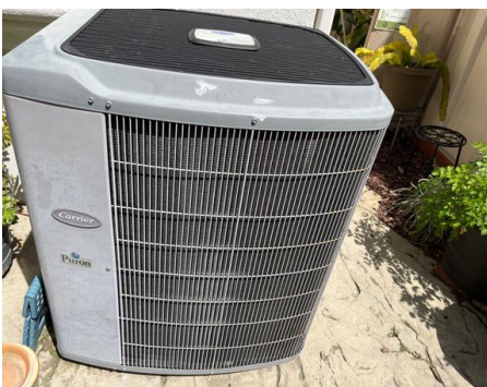
Example Noted at Condenser
