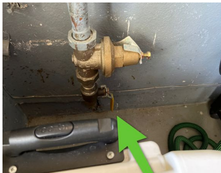
Example Noted at Garage
