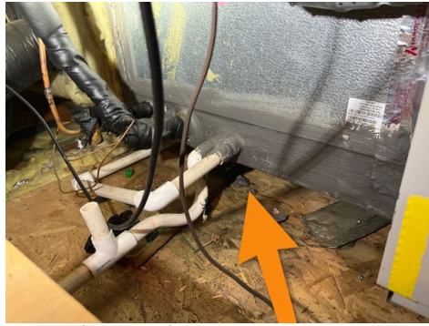
Example Noted at Heater
