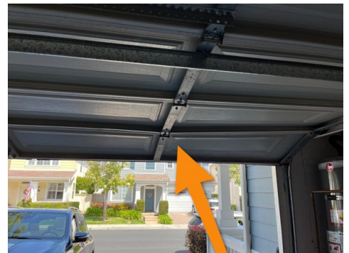
Example Noted at Garage
