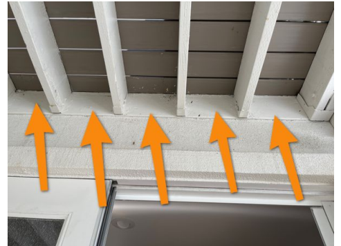
Example Noted at Rear
