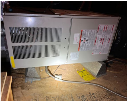
Example Noted at Heater
