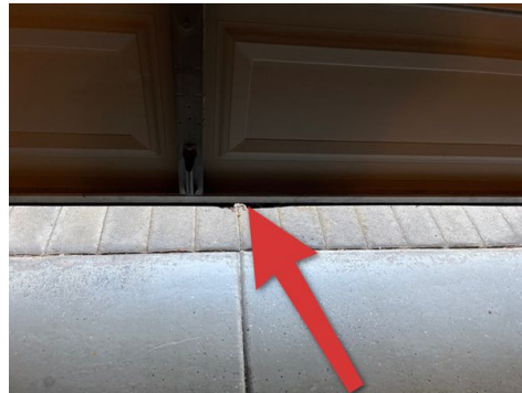
Example Noted at Garage
