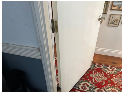
Example Noted at Garage
