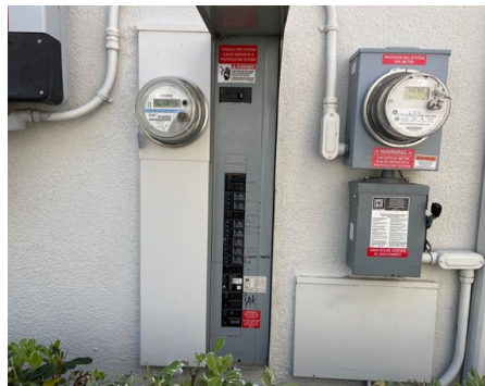
Example Noted at Main Panel
