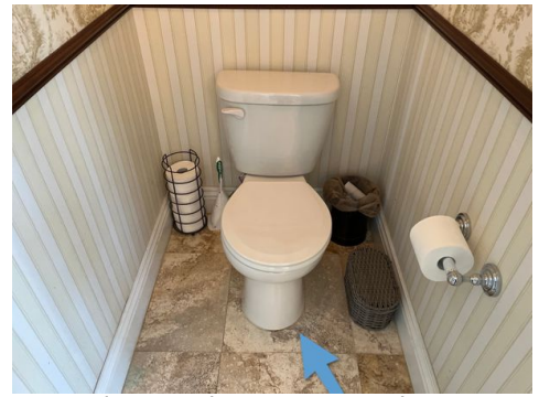
Example Noted at Master Bathroom
