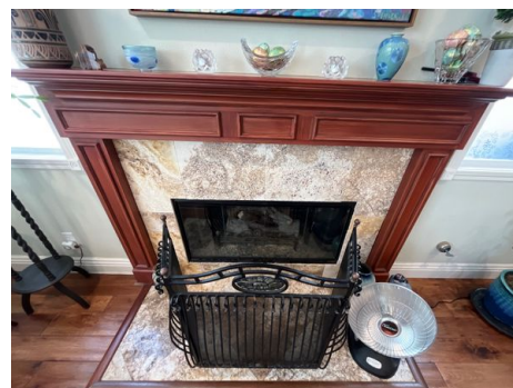
Example Noted at Fireplace
