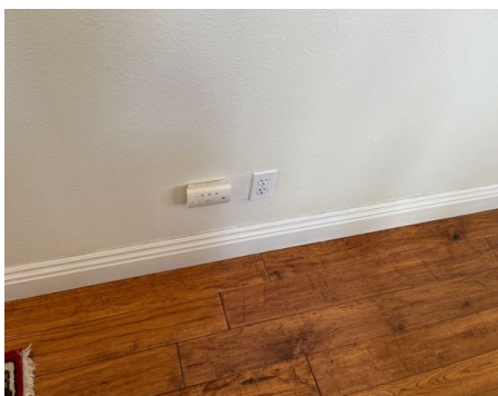
Example Noted at Hallway
