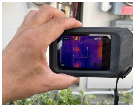
Example Noted at Main Panel
