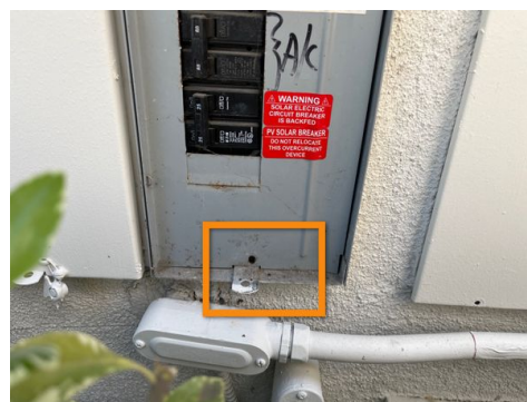
Example Noted at Main Panel
