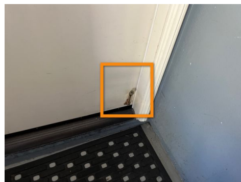
Example Noted at Garage
