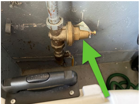
Example Noted at Garage
