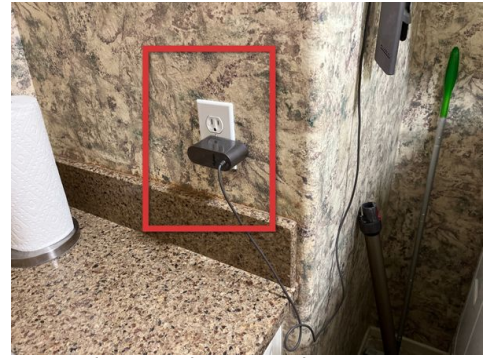
Example Noted at Laundry Room
