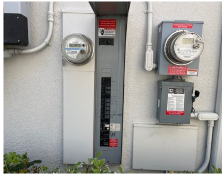
Example Noted at Main Panel
