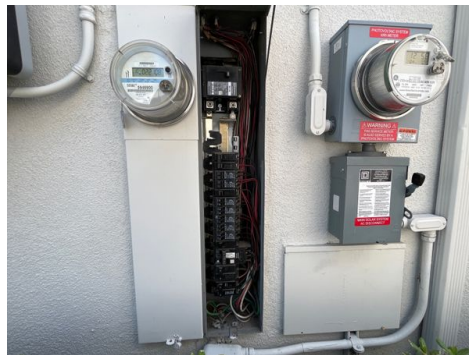
Example Noted at Main Panel
