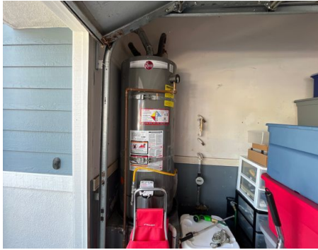
Example Noted at Water Heater
