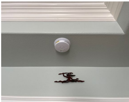
Example Noted at Master Bedroom
