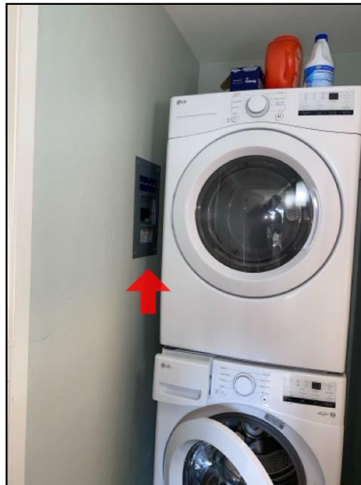
12. Inaccessible electrical subpanel
