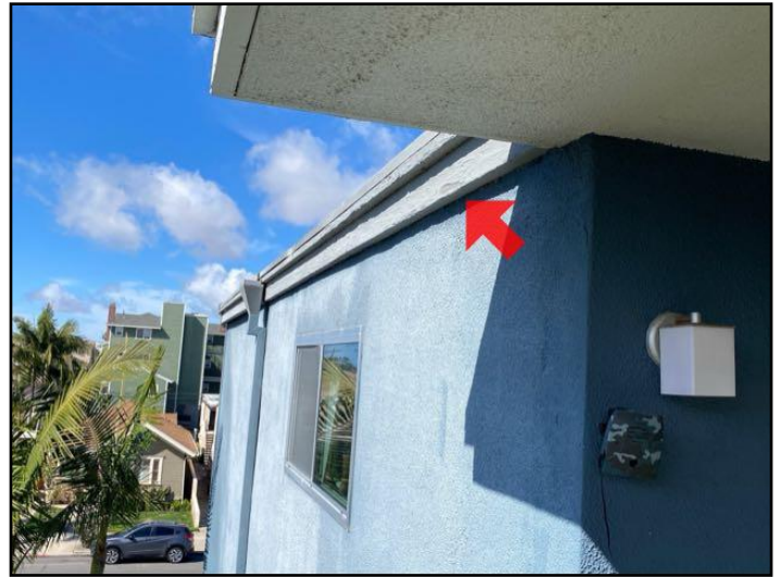
5. Paint improvement recommended
