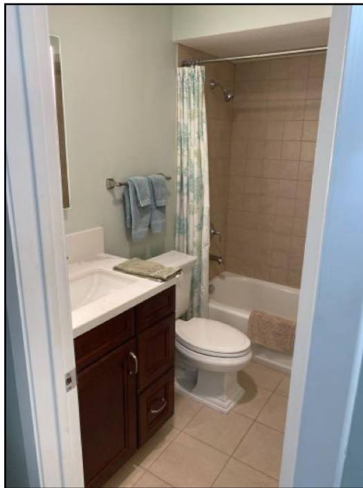
20. Below average water pressure/flow
