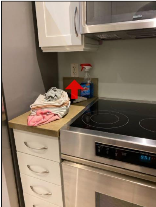
13. Damaged outlet (Kitchen)
