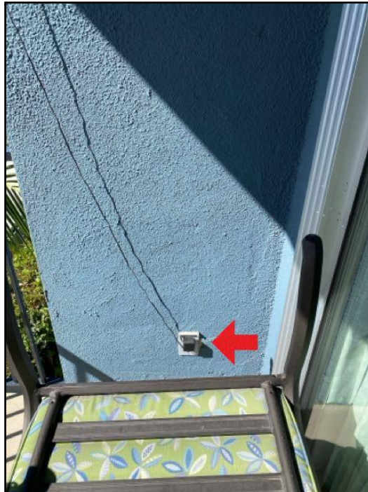
15. Missing exterior outlet weather cover
