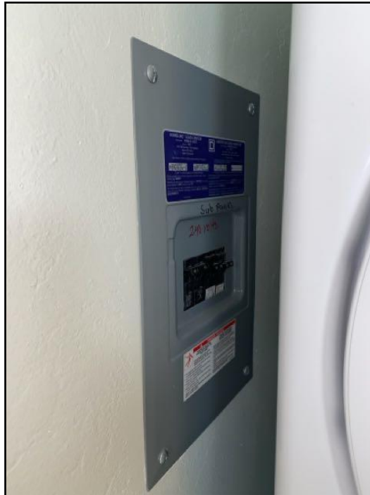
9. Breakers - Interior hallway
