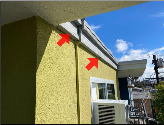
4. Paint improvement recommended
