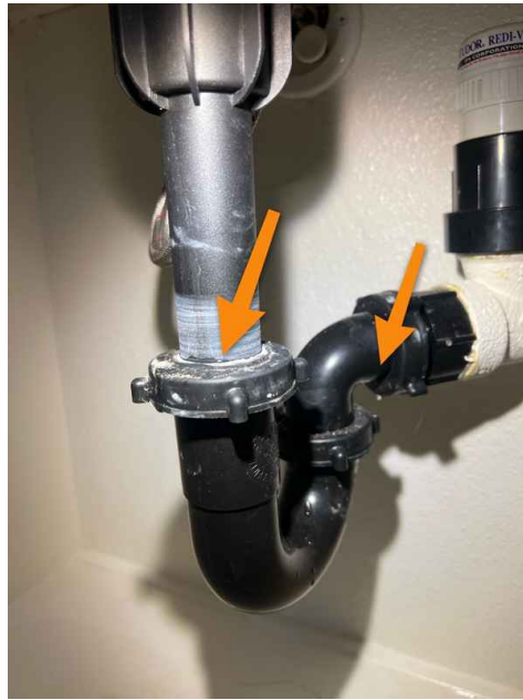
2nd Floor Hall Bath left sink
